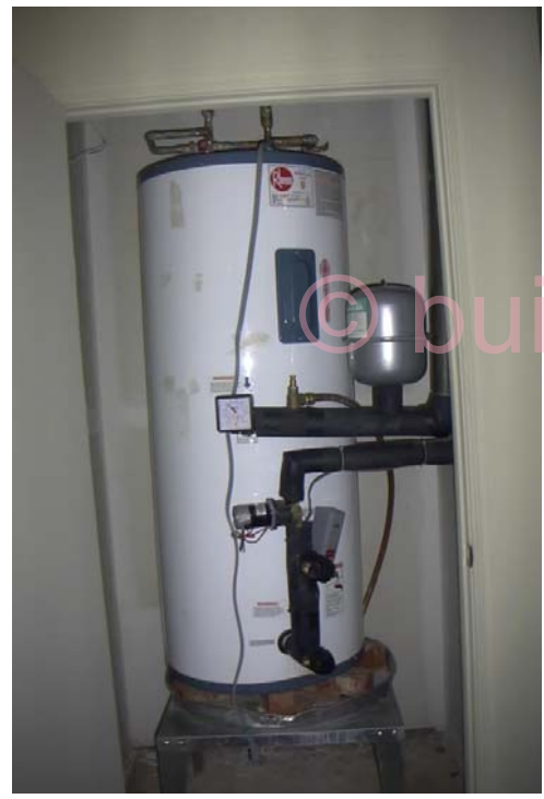
Tank and piping
