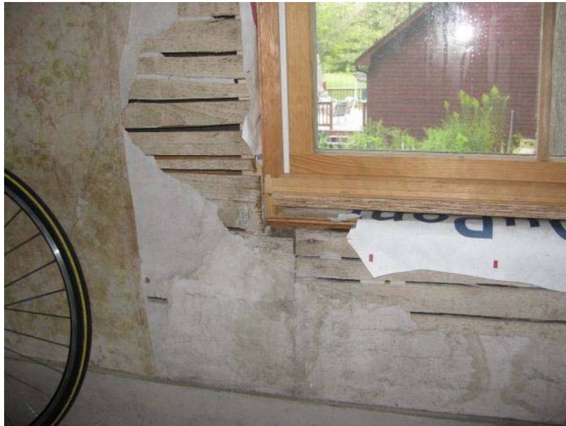
Existing replacement windows installed without flashing
