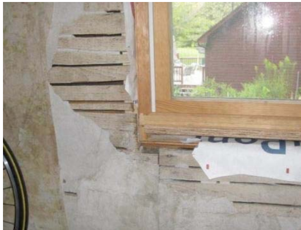
Existing replacement windows installed without flashing
