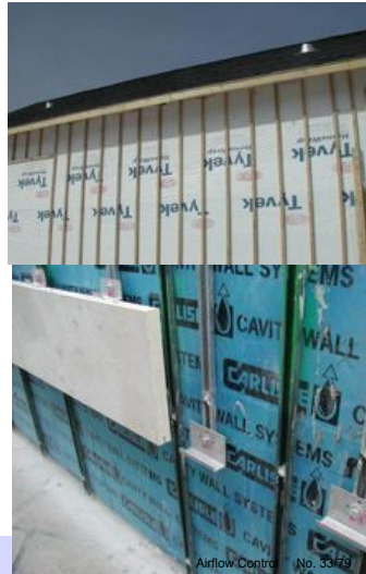
Airflow Control No. 33/19
