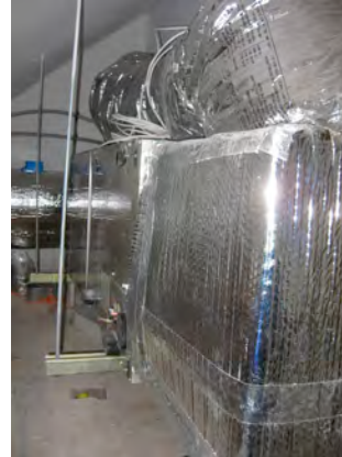
Air handler in conditioned attic
