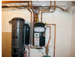
High efficiency boiler
