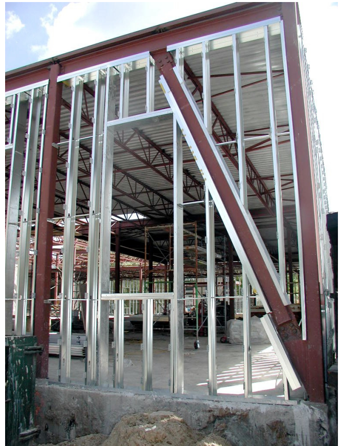
Photo 4: Conductive Heaven. Not much to say here except “what were you possibly thinking?” It is a waste to insulate the cavities. Exterior insulation is the only rational option here.
