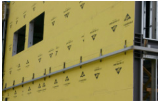
Photo 6a: Offset Relieving Angle. The angle iron support for the brick veneer is held away from the structural frame allowing exterior insulation to run by.
