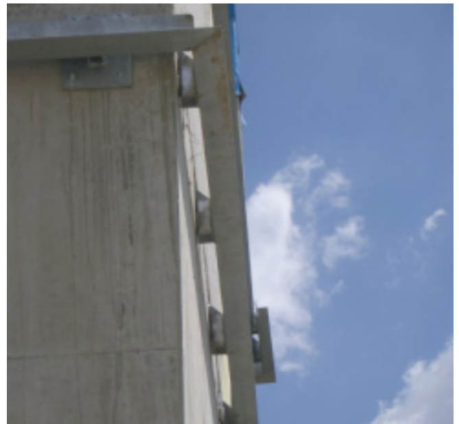
Photo 6b: Offset Relieving Angle. The angle iron support for the brick veneer is held away from the structural frame allowing exterior insulation to run by.
