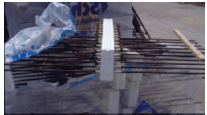
Photo 12: Structural Innovation. Thermal break at slab-balcony connection. Stainless steel rods are welded to reinforcing bars cast into the structural slab. The rods pass through a foam block that acts as a thermal break. The rods are staggered up and down to handle both compression and tension loads.
