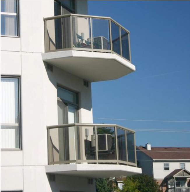
Photo 7: The Ultimate Thermal Bridge. A balcony is an efficient concrete-to-air heat exchanger that transfer every last available BTU across the structure.
