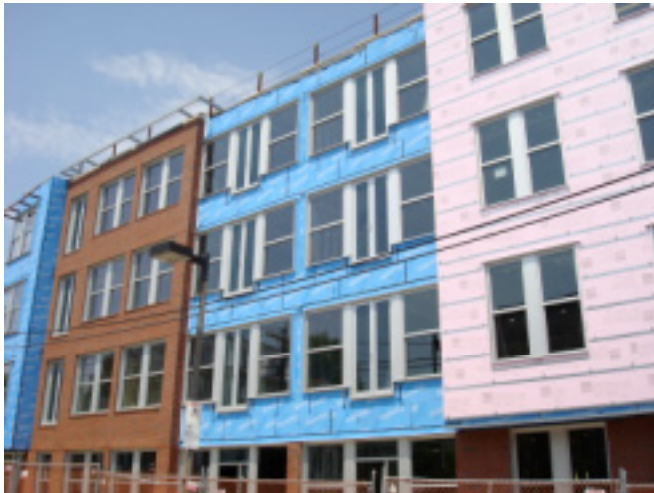
Photo 5: Exterior Insulation. The pink is the exterior insulation. The blue is the rain control layer (drainage plane) and the air control layer (air barrier) and the vapor control layer. The brown is the brick cladding.
