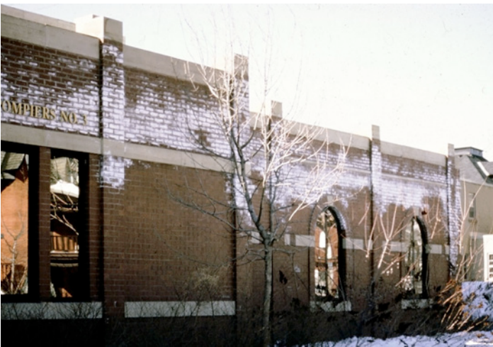
Photograph 2: Stack Effect Damage —This is stack effect air leakage leading to moisture induced damage for sure. Not rain. Why? Only happens in winter when it does not rain. Efflorescence. It came from inside and ate your building.... woo...scary stuff boys and girls...
