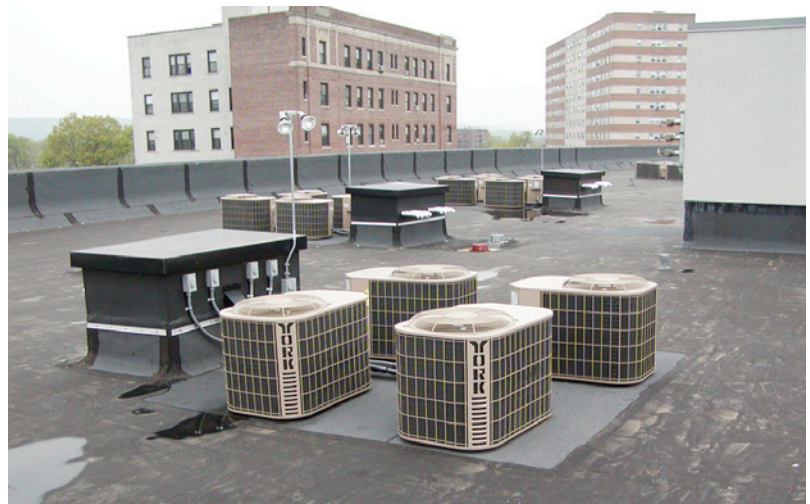
Photograph 3: Distributed Mechanical Systems —This is why the Gods of Building Science invented flat roofs: a place to stash mechanicals. Rooftop penetrations are collected and located in “doghouses”—all cable, duct and pipes are run through walls of “doghouses”.
