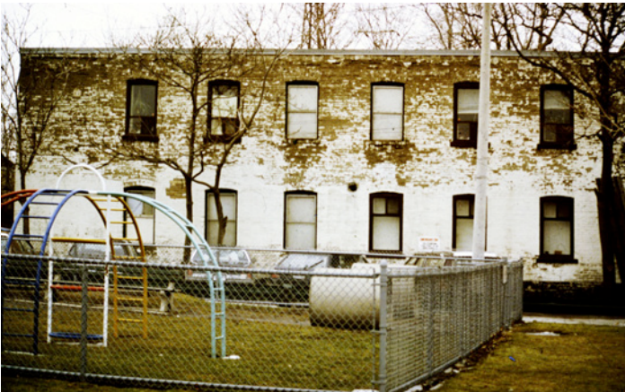
Photograph 1: Peeling Paint “Tell” - Where is the neutral pressure plane in this photograph? Neat eh? Air exfiltrating above the neutral pressure plane typically carries interior moisture. This moisture is deposited in the wall leading to peeling paint problems. Below the neutral pressure plane air is infiltrating from the exterior carrying little or no moisture. Legend has it that in this building an old oil boiler with a large active chimney was replaced with a sealed combustion condensing gas boiler lowering the neutral pressure plane. Of course, this picture could also be explained by rain deposition, but I am sticking with the air leakage neutral pressure plane story because it is so cool.
