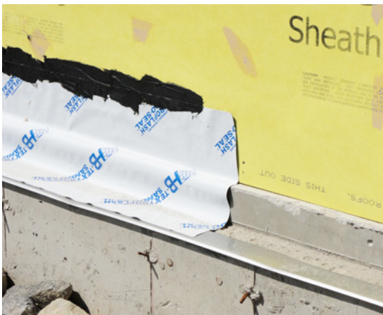
Photograph 7: Termination (left)– This “terminate” the reverse lap thing is a big deal. A continuous bead of sealant is used to glue the top edge of the reverse lap to the underlying membrane or sheathing.
