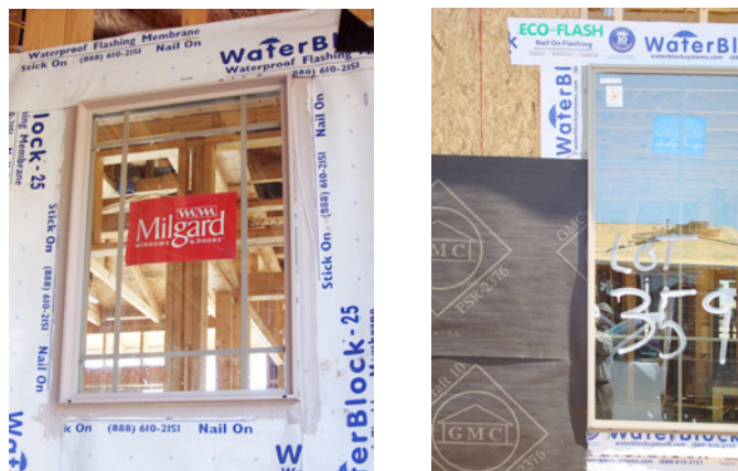
Photograph 1: Gravity Lap Part I (left)– The flashing strips are layered shingle fashion. Horizontal bottom sill first. Vertical side jambs next. Horizontal head flashing last. Note the sealant used to provide water control layer continuity between the window unit and the flashing strips. Photograph 2: Gravity Lap Part II (right)– The rolls of building paper are installed horizontally shingle fashion. The vertical edge of the building paper is sealed to the edge of the window unit with more sealant. Any water that enters at that joint is expected to be controlled by running down the vertical “side flashing” or jamb flashing and out at the bottom. The width of the jamb flashing is problematic. That is why the flashing tape and housewrap detail at the window jamb flange shown in Figure 2 (and in Sidebar I) is such an improvement.
