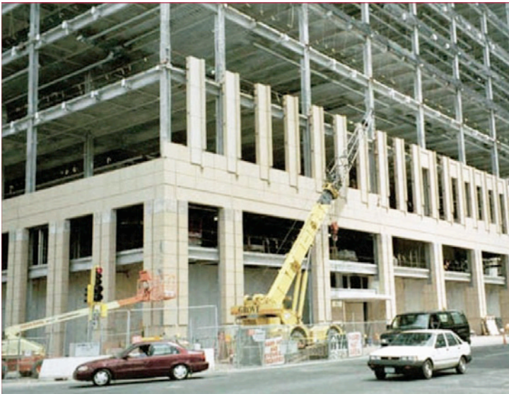
Photograph 1: Face-Sealed Panels —High risk in cold climates if air permeable insulation is used.
