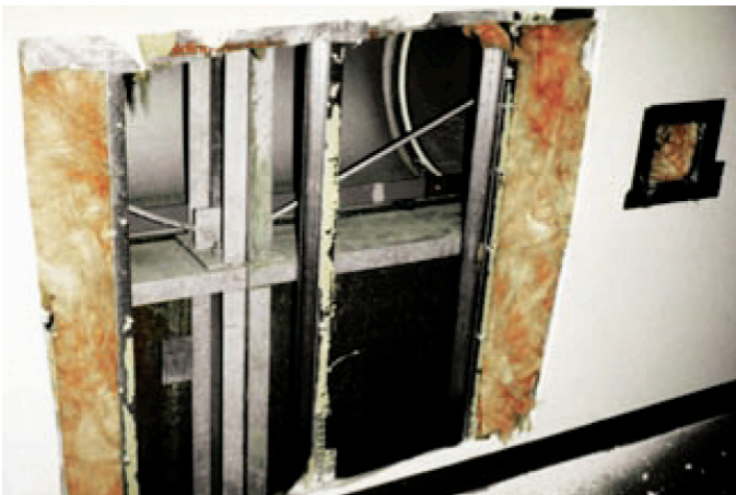
Photograph 4: Interior of Weeping Building —Typical steel studs, fiberglass batts, polyethylene vapor barrier and faith-based air sealing. No chance. This building was humidified. It “cried” as a result.
