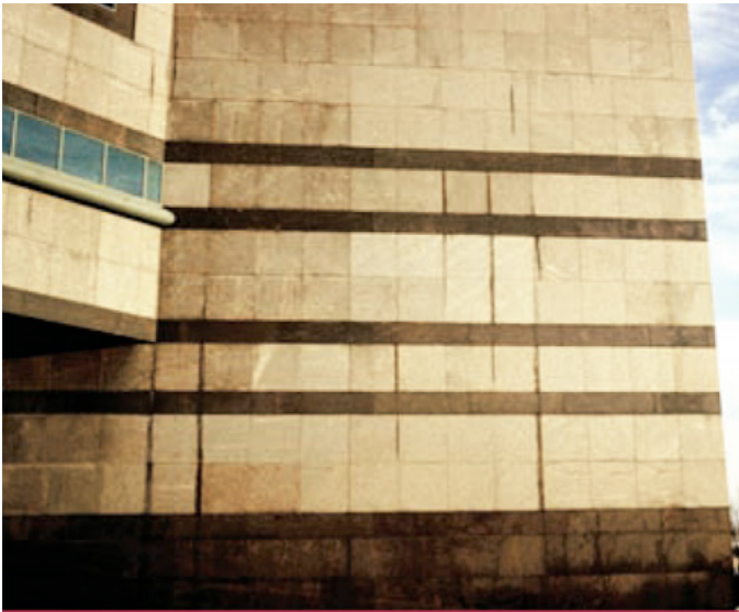
Photograph 3: Weeping Building —Face-sealed building where condensation is leaking out cladding joints.
