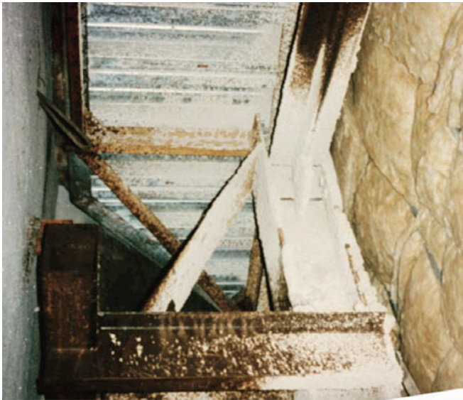
Photograph 5: Gift from the Engineering Gods—A continuous perimeter air gap between the precast panels and the interior insulated steel stud wall framing.
