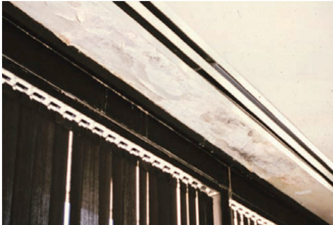
Photograph 4: Water damaged interior finishes at exterior walls.
