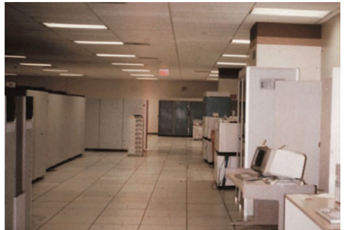
Photograph 2: Humidified and pressurized conditioned space.
