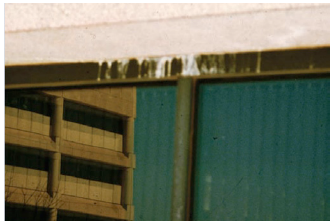
Photograph 3: Condensed water leaking out at window heads.
