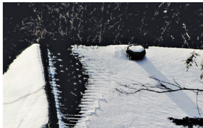
Photograph 7: Attic supply fan pressurizing roof cavity.
