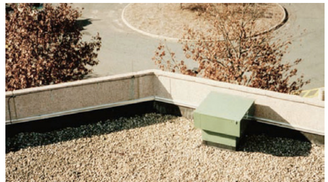
Photograph 6: Rooftop interstitial cavity pressurization system.
