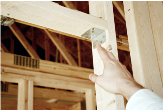
Photograph 5: Interior Wall Framing - Also framed on 24-inch centers. But these ones are 2x4's. And almost all of them are not load bearing so the connections are pretty much non-structural.
