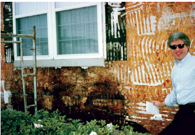
Photograph 4: Window Openings 1 —Leaking windows and OSB are a match made in consultant heaven. Notice the smile on the famous unidentified consultant. Of course the EIFS cladding had a little to do with this as well.
