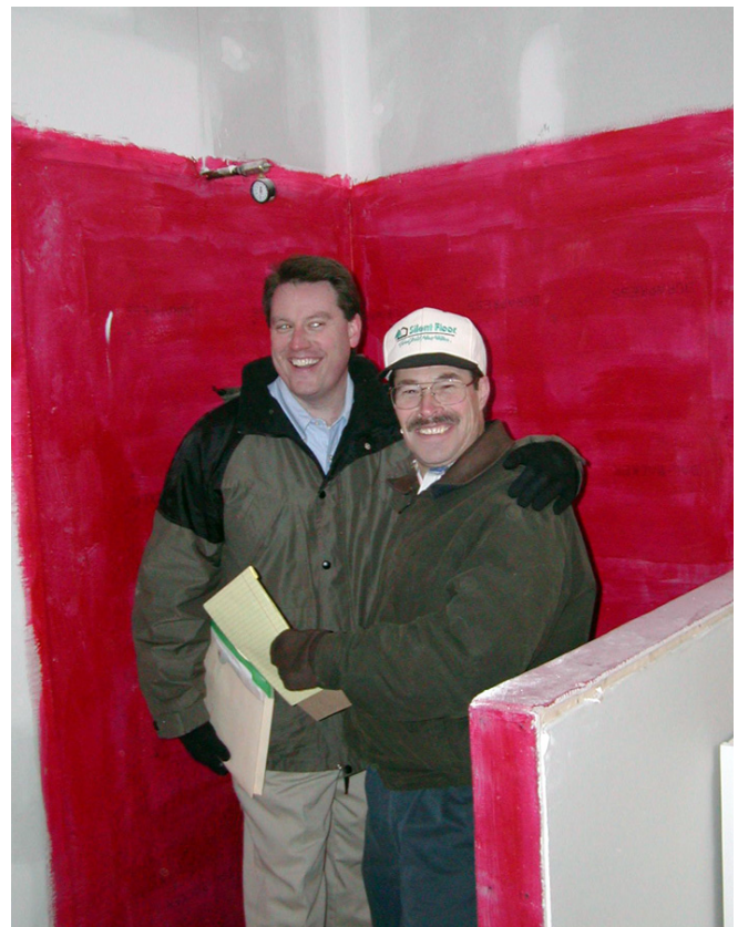
Photograph 7: Cement Board Shower Enclosure —A happy couple inside a cement board shower enclosure that has been coated with a liquid applied waterproofing prior to the application of tiles. They are happy as they are service and warranty personnel from a major production builder—they are celebrating the banishment of greenboard.
