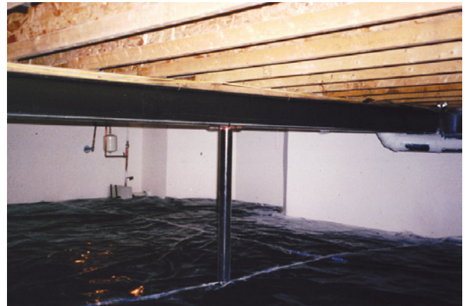
Photograph 6: Conditioned Crawlspace —Constructing crawlspaces like mini basements locates the engineered products within the interior environment.
