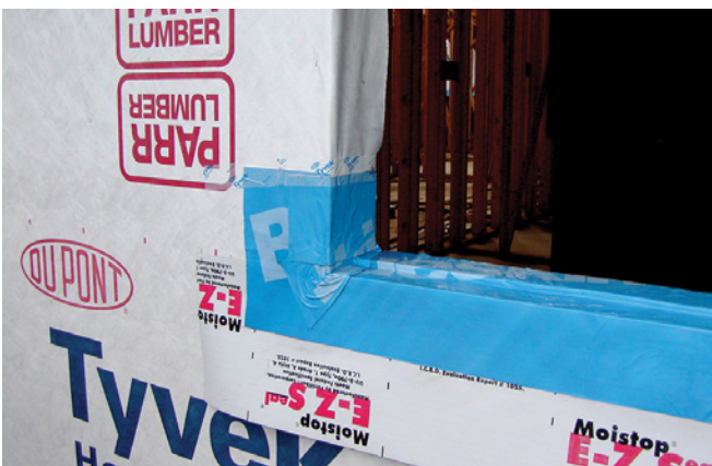
Photograph 5: Window Openings 2 —Notice the pan flashed opening. The products are discretely left unidentified as we don't actually want ASHRAE members to know what products actually work.
