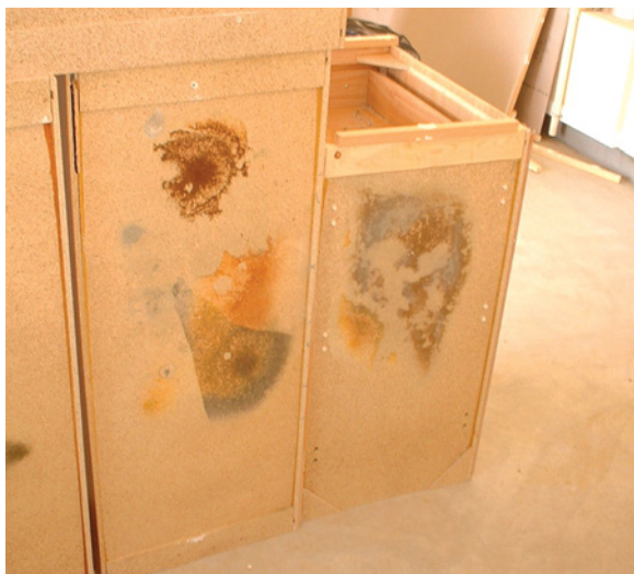
Photograph 2: Grass Cabinetry —Greenie weenie compressed grass laminate used in kitchen cabinets didn't fare very well in this "award winning" sustainable community. Solution? Get rid of the grass stuff? Nope. Back vent the cabinets.
