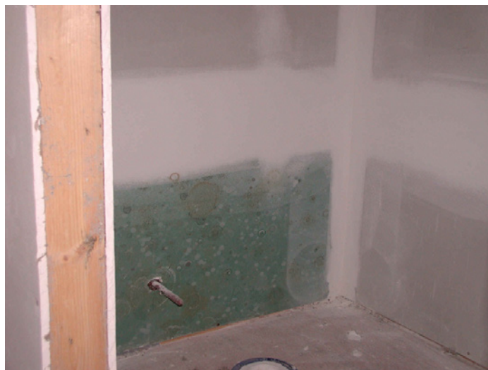
Photograph 3: Greenboard —It's not a good sign when the mold is already on the greenboard before the tiles are installed. What gives? The waxes added to protect the paper from liquid phase water—to meet a ridiculous ASTM spec—are "mold food." When products are optimized to meet arbitrary ASTM specifications rather than optimized to meet the "real world" problems result. Of course paper in a shower regardless of color is pretty dumb.
