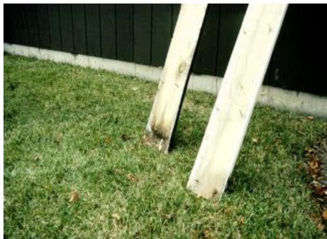
Photograph 6: Trim Issues - Trim elements tended to be the “weak link” as they tended to be adjacent to the most joints hence the most cut ends and exposed fibers. Where they butted into other elements or components or other trim pieces capillary absorption tended to be enhanced.
