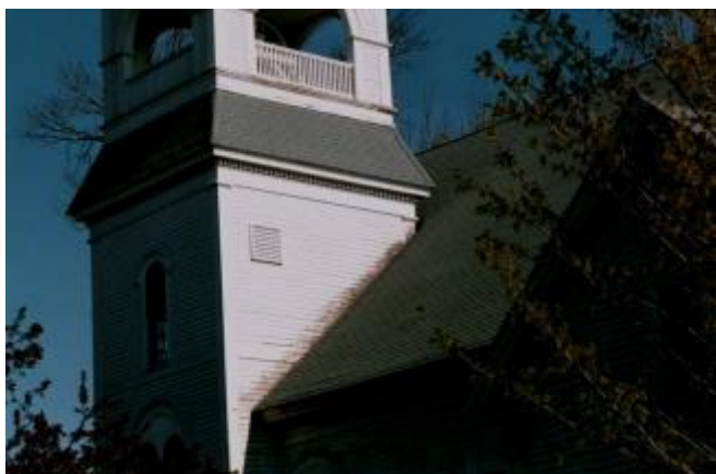
Photograph 5: Faith Based Water Control – Sloping end cuts not sealed where the cladding intersects the sloping roof.
