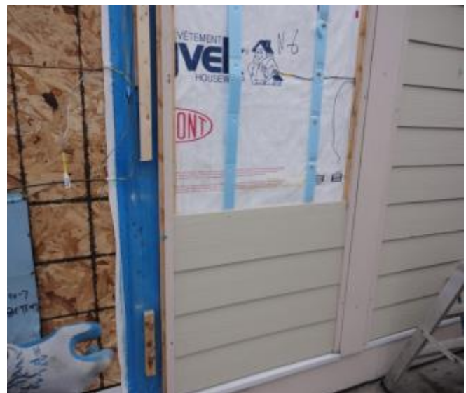
Photograph 9: More Test Hut Stress - Apparently, somewhere between 1/4 inch and 3/8 inch works well with wood and engineered wood based claddings and trim along with fiber cement cladding and trim components.
