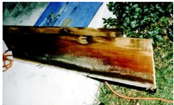
Photograph 3: More Capillary Wetting – This is more of a cold climate issue than a warm climate issue. Inward drive in warm climates increases the drying of the cladding. Of course this assumes that the inwardly driven moisture can go
