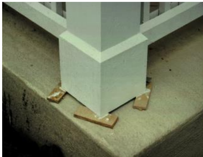
Photograph 7: Trim Gap - Sealing/painting cut ends, back coating and adding an air gap to act as a capillary break became necessary.
