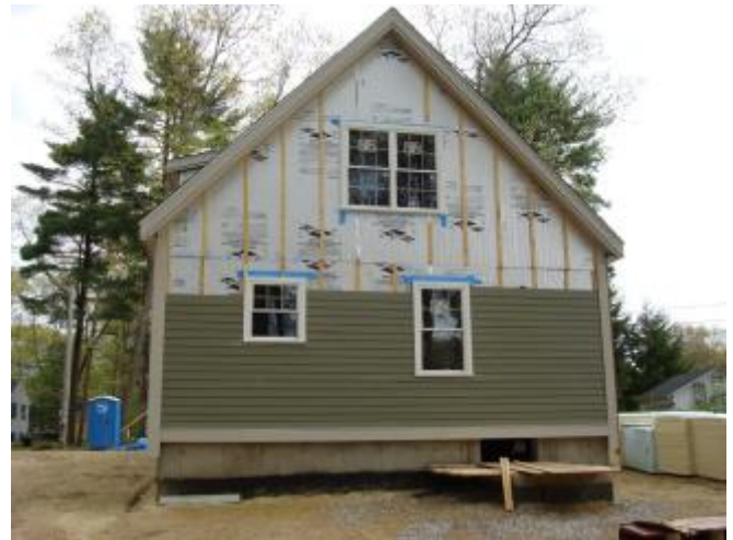
Photograph 12: Wood Furring - When you get to thicker layers of continuous insulation things get more complicated. You are pretty much limited to furring strips of 1x4 wood and long wood screws. Epoxy coated steel works well.
