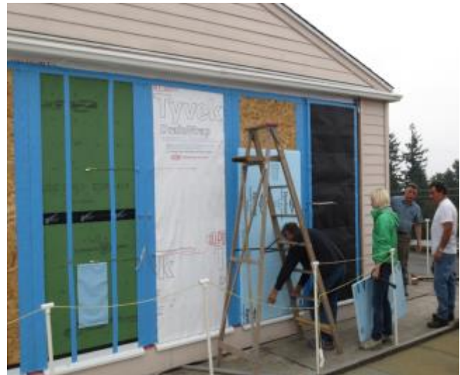
Photograph 8: Test Hut Stress – You can't calculate this. Being an old school engineer the approach to figure this out was obvious – guess – and test to failure.
