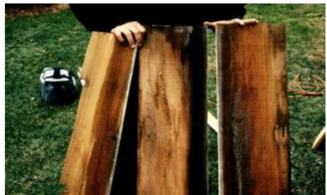
Photograph 2: Capillary Wetting - The effect of increasing the dwell time for moisture at the overlaps of siding. The “classic” means of addressing this issue is to reduce the capillary absorption at the overlaps and joints by “back priming” or “back coating” the back surfaces of the siding.
