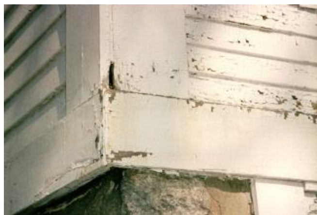
Photograph 1: Bad Paint - The paint looks bad, real bad, but there is no decay. This is an old uninsulated wood frame building. Board sheathing, asphalt impregnated felt building paper. Wood clapboard siding and wood trim. Oil based primer and oil based paint. Water is getting behind the wood siding and trim via capillarity. The water can't evaporate outward through the impermeable paint film.
