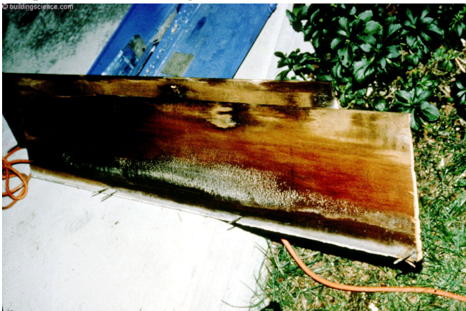
Photograph 4: Rotting moldy siding -thank you CHIP
