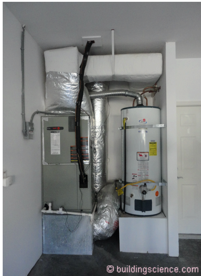
Photograph 8: Mechanical air distribution systems (forced air furnaces/AC units) and associated ductwork should not be installed in attached garages due to the potential risk for air leakage of such systems drawing air from garages into occupied unit spaces
