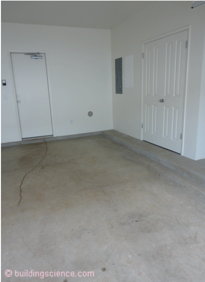
Photograph 9: Mechanical systems should be located within "air-sealed" rooms that are connected to the occupied space. Note the automatic door closer for the door to the occupied unit. Airtight door sweeps and weatherstripping are necessary.
