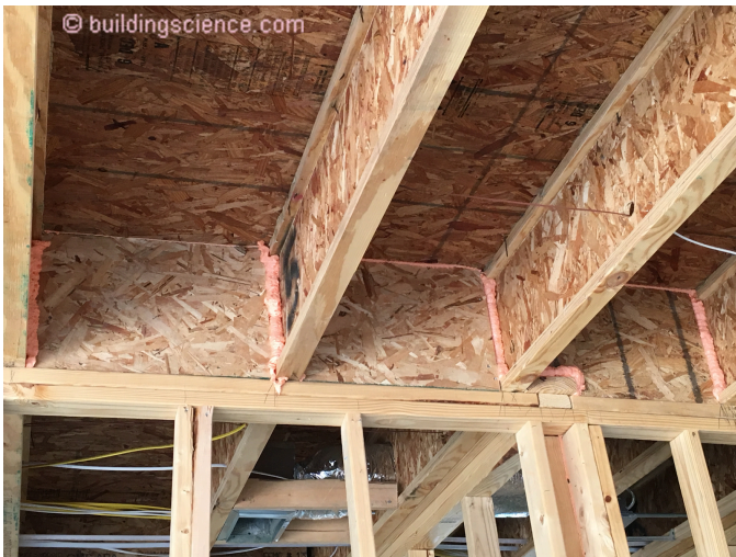
Photograph 3: OSB blocking that is notched and sealed around wood I-joint floor framing.
