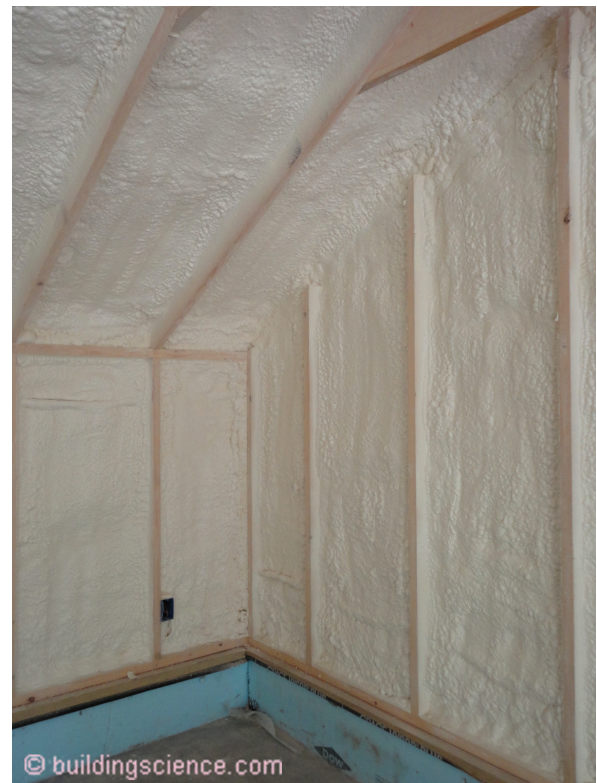
Photograph 7: Spray foam cavity insulation on the walls separating the garage from the exterior. Again, note that the wall assembly will need to meet the applicable fire rating requirements.
