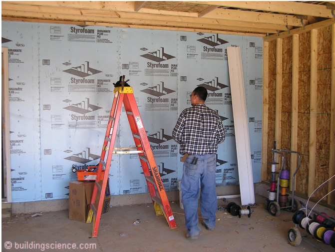
Photograph 2: Rigid insulating sheathing installed on the wall separating the house from the garage. Note that the rigid insulation assembly will need to meet applicable fire rating requirements
