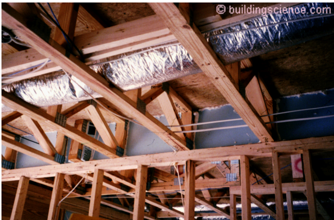
Photograph 4: Gypsum board blocking used with a floor truss assembly. Note the location of a vertical member within the floor truss
