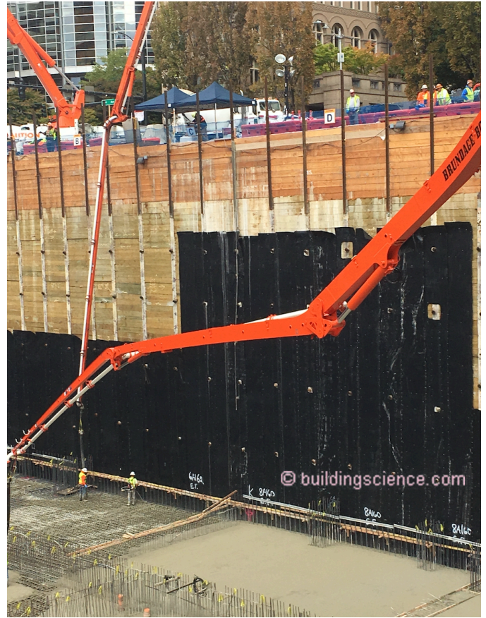
Photograph 5: Waterproofing membrane on the interior of a deep soldier pile foundation with wood lagging.
