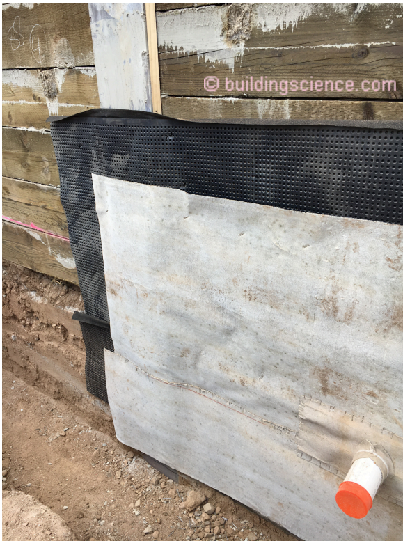
Photograph 4: Note the well-sealed service penetration in the waterproofing membrane, drainage mat and protection layer on the interior of soldier piles and wood lagging.
