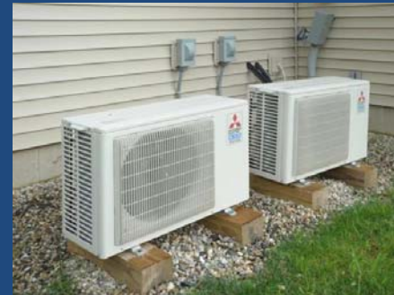
Mitsubishi Outside Units
