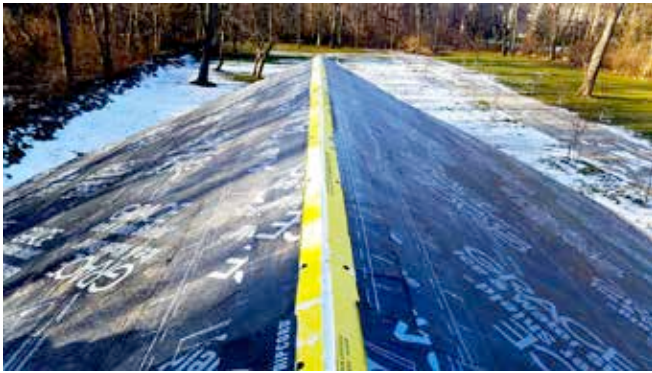
Photograph 4: Vapor Diffusion Port Under Construction —Note the glass fiber-faced gypsum board strip on either side of the ridge. This material acts as a water vapor control layer and air control layer while providing high water vapor transmission. It also provides fire resistance. Note the snow on the ground. This is not New Orleans or Galveston – it is my backyard.
