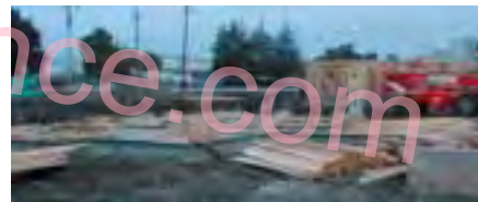
Figure 8a This is not the way to store materials on the job site.
