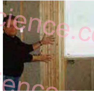
Figure 2 Where one stud is good, two must be better, and 9 must be the ultimate. This is MVE — minimal value engineering.
