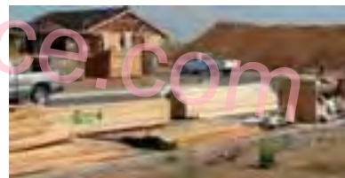
Figure 8b This is the way to store materials on the job site.
