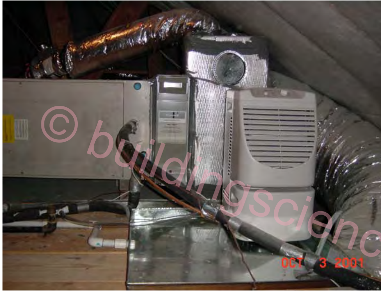
Figure A-2a. Stand-alone dehumidifier in conditioned attic
