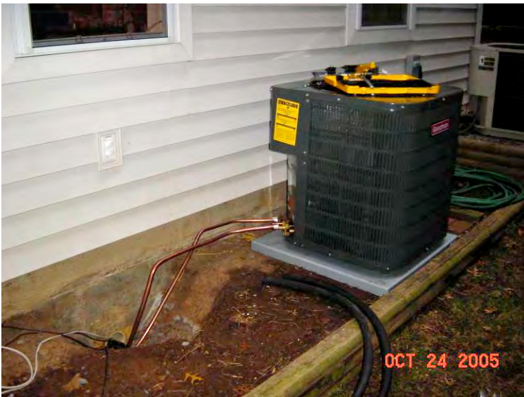
Figure 8: Outdoor unit with scroll compressor and accumulator being fitted for refrigerant piping
