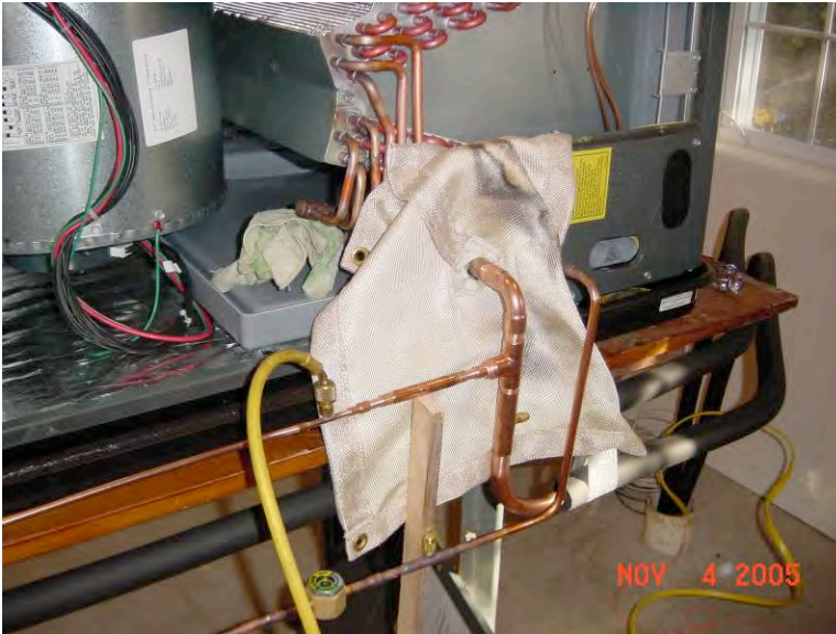
Figure 11: Connections brazed at indoor unit with nitrogen flowing internally; heat sensitive components protected with blaze cloth and wet rags
