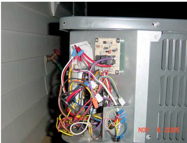
Figure 17: 24 Vac relay added to outdoor unit to allow on/off control of condenser fan
