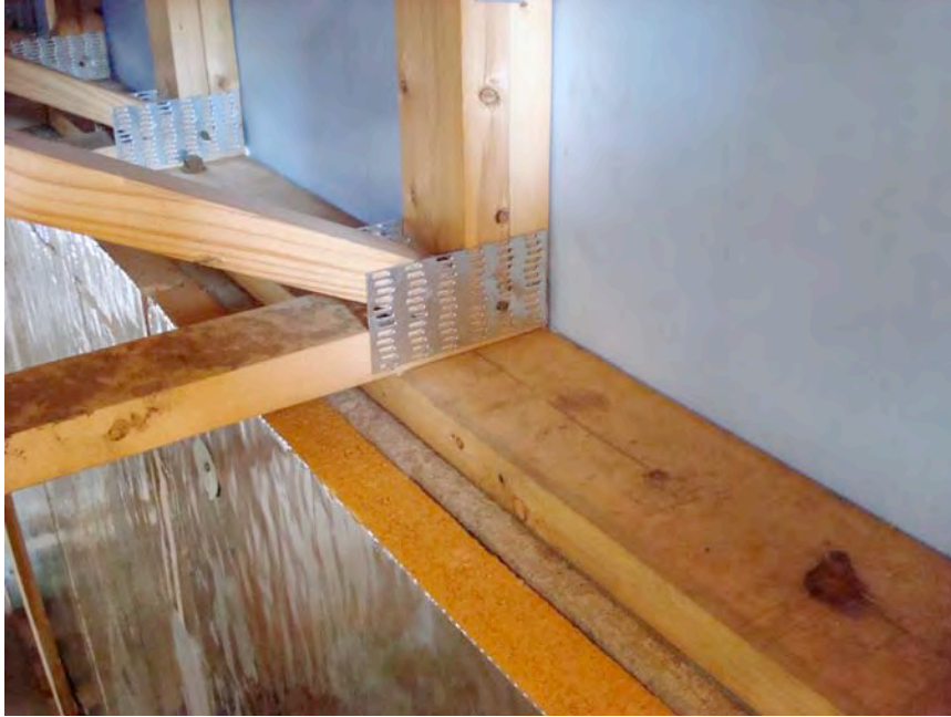
Figure 4.3: Photograph of floor system at top of foundation wall - this area to receive spray foam air seal.
