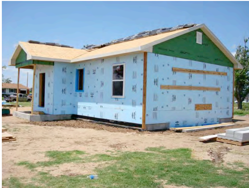
Figure 4.11: Photograph of house exterior with insulating sheathing and windows partially installed. Pan flashing visible where window has not been installed on front of house.
