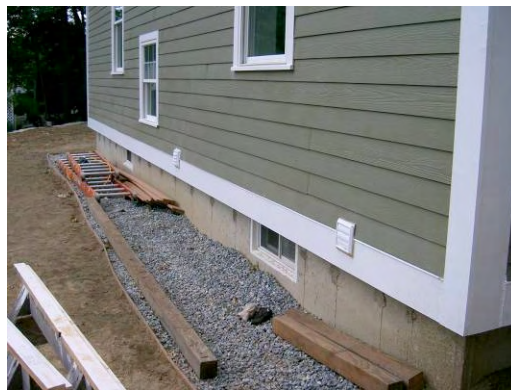
Figure 1.37: ERV intake and exhaust
