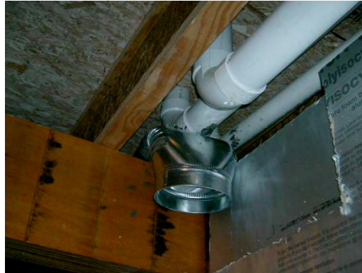
Figure 1.36: Plumbing, ductwork and foam in joist bay
