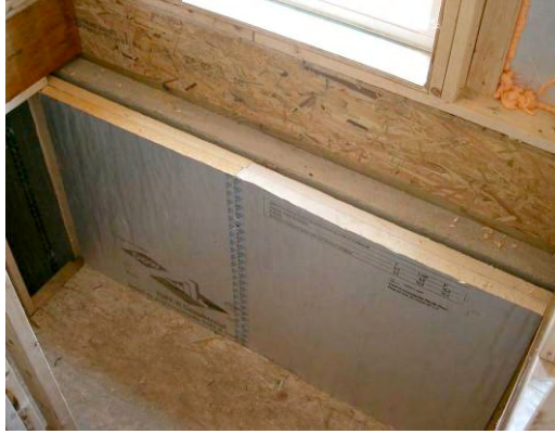
Figure 1.24: Basement foam at stairwell (pre air sealing)
