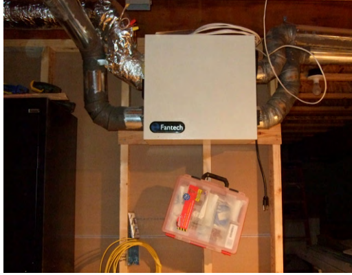
Figure 1.11: Installed energy recovery ventilator
