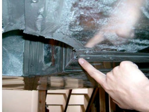
Figure 1.44: Air leakage location in sheet metal duct
