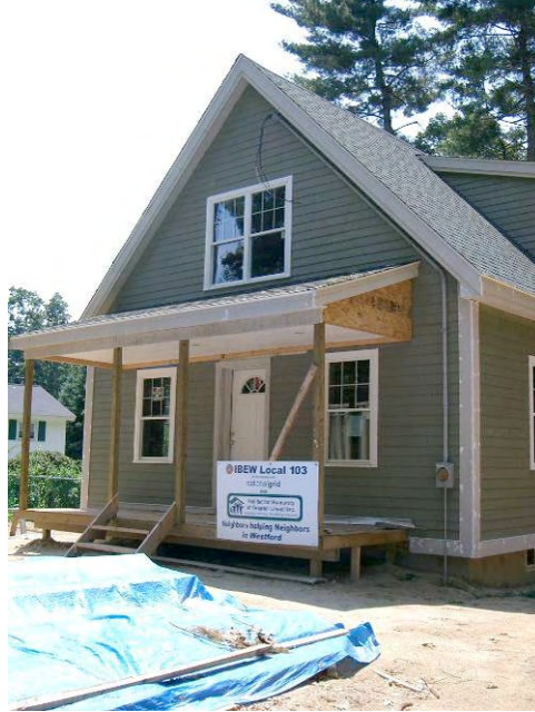
Figure 1.42: Electrical service on front of house
