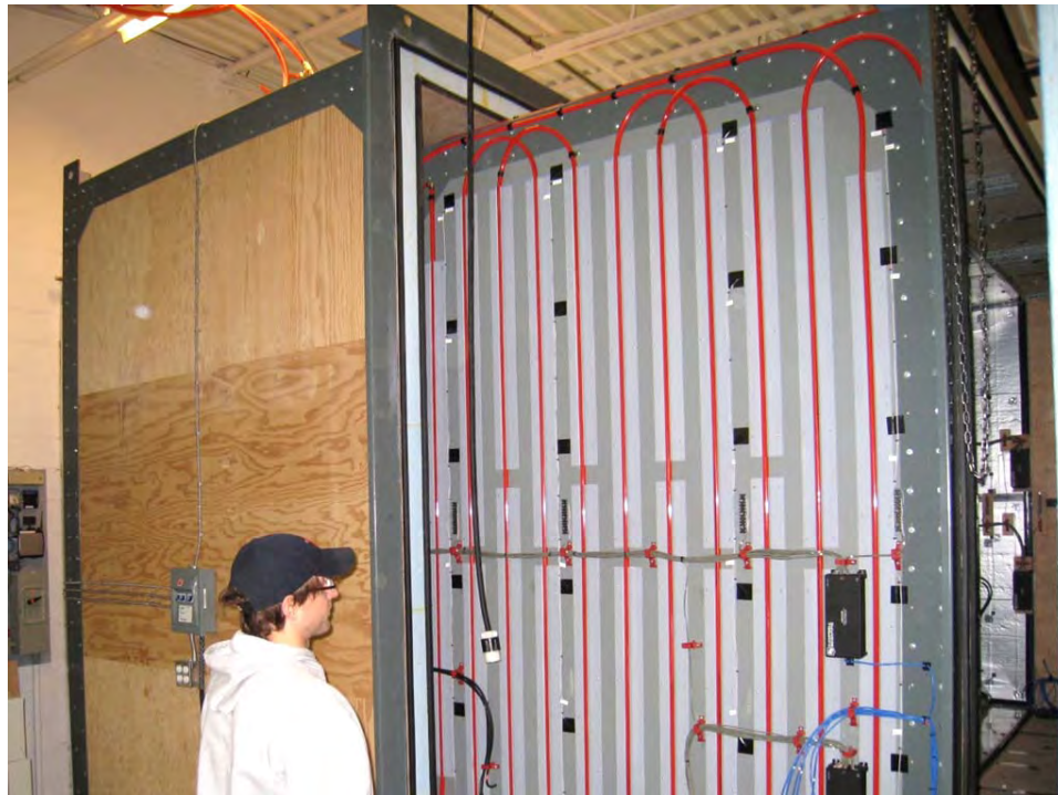
Figure 4 - Double Guard: Guard Box (Left) and Liquid Guard Loop on Meter Box (Right)
