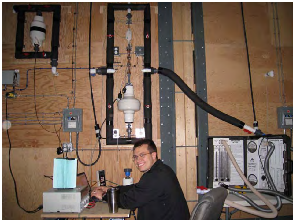
Figure 29 – Air Transfer System Commissioning
