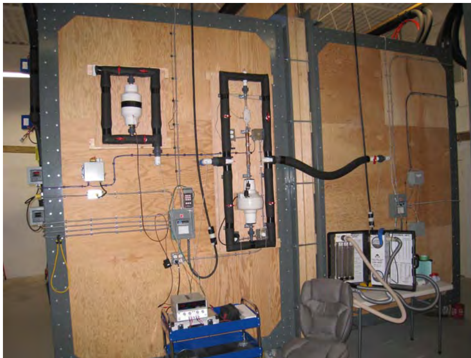
Figure 8 – Guard Fan (Left) & Air Transfer System (Center)
