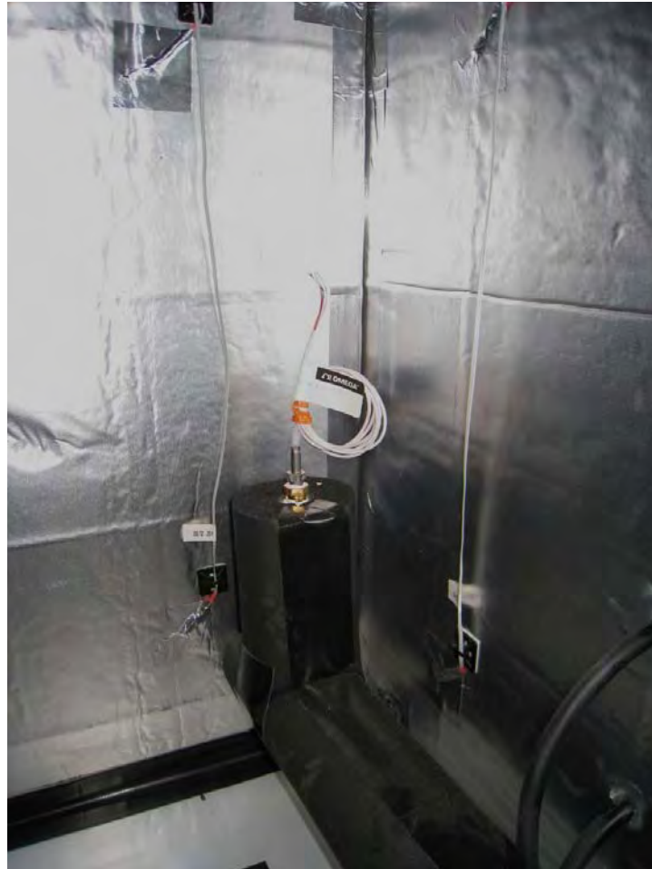
Figure 26 – Insulation around Meter Box Cooling Water Return Temperature Measurement
