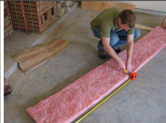
Cut R-13 fiberglass batt to appropriate length (4' for 8" ducts, 3' for 6" ducts, 2' for 4" ducts).
