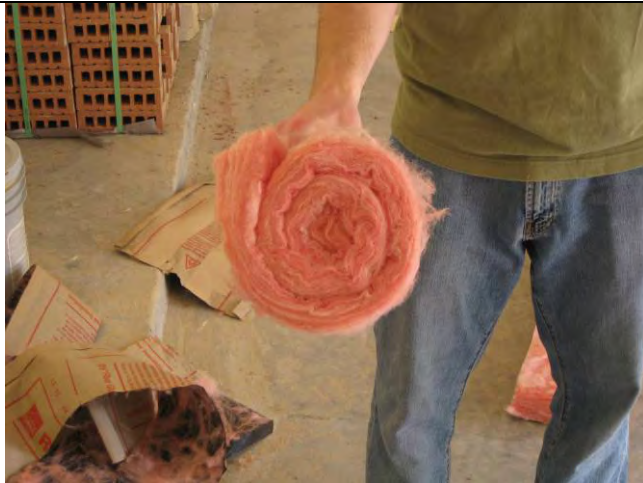
Peel off kraft facing and roll into cylinder.
