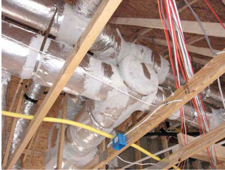
Figure 3.3.8: R-6 Insulated Ducting in Attic Space
