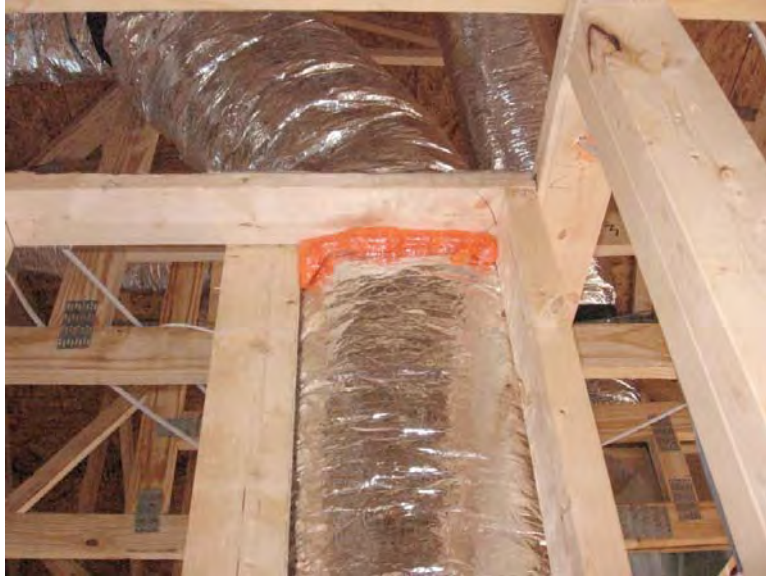
Figure 3.3.4: R-6 Insulated Ducting Entering from Attic Space
