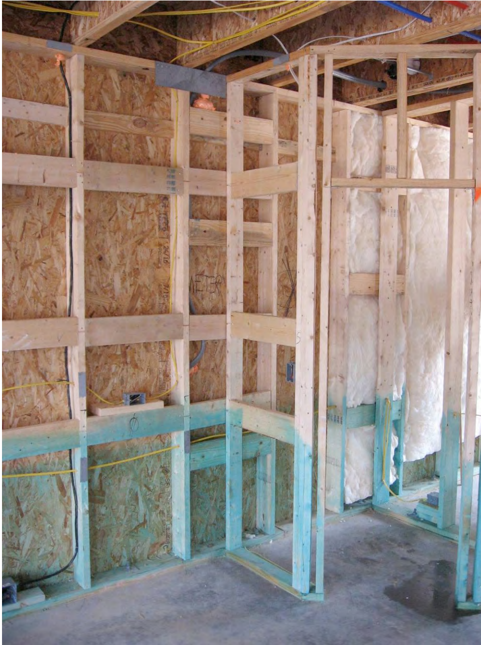
Stack Framing at 24" OC, Single top and Bottom Plates and blocking for Cabinetry
