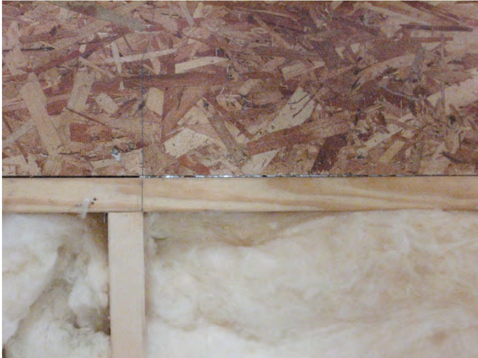
Example of Air Leak Requiring Sealing – Note visible light above top plate and below header – Repaired on while on site.
