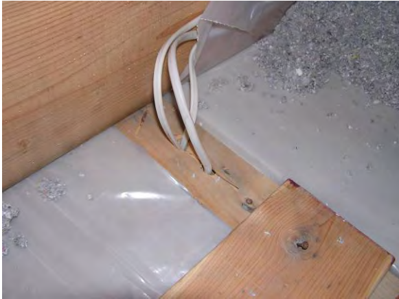
Figure 11: Un-sealed wire penetrations
