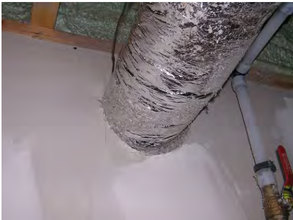
Figure 5: Leakage around exterior outdoor air intake duct
