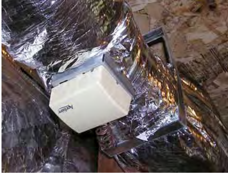
Figure 1.3.11: Aprilaire motorized damper installed on outdoor air intake duct
