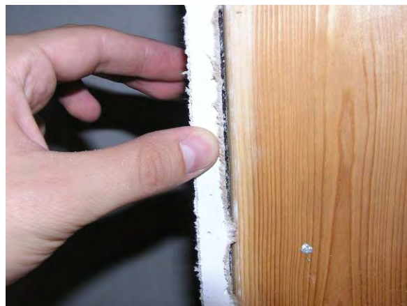
Figure 18: No caulk visible around window openings
