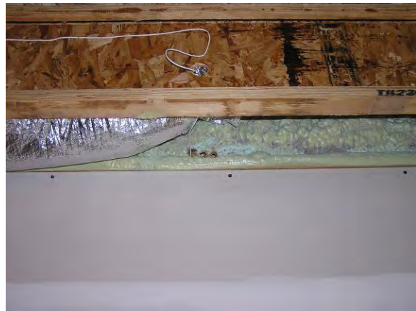
Figure 6: Leakage at small holes drilled through exterior foam seal
