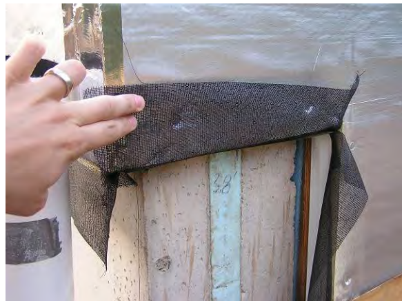
Figure 22: Insect screen installed to wrap the exposed edge of the foam sheathing
