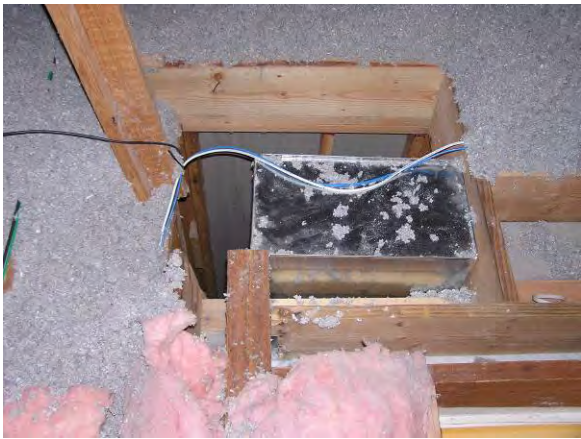
Figure 7: Open hole at top of duct chase
