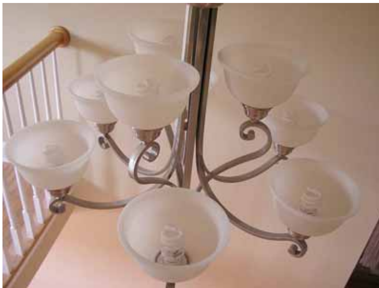
Figure 1.3.12: Compact fluorescent lamps installed in the lighting fixture
