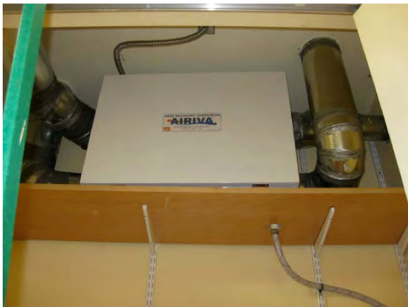
Figure 10.3.14: Heat recovery ventilator installed in second floor closet
