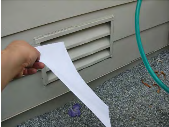
Figure 6: Outside economizer damper; HVAC system running
