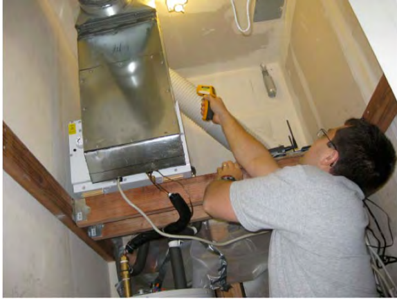
Figure 10.3.10: Ductwork attached to AirTap air source heat pump water heater
