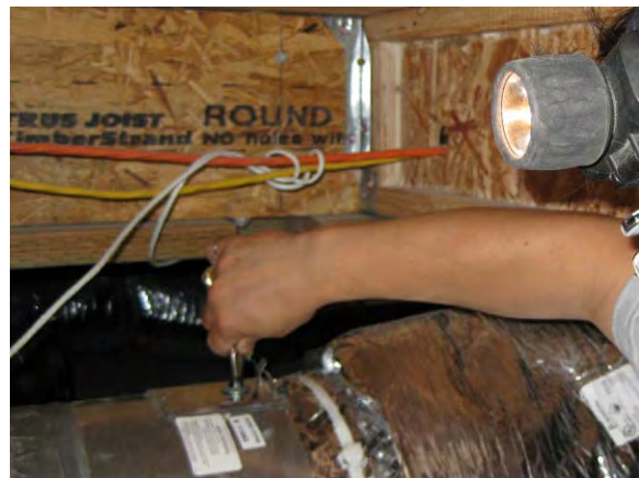
Figure 5: Manually tightening damper seal
