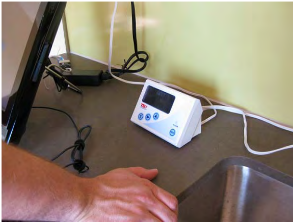
Figure 20: TED installed on kitchen counter
