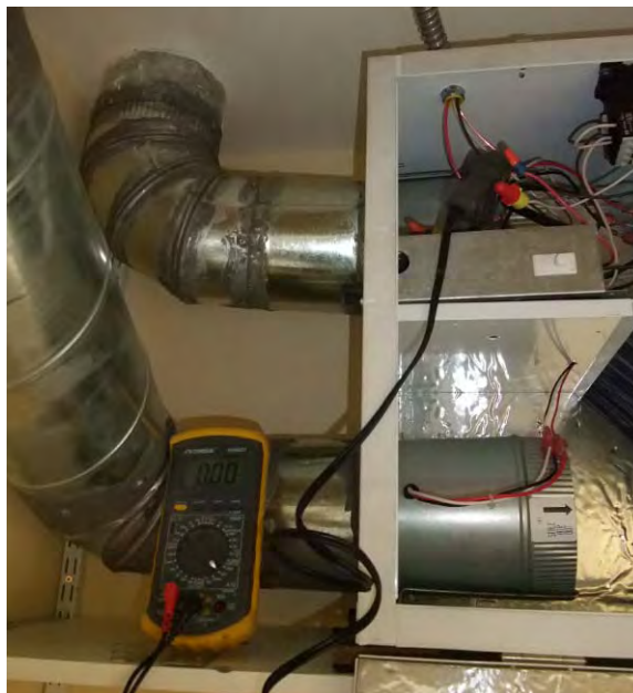
Figure 22: Power measurement of HRV using amp clamp (HRV door closed during test)
