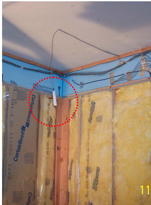
Figure 4: T/RH sensor protected by pipe segment (indoor application shown; will be used for outdoor sensor)
