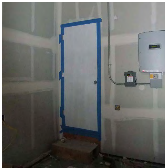
Figure 4: Mechanical room door sealed
