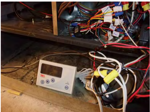
Figure 38: Air handler monitoring installation (TED & switching relays for runtime)
