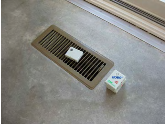
Figure 10: Use of data loggers to collect delivered register air temperature
