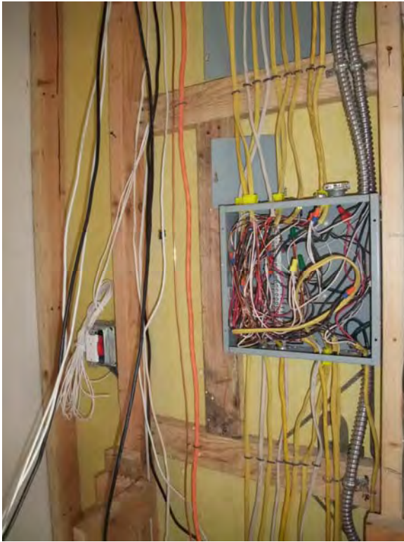
Figure 24: Wall between mechanical room and bathroom, showing electrical panel and wires
