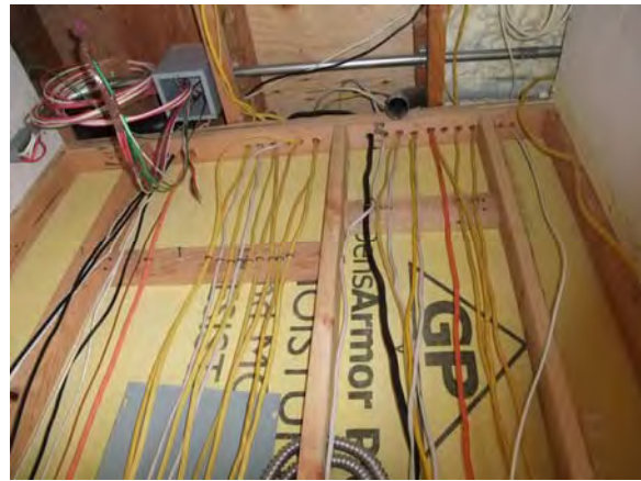
Figure 26: Mechanical room-bathroom wall, showing electrical penetrations
