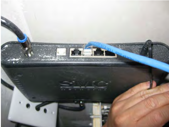
Figure 17: Router, showing open ports
