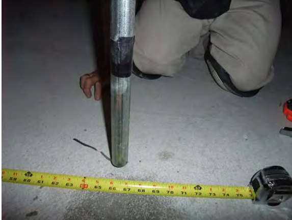
Figure 8: Concrete basement slab surface T (front of basement)
