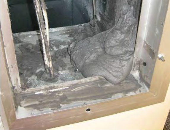
Figure 3: Slumped mastic at upstairs return
