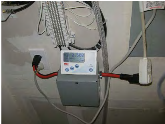
Figure 23: TED for heat pump water heater logging
