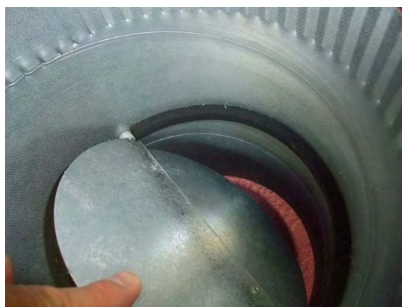
Figure 15: Close up of motorized damper gasket seal as example
