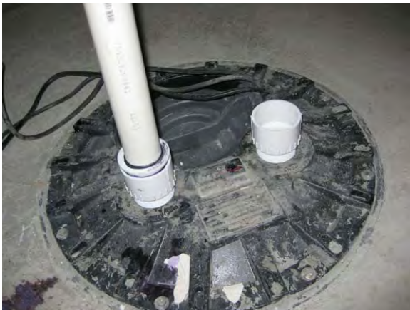
Figure 19: Sump pit cover
