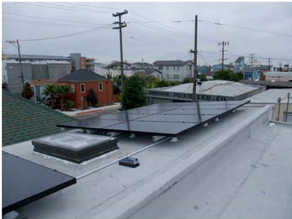
Figure 10.3.25: 5.4 kW PV array mounted on roof, surrounding skylight
