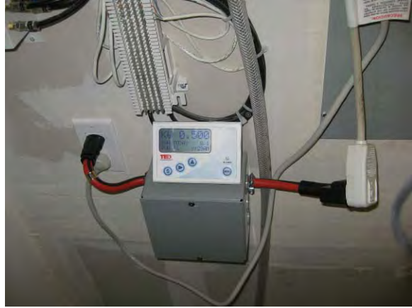
Figure 9: Measurement of AirTap power use
