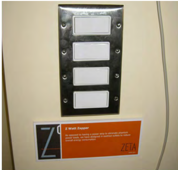
Figure 10.3.19: Plug load control with “z Watt Zapper” switched receptacles
