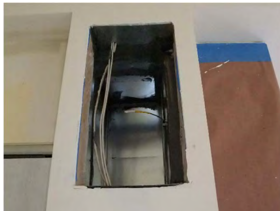
Figure 10.4.14: T/RH sensor installed in second floor return duct
