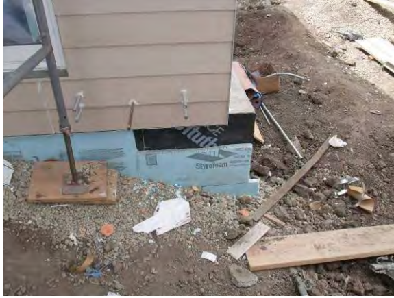
Figure 10.3.5: Exterior view of conditioned crawl space, showing 1.5" R-7.5 XPS
