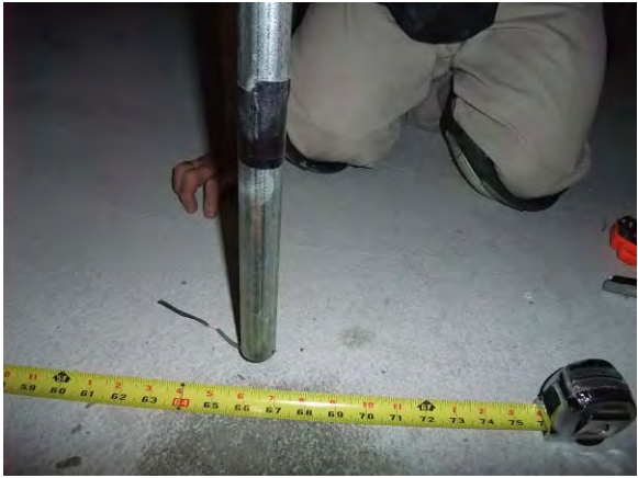
Figure 34: Concrete slab surface T (front of basement); pipe provides physical protection
