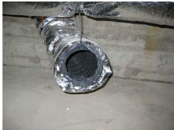
Figure 10.4.8: Data logger placed in open duct in basement ('Bsmt Duct')
