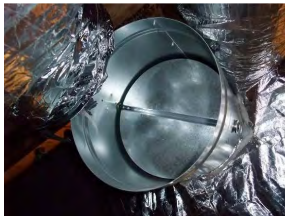
Figure 10.5.4: Motorized damper, showing lack of gasket or sealing measures
