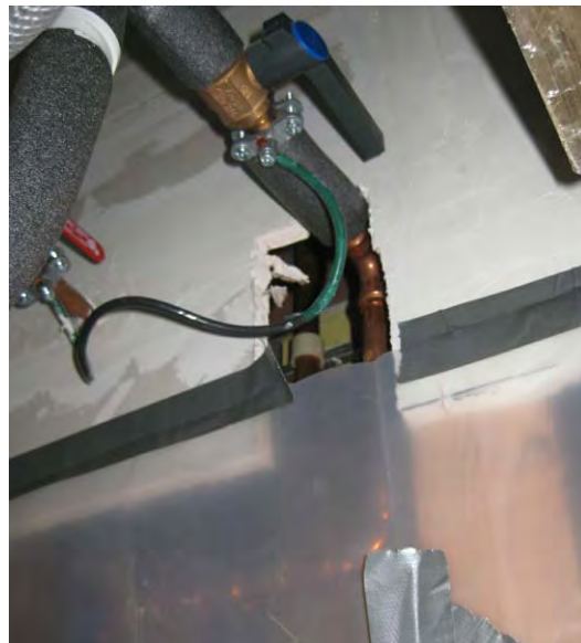
Figure 2: Mechanical room, showing open penetration connected to mechanical core
