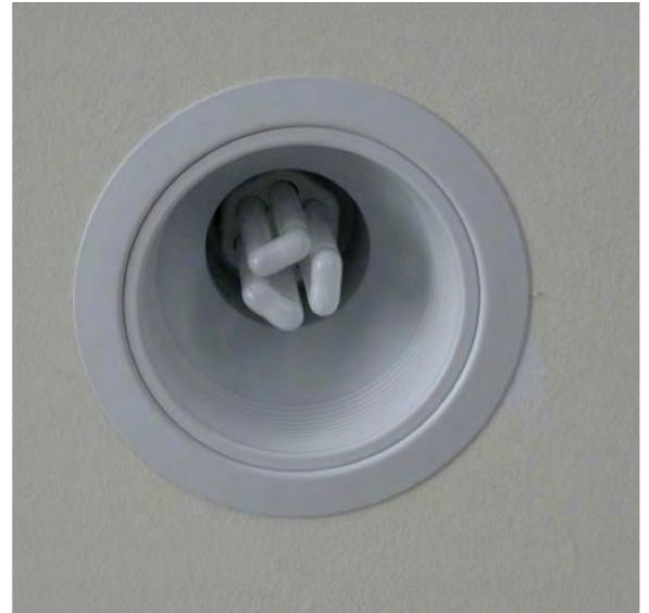
Figure 10.3.20: Pin-based compact fluorescent light recessed fixtures (in
