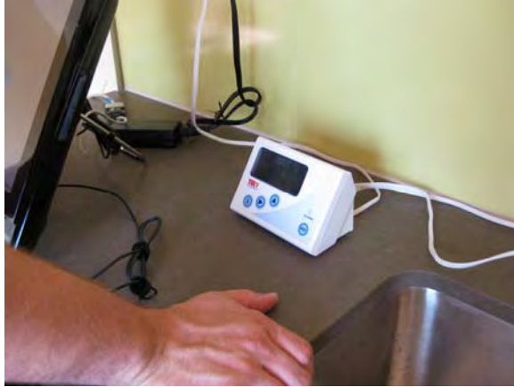
Figure 22: TED installed at kitchen counter
