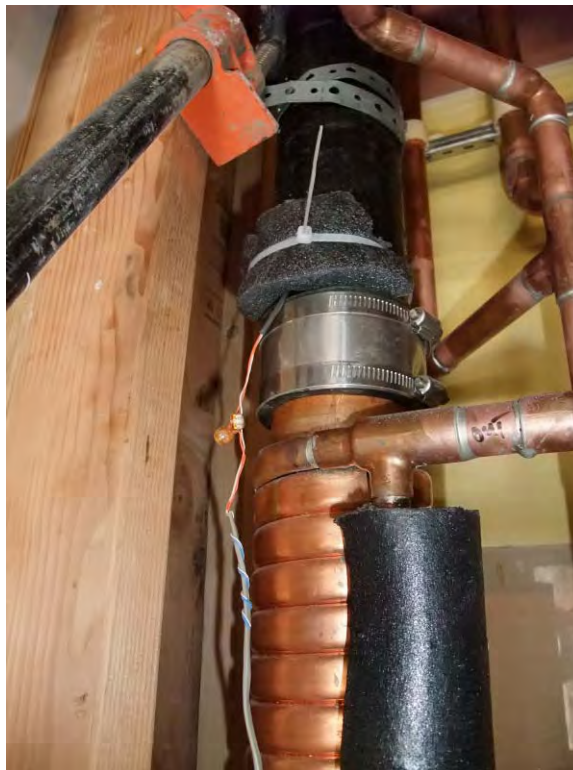
Figure 26: Incoming drainwater pipe temperature sensor (thermistors)
