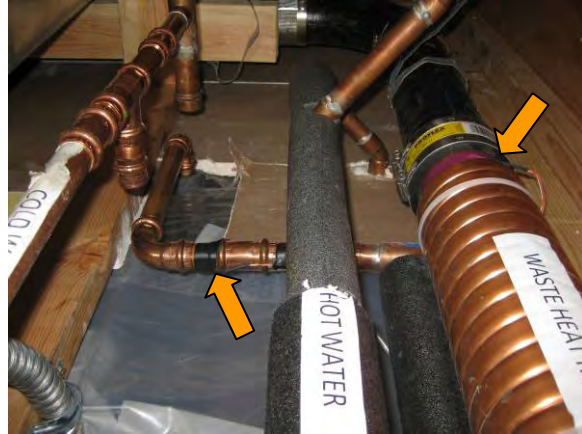
Figure 16: Tempered water output sensor (left) and incoming drain water temperature (right)
