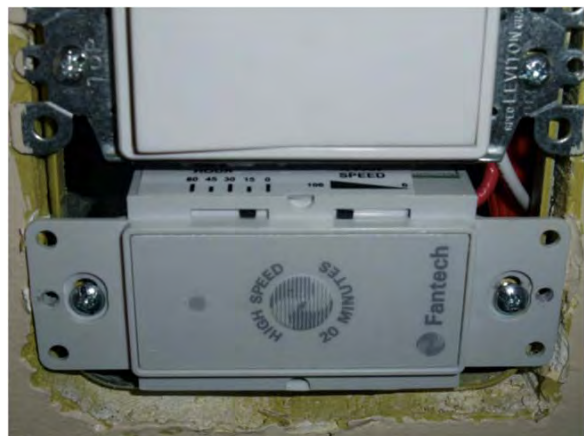
Figure 10.3.17: Fantech Ventech fan controller (bathroom exhaust + dilution ventilation runtime)
