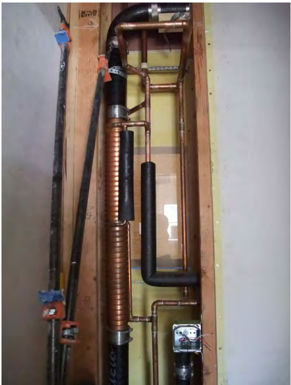
Figure 25: Drainwater heat recovery plumbing setup
