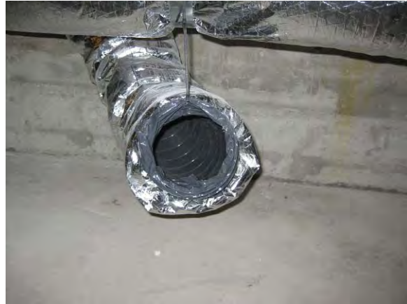
Figure 11: Data logger placed in open duct in basement (‘Bsmt Duct’)
