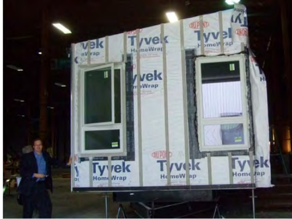
Figure 10.5.7: Fiber cement furring strip installation at Artisan Matrix panel cladding
