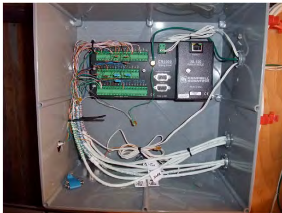
Figure 10.4.13: Data acquisition system installed at Lancaster prototype
