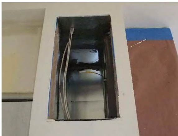
Figure 30: T/RH sensor installed in second floor return duct
