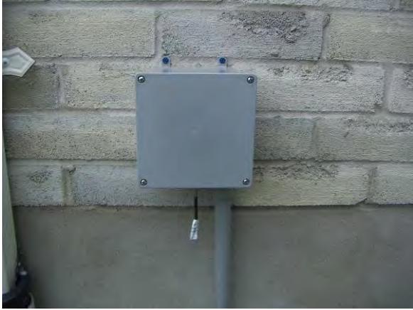
Figure 2: Outdoor electrical box with sensor as example
