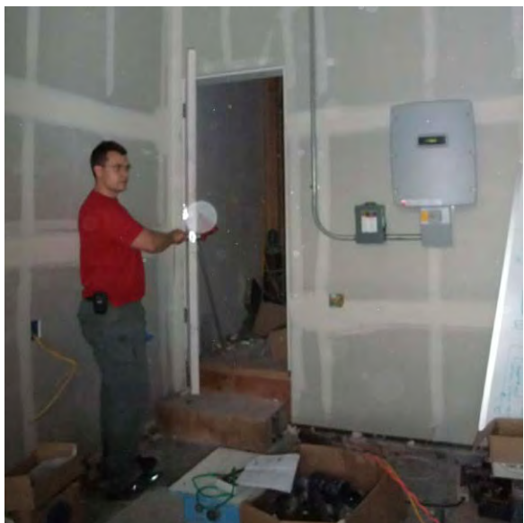
Figure 3: Mechanical room door open
