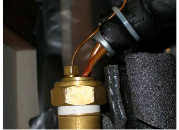
Figure 10.3.11: Kinked fitting on AirTap water heater
