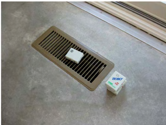
Figure 10.4.7: Use of data loggers to collect delivered register air temperature
