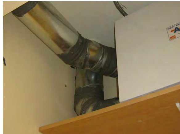
Figure 11: Available space on left hand side of HRV installation
