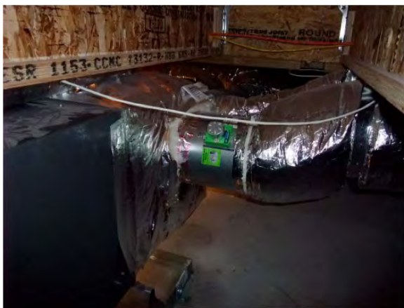
Figure 10.5.3: Economizer duct connected to return, showing motorized damper
