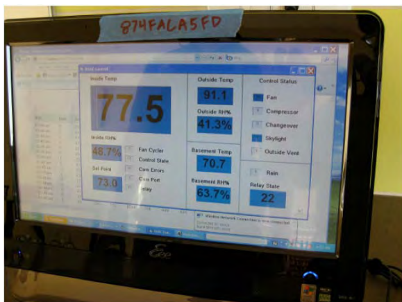
Figure 10.3.23: zTherm controller computer screen interface
