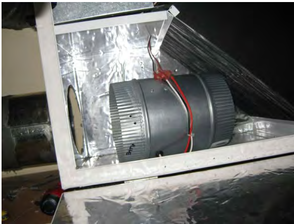
Figure 10: Removal of HRV exhaust side fan for reversal of flow direction
