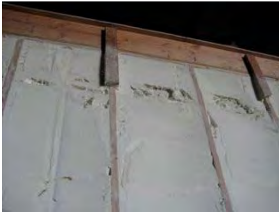
Figure 10.3.3: Spray foam installation (walls) showing excessive “shaving” of surface
