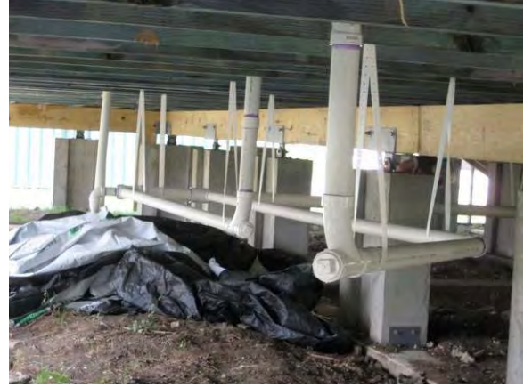
Figure 9.4.6: Plumbing below floor joists
