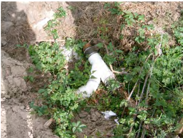
Figure 1.1 – Broken Cast Iron Sewer Line
