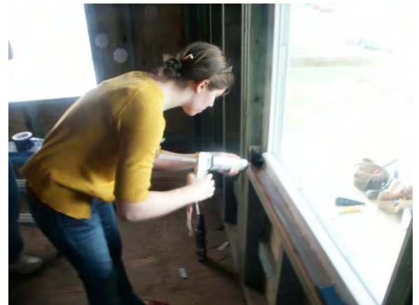
Figure 9.4.12: Installing air seal between top of wood sill and back of sill pan
