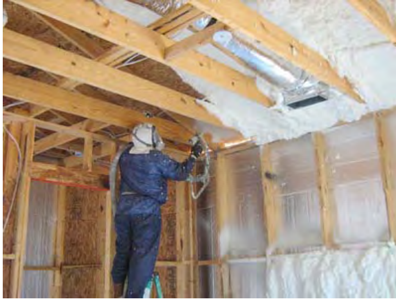
Figure 8.3-15: Low density open cell spray foam being installed in the unvented cathedralized attic and exterior walls
