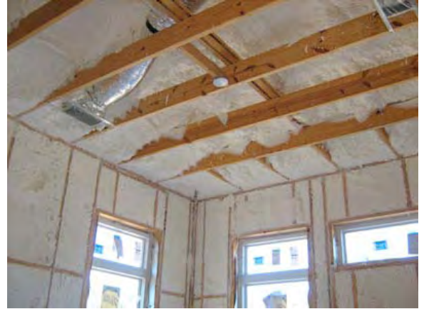
Figure 8.3-16: Low density open cell spray foam installed and shaved prior to drywall installation
