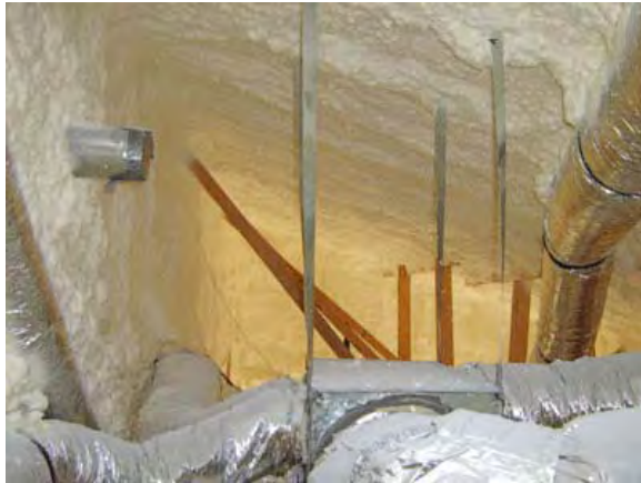
Figure 8.3-3: Unvented cathedralized attic with foam installed at the roof and knee walls
