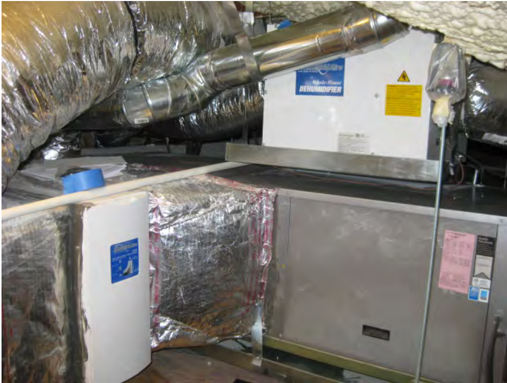
Figure 5: GeneralAire Model 1300 installed on top of air handler
