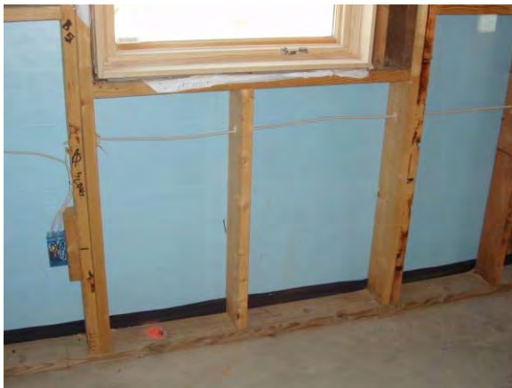
Figure 7.3-9: No cripples installed next to the jack studs
