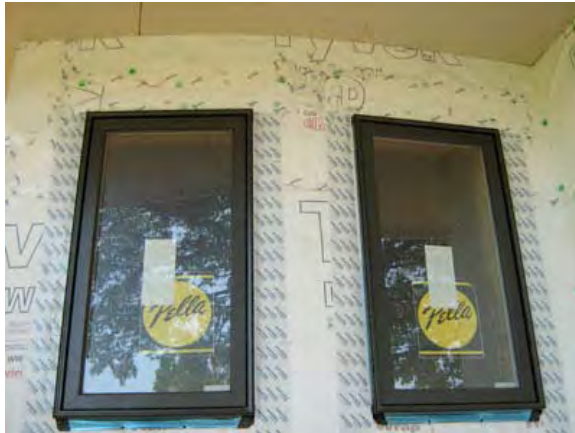
Figure 7.3-11: Fiberglass LoE 3 windows
