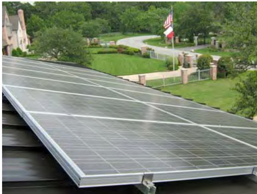
Figure 7.3-22: 3.0 kW Photovoltaic System
