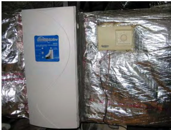
Figure 7.3-20: (L-R) GeneralAire® AC22 Filter and Aprilaire® 8126 VCS control panel on supply plenum
