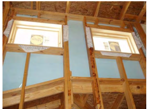
Figure 7.3-10: Two windows with no adjacent to jack studs
