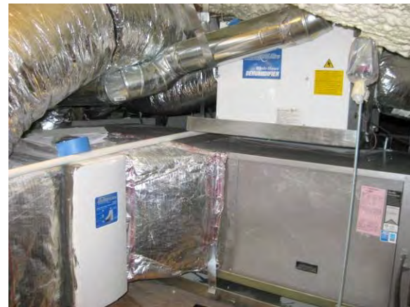
Figure 7.3-21: (L-R) GeneralAire® AC22 Filter, WaterFurnace® Air Handler and GeneralAire® Model 1300 whole house dehumidifier on top of air handler
