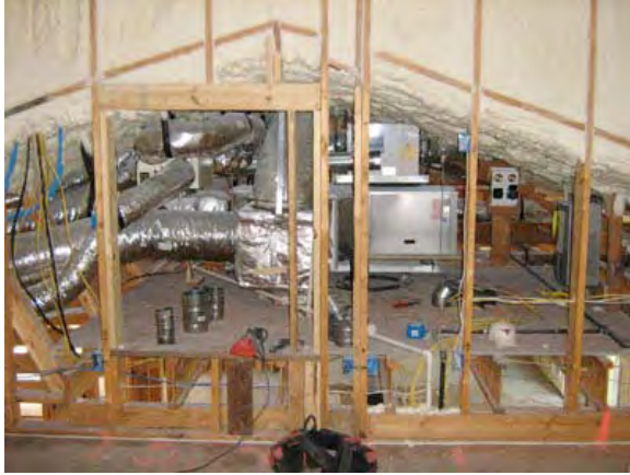
Figure 7.3-3: Unvented cathedralized attic with foam installed
