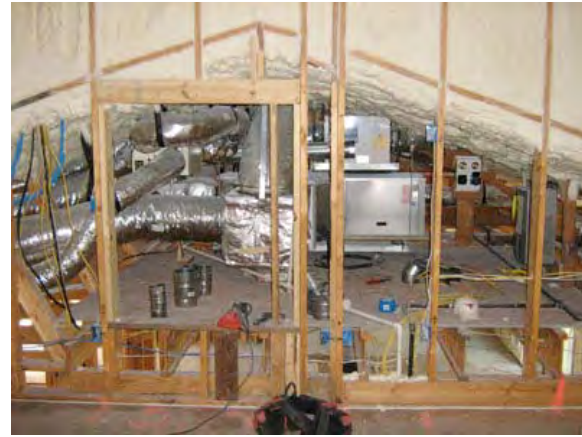
Figure 7.3-18: HVAC system located in the conditioned unvented cathedralized attic
