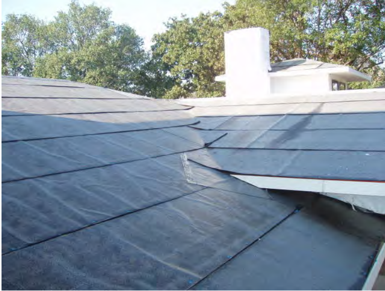
Figure 3: Fully adhered roof membrane installed over roof sheathing as underlayment for standing seam metal roof
