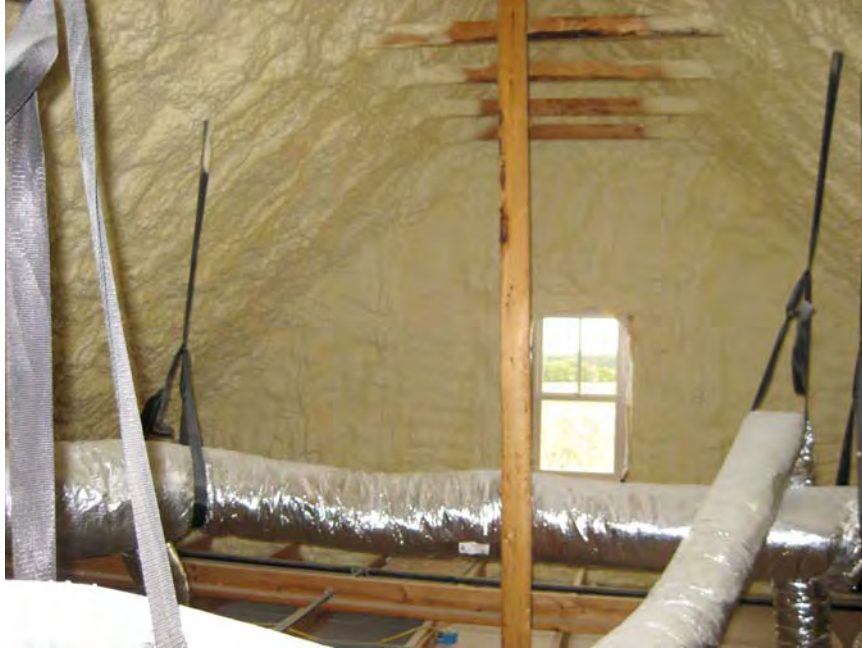
Figure 6.3.19: Unvented cathedralized attic with R-30 open cell low density spray foam installed under the roof deck
