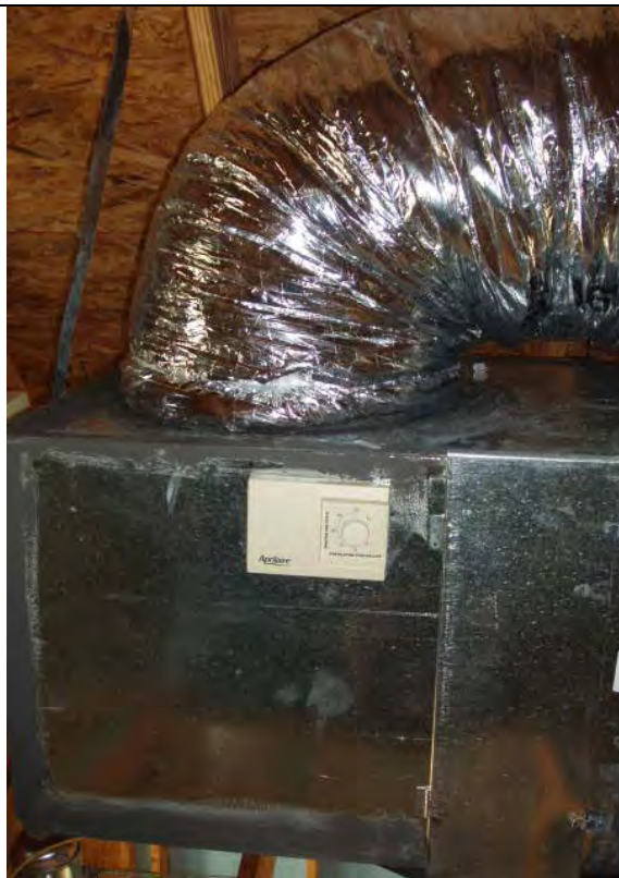
Aprilaire 8126 VSC fan cycler installed
