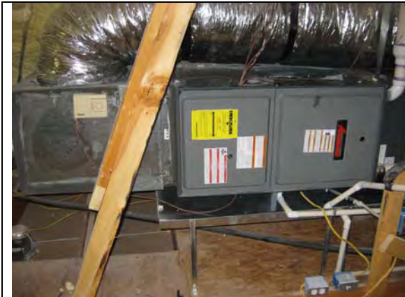
Ductwork with dehumidifier showing
