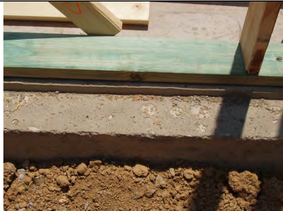
Bottom plate with stepped down slab edge for brick veneer front wall
