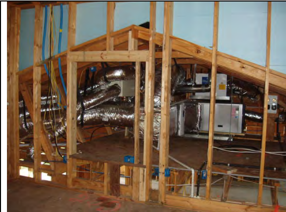
HVAC system in unvented attic space
