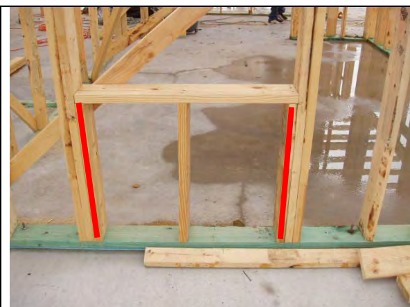
Window sill framing – edge cripples (in red) not necessary
