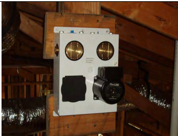
Water Furnace® GeoLink® Flow Center will feed both the hot water tank and HVAC system.
