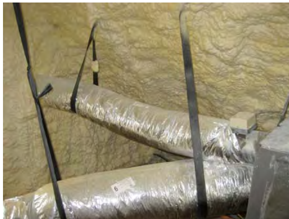
Figure 6.3.28: 6" insulated flex duct installed as an outside air duct that draws in outside air to the return plenum
