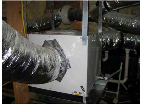
Figure 6.3.27: Dehumidifier integrated with duct system in the conditioned unvented cathedralized attic
