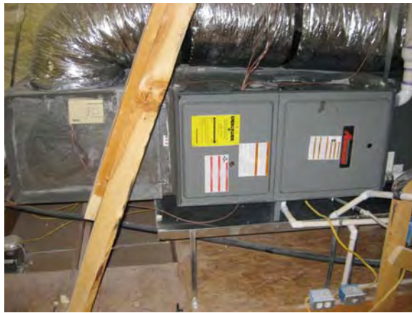
Figure 6.3.23: Unit 1 (3-ton) for the first floor
