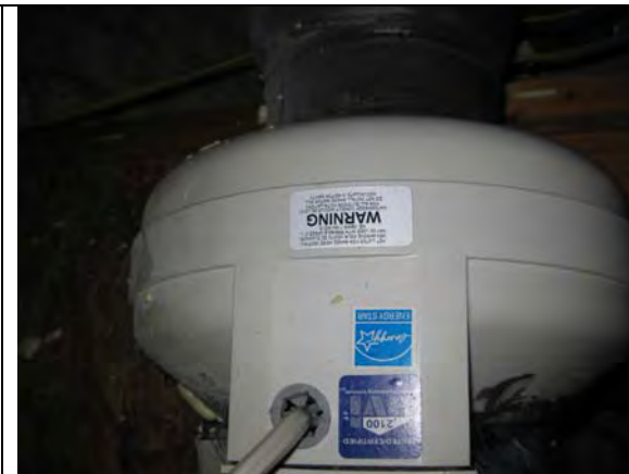
Inline fan connecting the three bathrooms to the outside via a single duct
