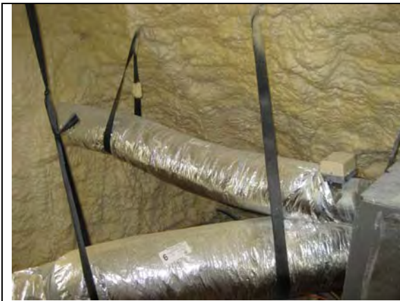
6" outside air duct with mechanical damper at return plenum
