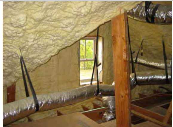
Ductwork in cathedralized attic
