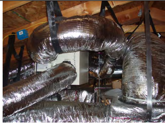
GeneralAire ERV coupled to outside air duct
