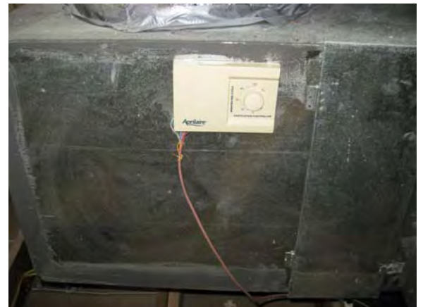
Figure 6.3.29: Aprilaire® 8126 VCS fan cycling control installed on the return plenum
