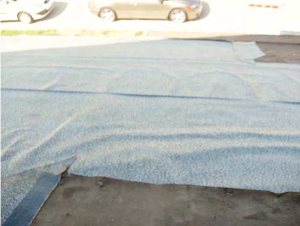
Figure 3: Fully adhered roof membrane installed at edges and at roof intersections with #30 felt in the roof field for composition shingle roof.
