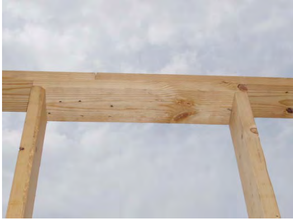
Figure 6.3.8: One method of joining the single top plates together: through a 24" splice
