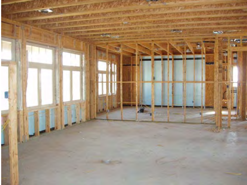
Figure 6.3.12: ¾” XPS insulating sheathing with ½ OSB at the corners for structural support
