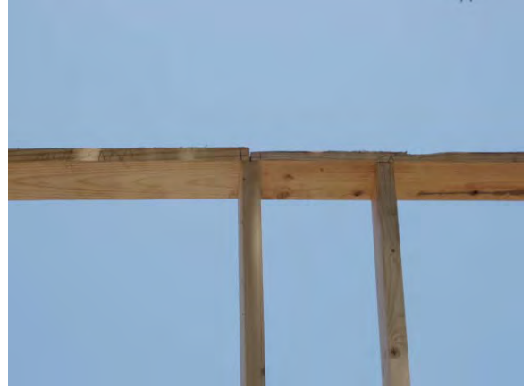
Figure 6.3.9: Another method of joining the single top plates together: line the joint on top of an existing stud
