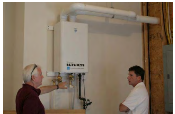
Figure 5.3.8: Terrance Babbie and BSC's Armin Rudd with Navien water heater
