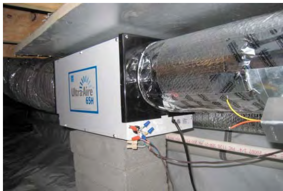
Figure 5.3.7: Dehumidifier installed in crawlspace
