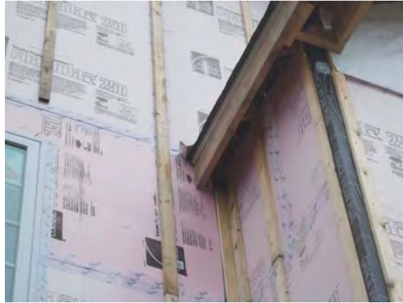
Figure 4.4.2: Kick out flashing at roof to wall and self-adhered membrane at building corners
