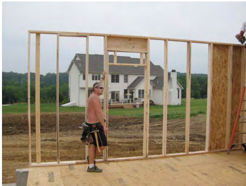
Figure 4.4.1: Advanced framing (lateral brace panel in corner, single header, single top and bottom plates)
