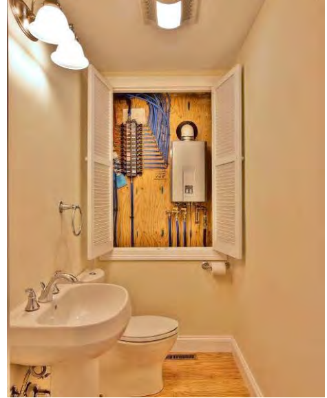
Figure 3.4: On demand, sealed combustion hot water heater is located close to plumbing fixtures
