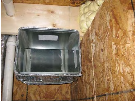
Figure 3.15: Supply plenum showing mastic applied to the inside of the duct
