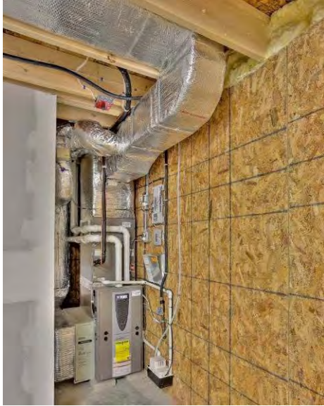
Figure 3.3: Premium efficiency, sealed combustion propane furnace is paired with a premium efficiency heat pump
