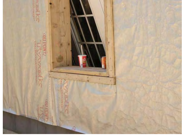
Figure 3.14: Prior to BSC guided demonstration window openings had been prepared with 2x bucks over the drainage plane and proud of the sheathing plane, strapping applied around window
