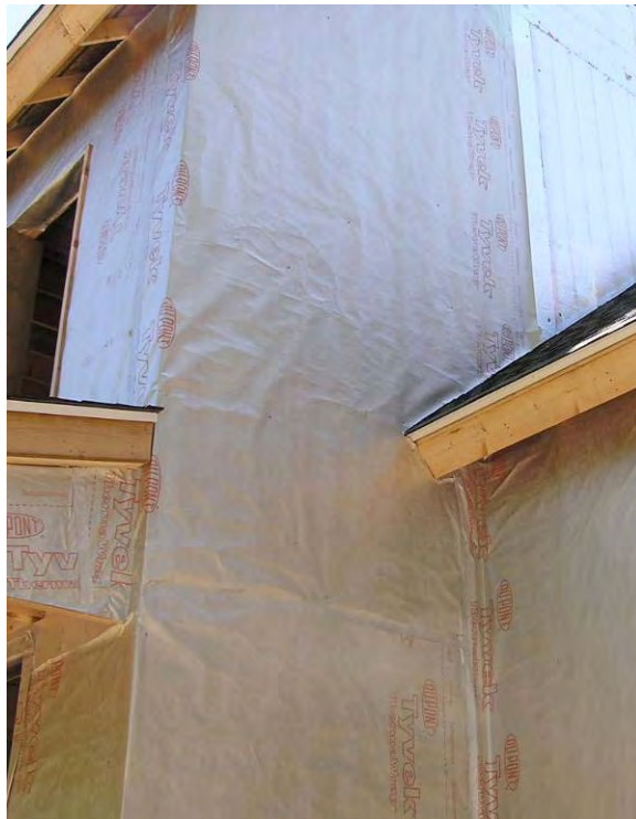
Figure 3.11: Step flashing installed behind the insulating sheathing drainage plane risked injecting water into the wall assembly
