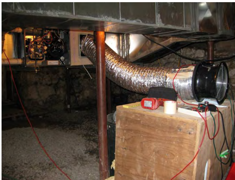
Figure 8 - duct blaster installation at air handler in basement
