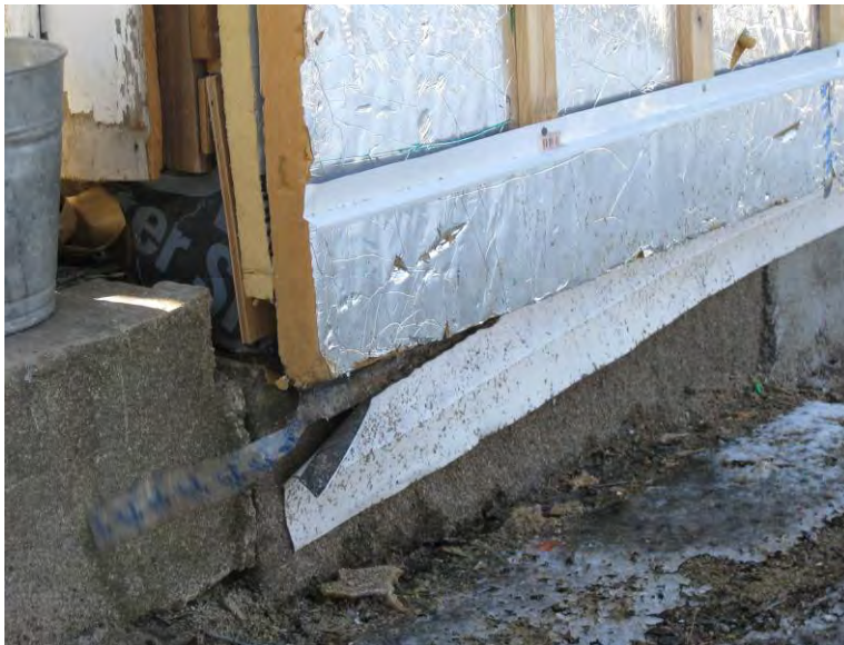
Figure 16 - transition membrane at Northeast corner failed to re-adhere after replacement of sheathing board
