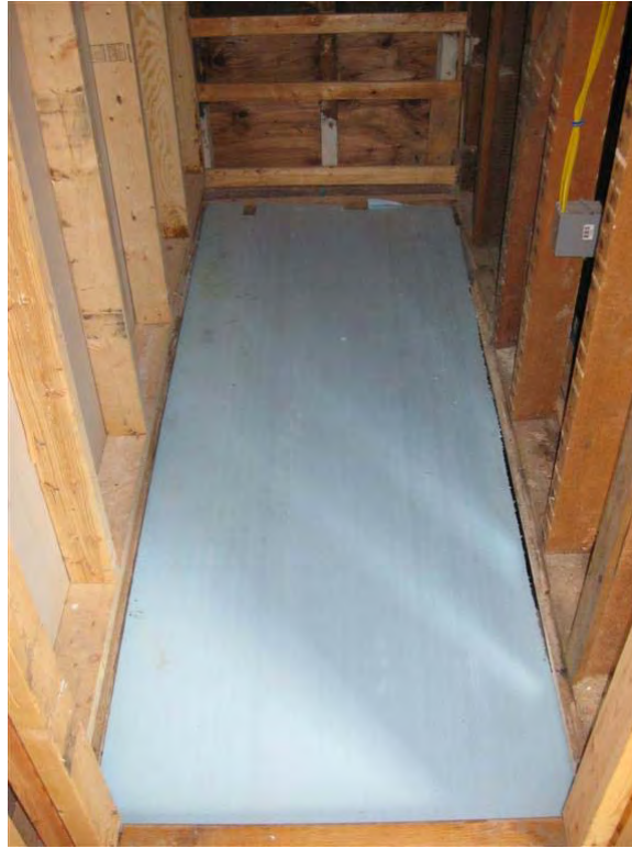
Figure 3 - XPS blocking at stair opening
