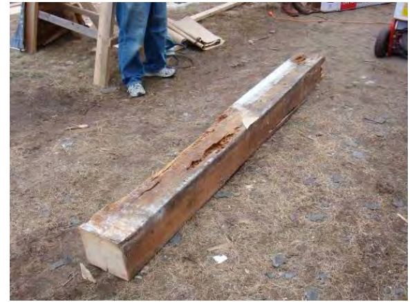
Figure 2.20: Sill beam decay noted at foundation-contact portions
