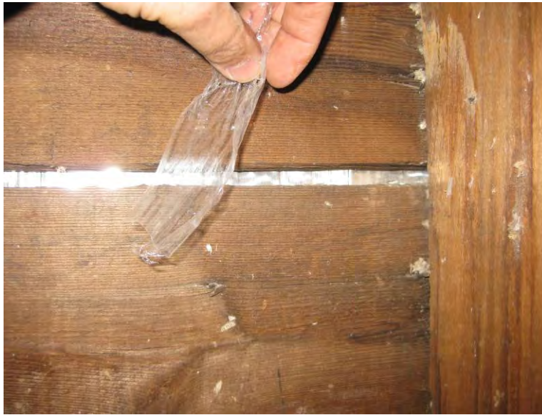
Figure 18 - air flow observed between sheathing boards near inside corner
