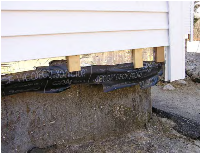
Figure 15 - flashing membrane did not adhere to the StraightFlash VF transition membrane
