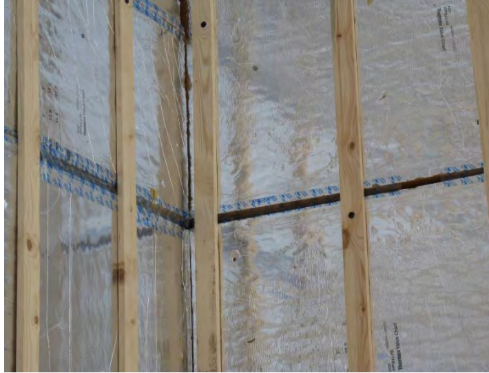
Figure 2 - Gaps in Foam Sheathing
