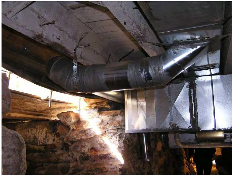
Figure 19 - duct work as observed at earlier site visit
