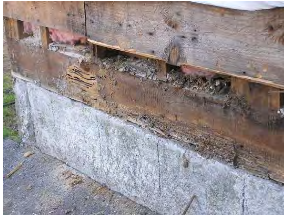
Figure 2.19: Sill beam decay visible after removal of board sheathing
