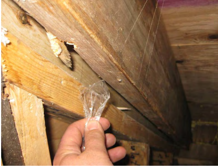
Figure 10 – observation of air flow at narrow rafter bay at addition roof rake
