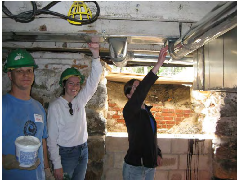
Figure 20 - Habitat volunteers and a BSC staffer locating duct leaks
