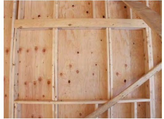
Figure 1.5.2: 2x4s extend from floor to ceiling, 2x6 sill provides continuous sill for all 3 windows
