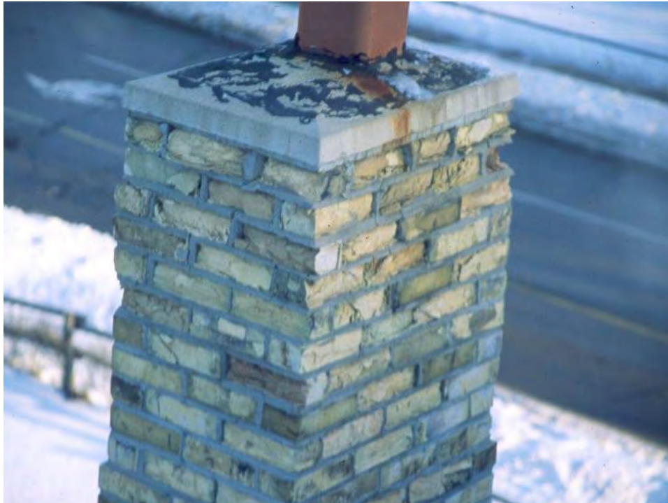
Figure 59: Severe freeze-thaw damage at existing chimney; lack of projecting cap with drip edge
