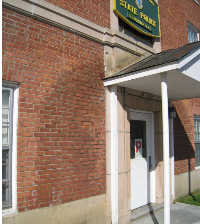
Figure 54: Water runoff concentration at roof-wall interface (kickout flashing required)
