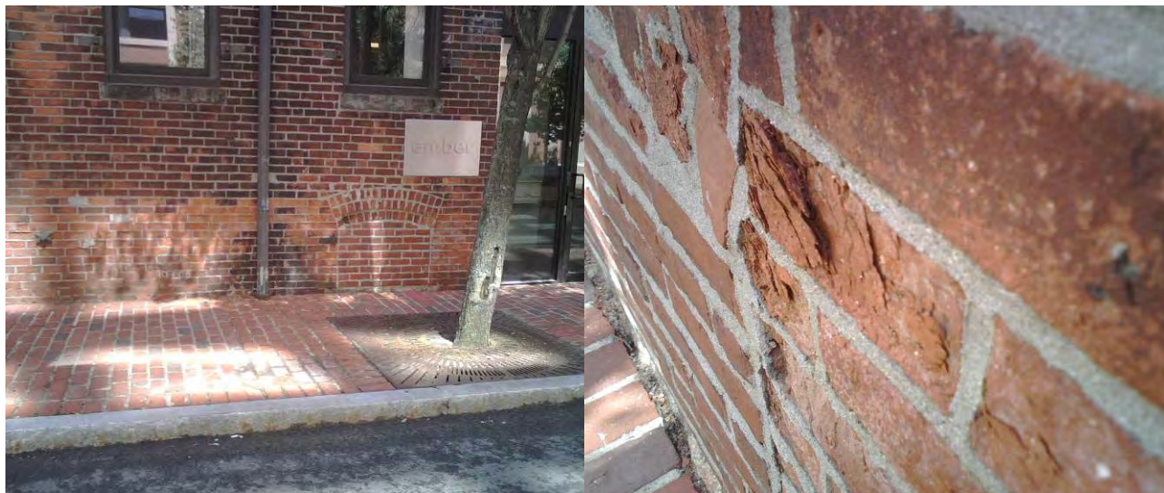
Figure 65: Freeze-thaw damage at downspout disconnection (L), delamination of brick (R)
