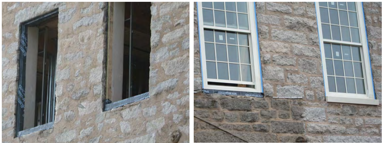
Figure 45: Membrane flashing wrapping window opening (L), and exterior view of window assembly and completed unit (R)
