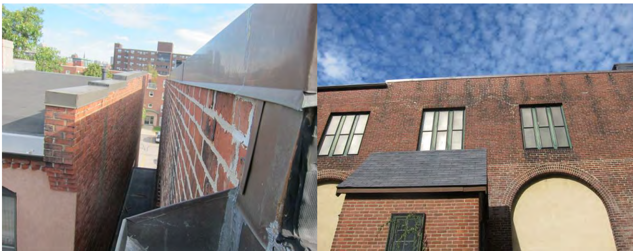
Figure 60: Coping detail and runoff staining at joints of previous coping design
