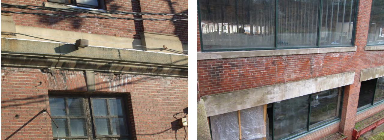
Figure 83: Exterior details that demonstrate freeze-thaw damage in existing masonry buildings
