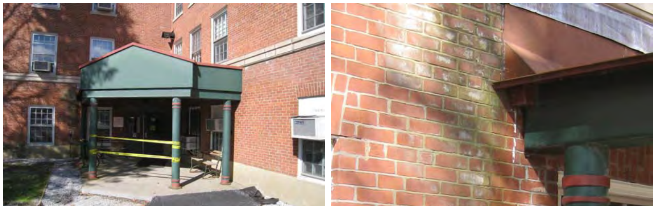
Figure 53: Retrofit roof over entrance; water runoff concentration at roof-wall interface
