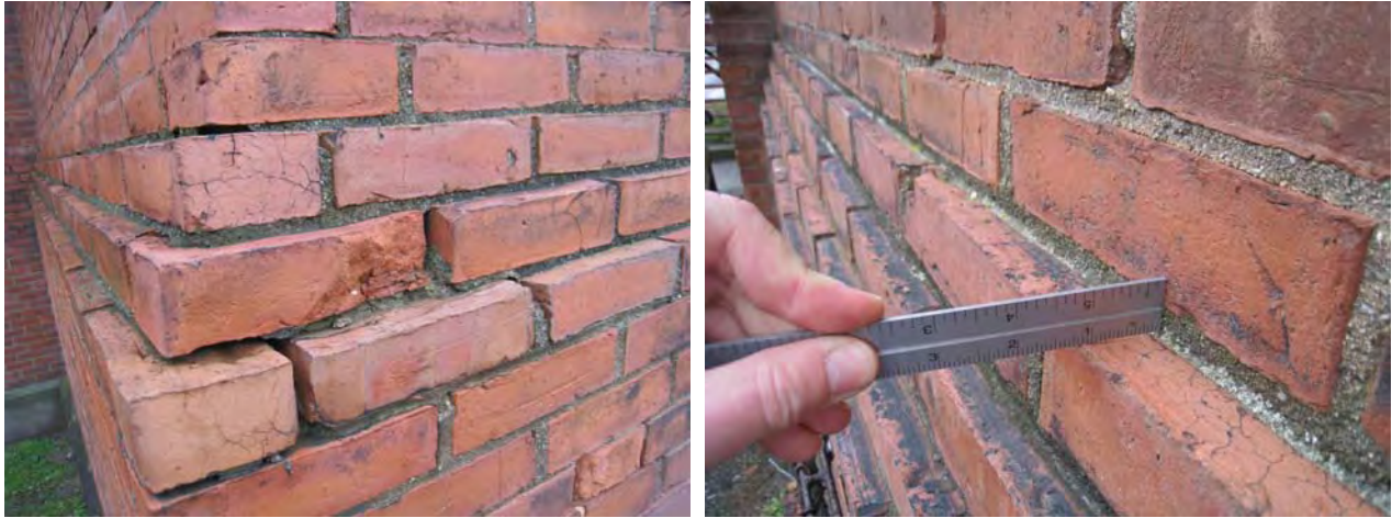
Figure 50: Steps in brickwork, and related cracking/freeze-thaw damage
