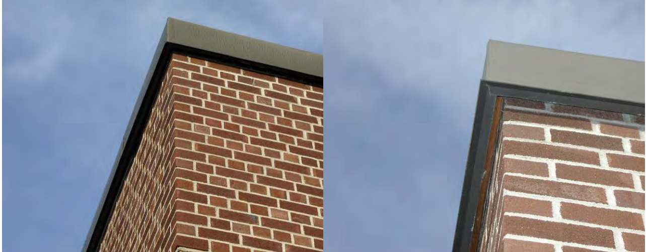
Figure 62: Improved drip edge overhang at coping
