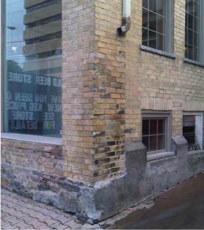
Figure 66: Disconnected downspout and related damage to masonry
