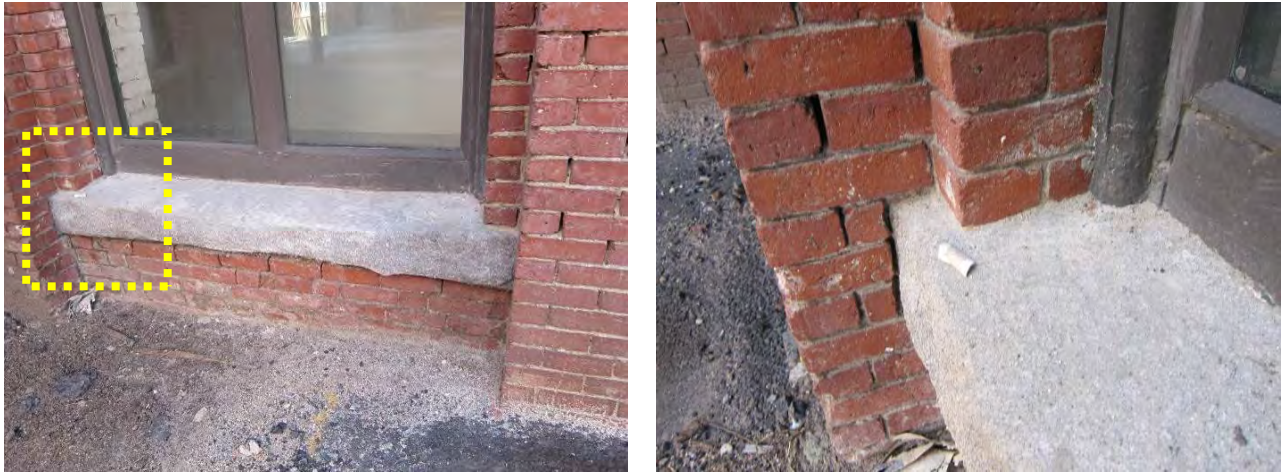
Figure 33: Solid granite sloped sill, potential for water introduction into wall
