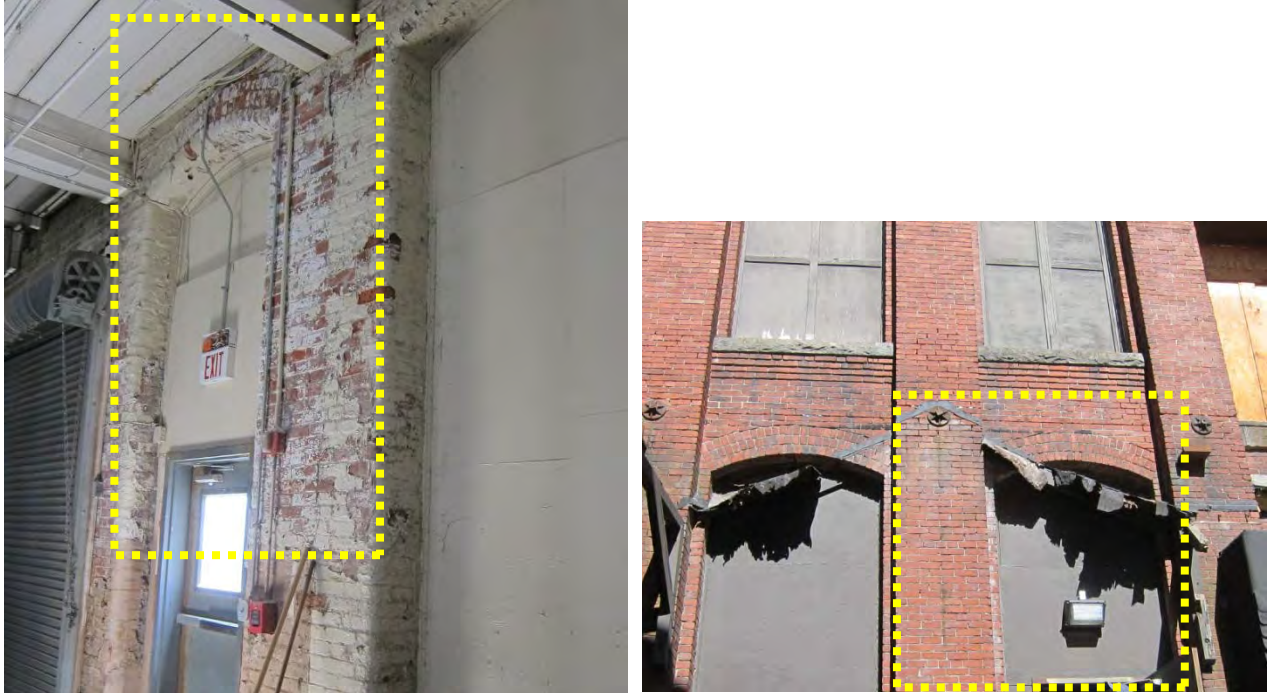
Figure 56: Interior paint/parging delamination, with exterior conditions for comparison
