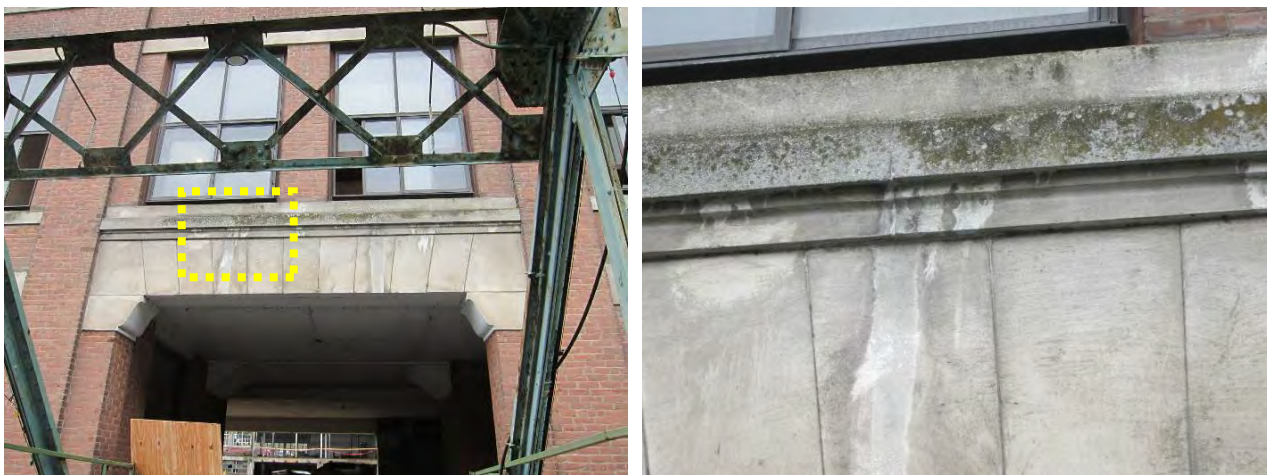
Figure 49: Staining on decorative arch coping stones, concentrations at joints
