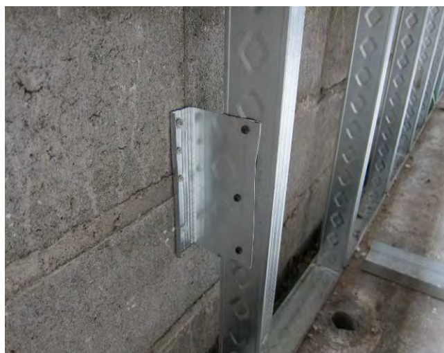
Figure 27: Clip tying framing to CMU backup wall, steel clip shown; not recommended
