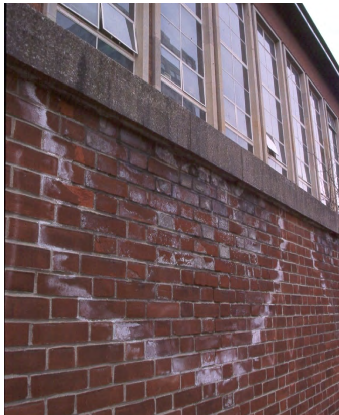
Figure 35: Failed mortar joint at sill concentrated run-off, resulting in brick failure
