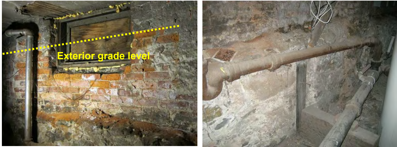
Figure 69: Severe subfluorescence/spalling at basement window; stone shelf below grade
