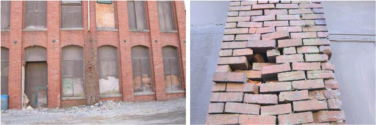
Figure 67: Damaged pilaster at downspout; severe mortar erosion
