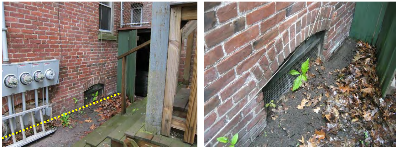
Figure 70: Rear wall near subfluorescence damage visible in basement; buried window
