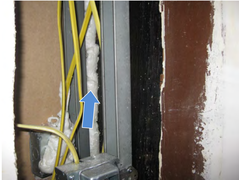
Figure 22. Airflow control connection between drywall and exterior wall achieved through open side of wall.
