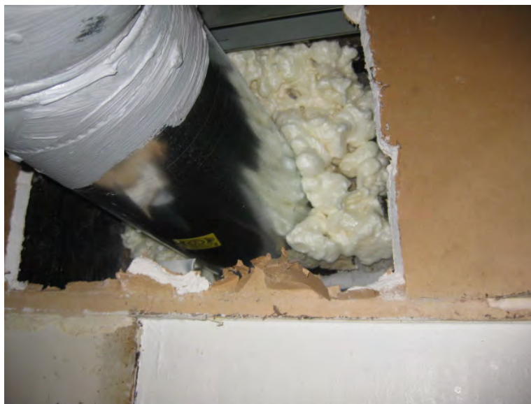
Figure 23. Large opening in drywall around exhaust duct allows access to exhaust duct penetration through CMU backup wall – the primary airflow layer for the exterior wall.
