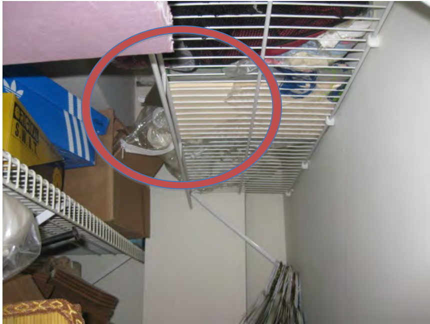
Figure 26. Duct riser to duct soffit connection at the back of a narrow closet in end-unit apartments.
