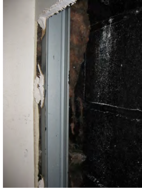
Figure 4. Furring cavity of exterior wall communicates with demising wall. Left: Drywall removed at section of exterior wall adjacent to demising wall; Right: Close-up of connection between furring cavity of exterior wall and demising wall.
