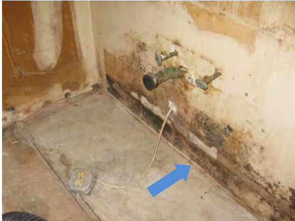
Figure 3: Apparent existing joint compound sealing at base of kitchen wall
