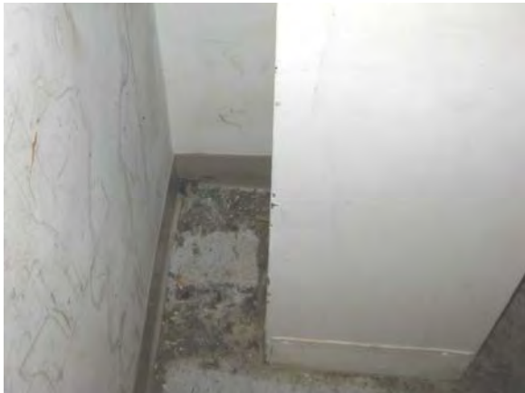
Figure 1: Copious evidence of rodent activity in second floor closet
