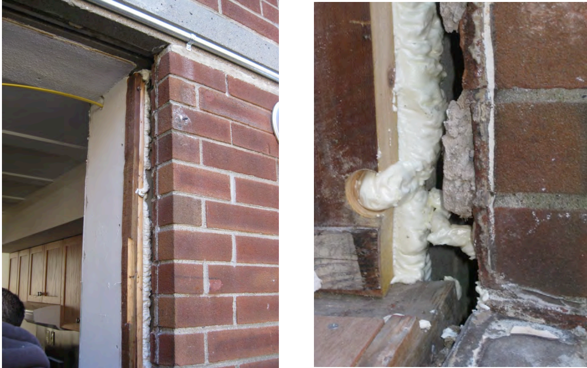
Figure 15. Left: Visual access enables verification of seal between buck and masonry opening; Right: Foam sealant in gap between wood buck and CMU backup wall.
