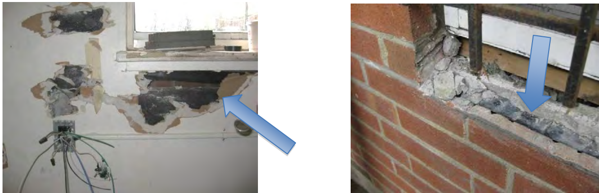
Figure 11. Destructive investigation into existing window assembly and installation. Left: Interior view of existing window installation in mock-up unit. Note the gap between masonry opening and sill; Right: Exterior view of existing window installation in mock-up unit. Note the sill membrane forming a trough that is filled with mortar.
