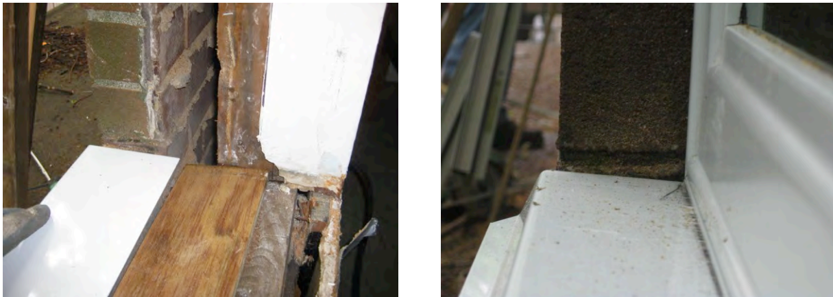
Figure 30. Left: Exterior sill trim above height of sill blocking; Right: Back-sloped sill trim.
