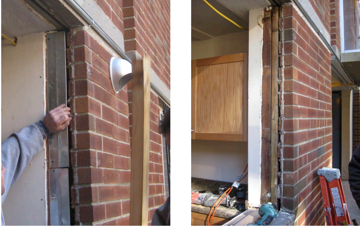
Figure 16. Left: Metal coil stock support for jamb flashing between wood buck and brick return; Right: Wood buck off-cut reattached as jamb flashing support.
