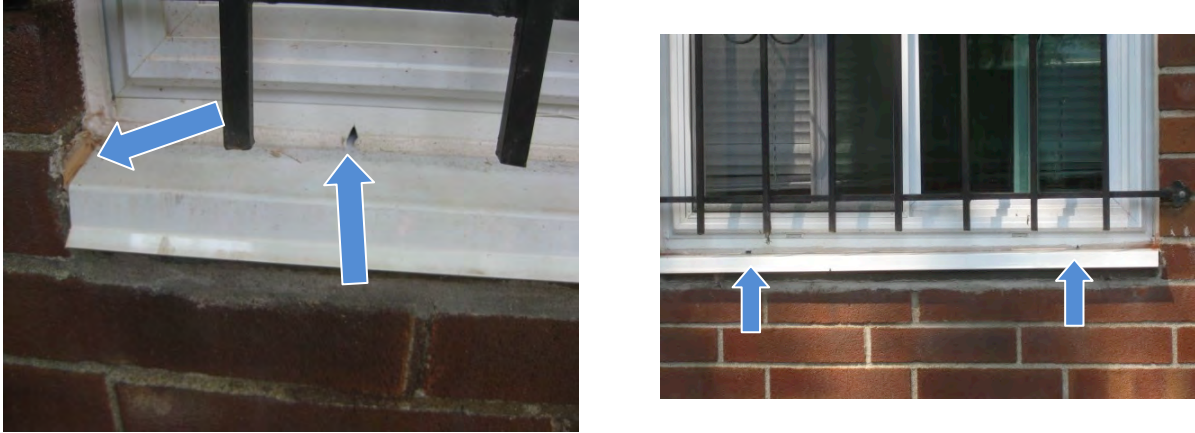
Figure 34. Left: Sealant joint between sill aluminum sill trim and brick, and “V” cut weep notched into sill trim closure; Right: Weep holes at \frac{1}{4} points of the sill closure trim.
