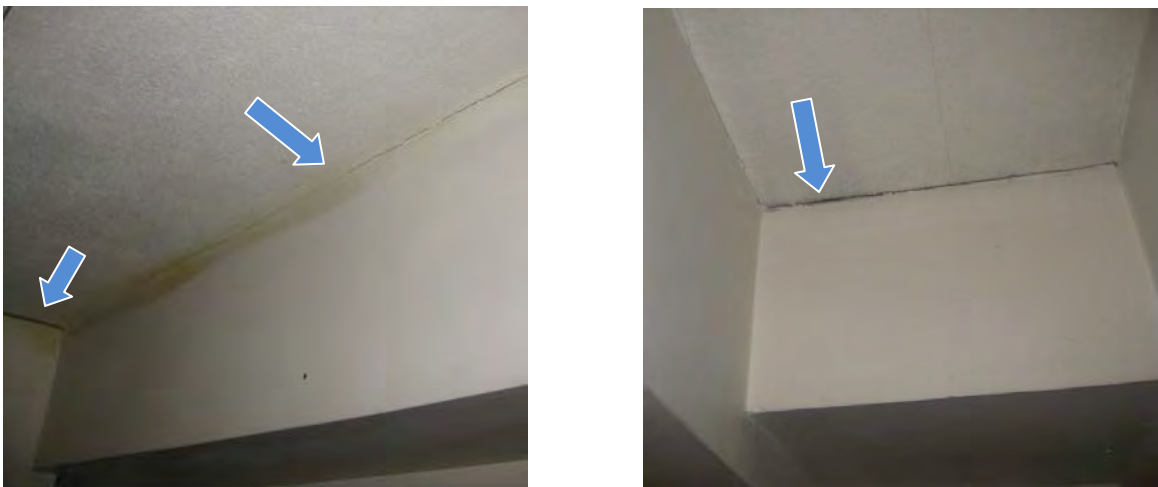
Figure 27. Gaps between drywall and floor/ceiling assembly observed at second floor
