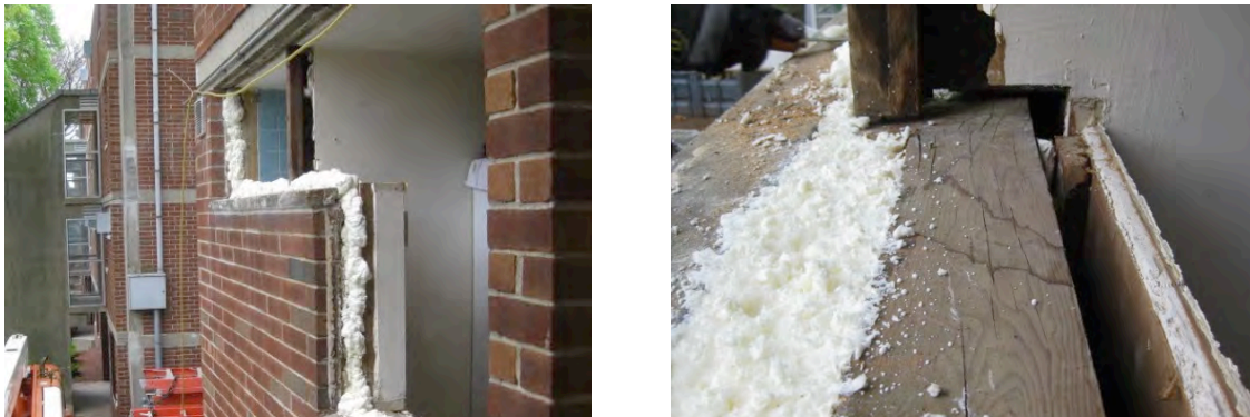
Figure 28. Left: Expanding foam sealant installed to bridge the cavity between the brick and the CMU; Right: Expanding foam sealant trimmed to provide substrate for flashing membrane.
