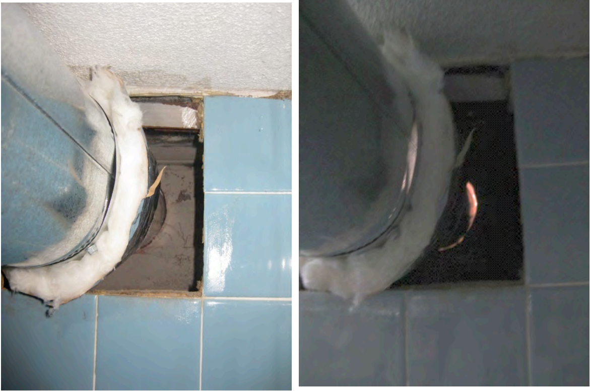
Figure 20. Left: Early attempt at sealing exhaust duct. Note annular seal between sleeve and duct but not between duct sections or sleeve and wall; Right: Backlit image of early attempt at sealing exhaust duct illustrates where air seal is needed.
