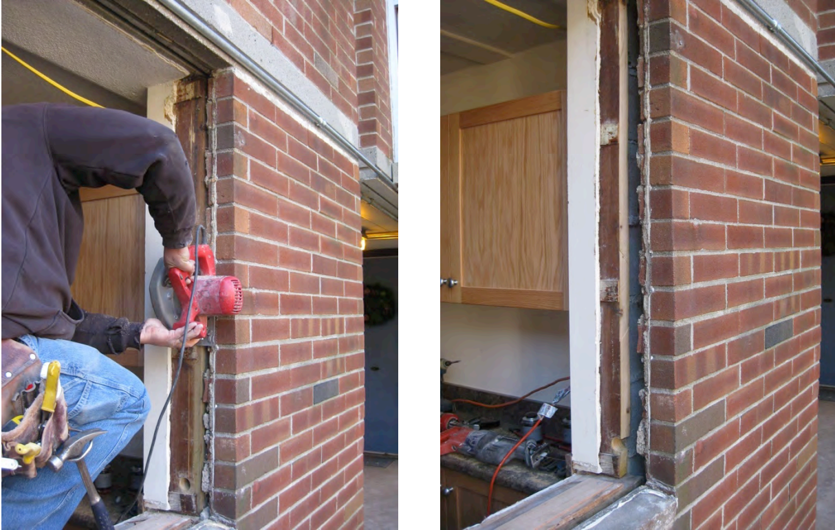
Figure 13. Left: Wood jamb buck being cut to allow access to joint between buck and masonry opening; Right: Wood jamb buck cut showing both working and visual access to the gap to be sealed.
