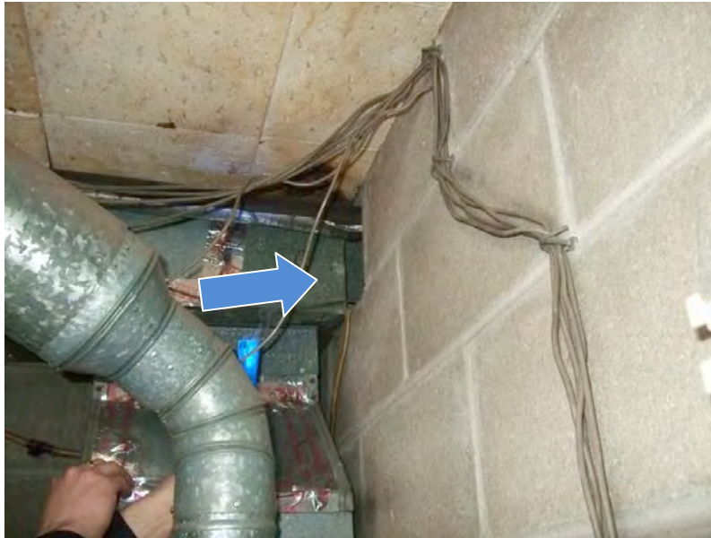
Figure 2. Typical gap around supply plenum in separation between mechanical room and apartment.
