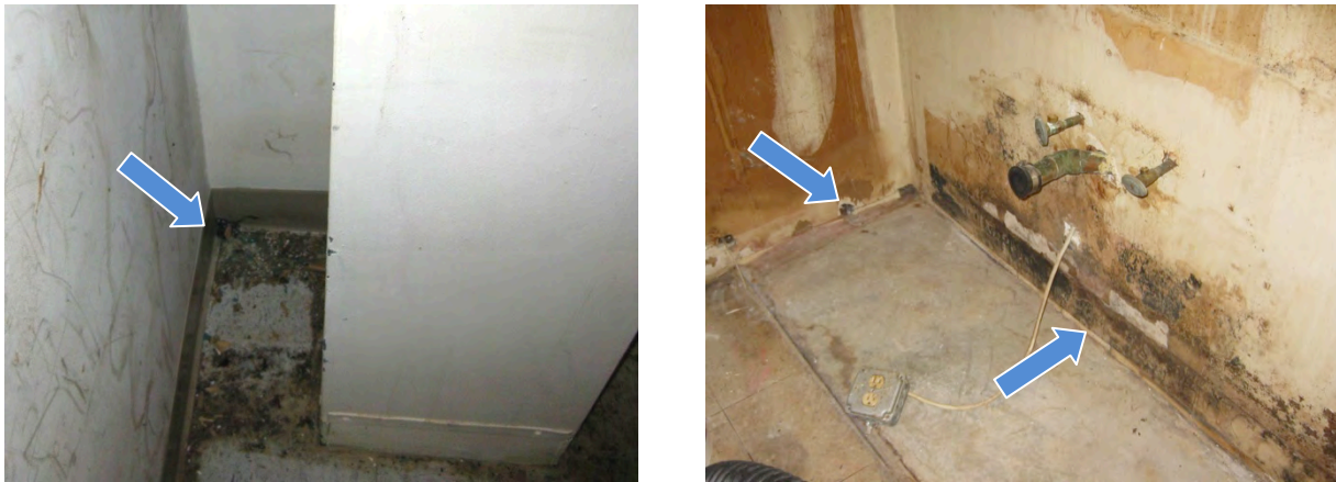
Figure 17. Left: Copious evidence of rodent activity on floor of second floor closet; Right: Rodent hole behind kitchen cabinet location and apparent pre-existing attempt at sealing base of wall to floor with joint compound.
