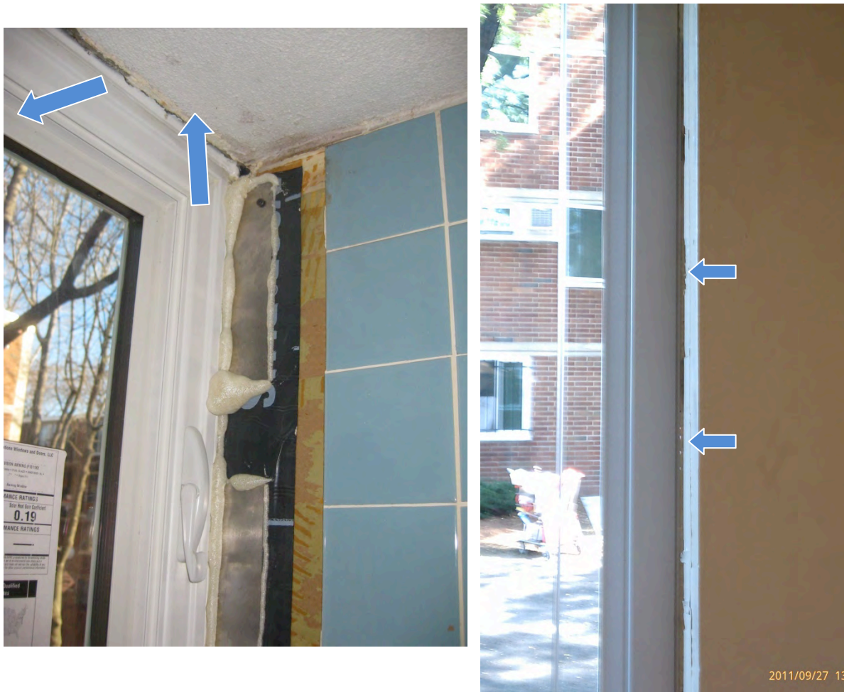
Figure 35. Left: Expanding foam sealant at window jamb and fillet bead of sealant at head of early window installation; Right: Poor seal at window perimeter with gaps permitting view to outside.
