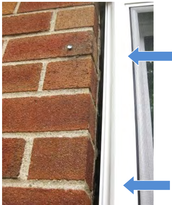
Figure 32. Jamb flashing membrane poorly adhered to brick substrate as evident in gaps between the membrane and the brick.
