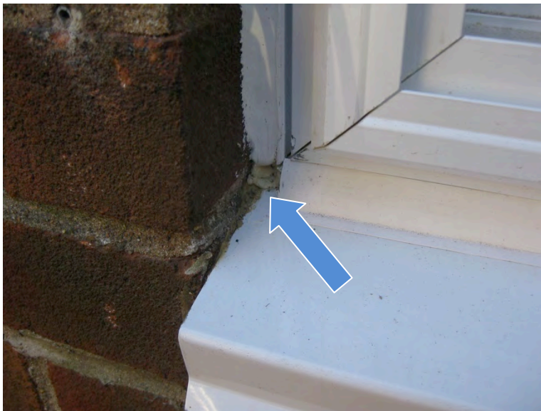
Figure 33. Sealant joint stopped short to allow drainage also presents potential path of water entry.
