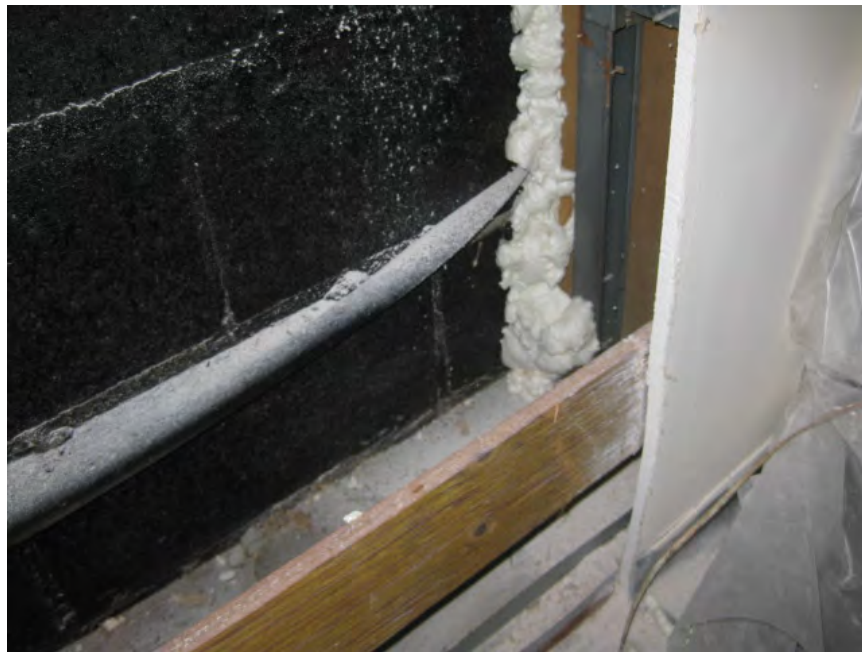
Figure 24. Inside of CMU layer in exterior wall. Note dampproof coating and through-wall flashing
