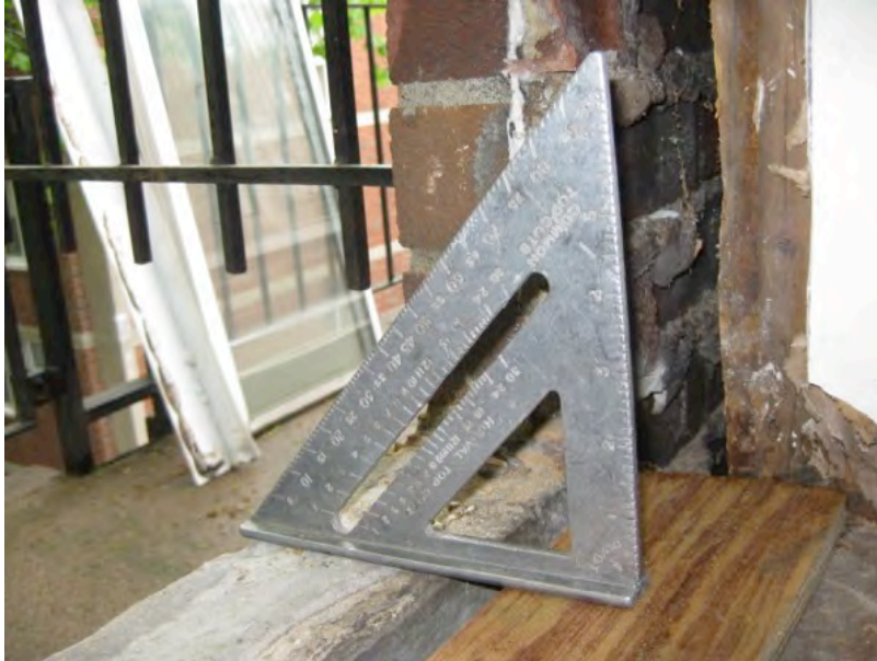
Figure 29. Sill blocking even with height of exterior sill prior to installation of exterior sill trim piece.
