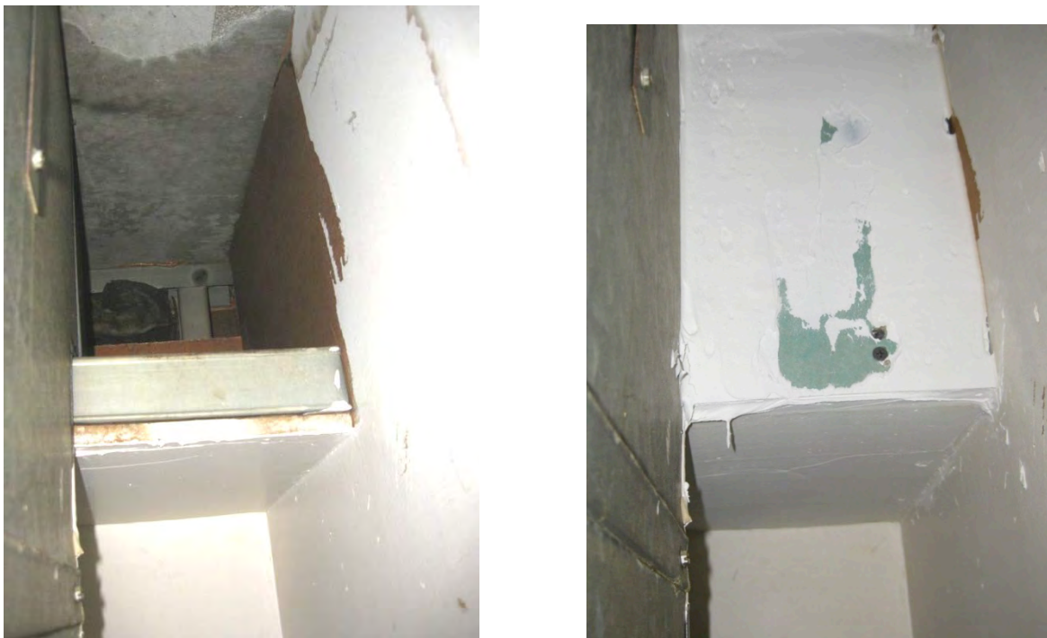
Figure 19. Left: Opening into duct soffit along side vertical riser. View into soffit and demising wall cavity (with dirty batt insulation) beyond; Right: drywall closure for duct soffit.
