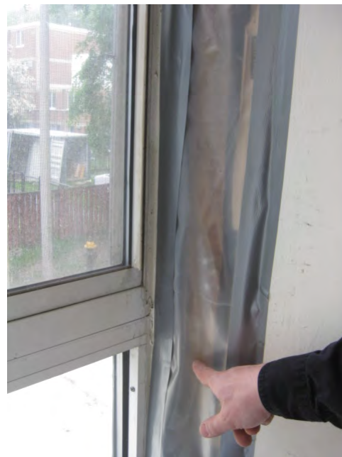
Figure 25. Left: Plastic sheeting at sill of window opening billowing inward during depressurization testing; Right: Plastic sheeting at window jamb return billowing inward during depressurization testing.
