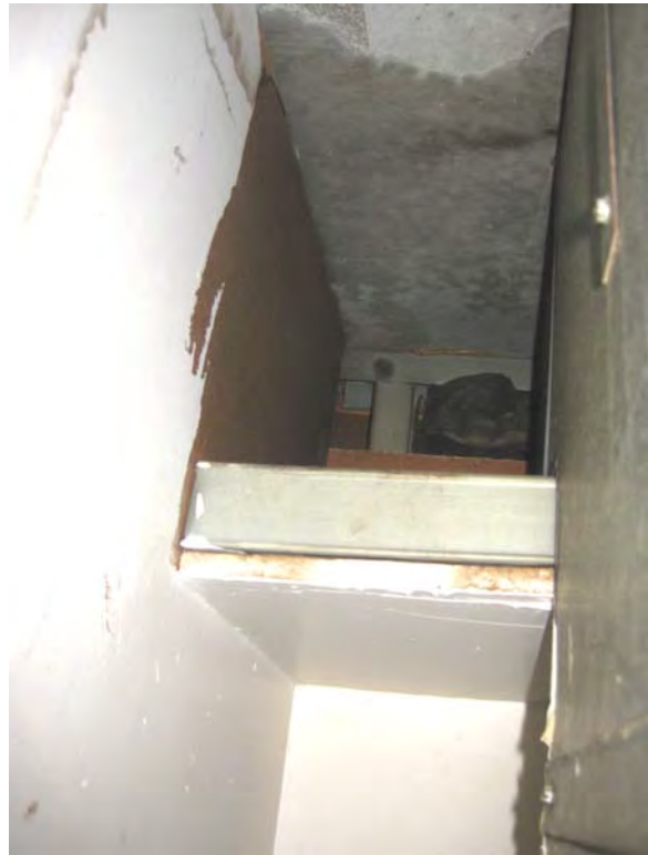
Figure 7: Opening into soffit at second floor of present low-rise mock-up apartment. Note opening into demising wall.
