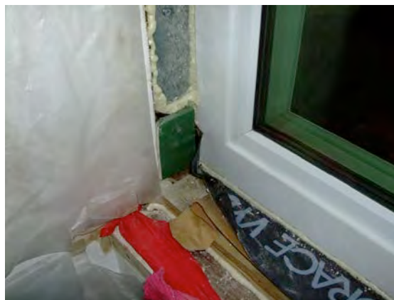
Figure 31. Corner of sill pan flashing in a very tight spot. Note that backing is left on the portion of the flashing membrane to the inside of the window to facilitate turning the membrane up at the sill to form a back dam.
