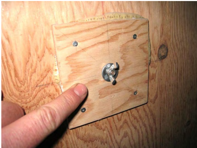
Figure 15 – Wing nut, washer and bearing plate in the field of the back panel (typ. of 14)
