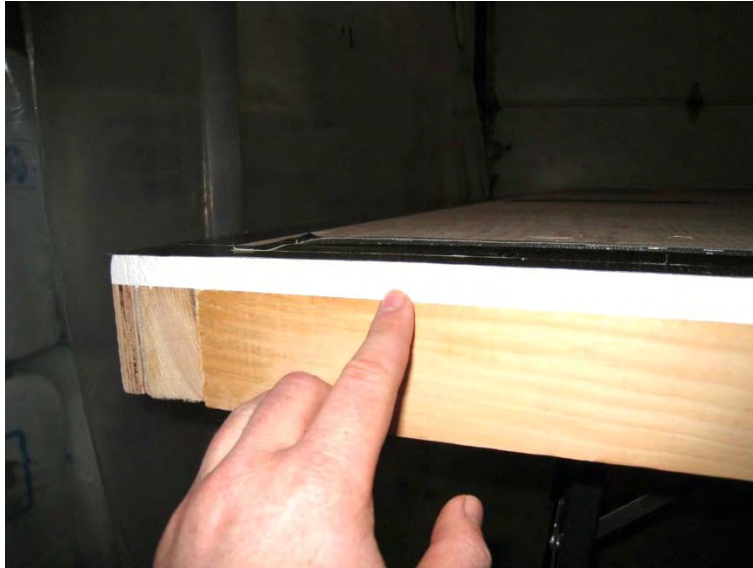
Figure 11 – Air seal coating applied to top & bottom edge of plywood on back panel
