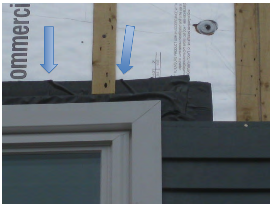
Figure 49. Wrinkles in flashing membrane wrapped over strapping and back to drainage plane. Note how this window head flashing requires flashing of its own.
