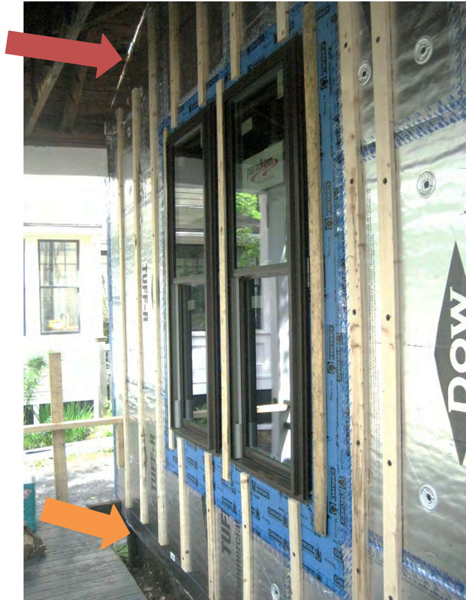
Figure 41. Porch deck, ceiling, and roof cut away from wall to allow continuous air, thermal, and water control, Test Home 2
