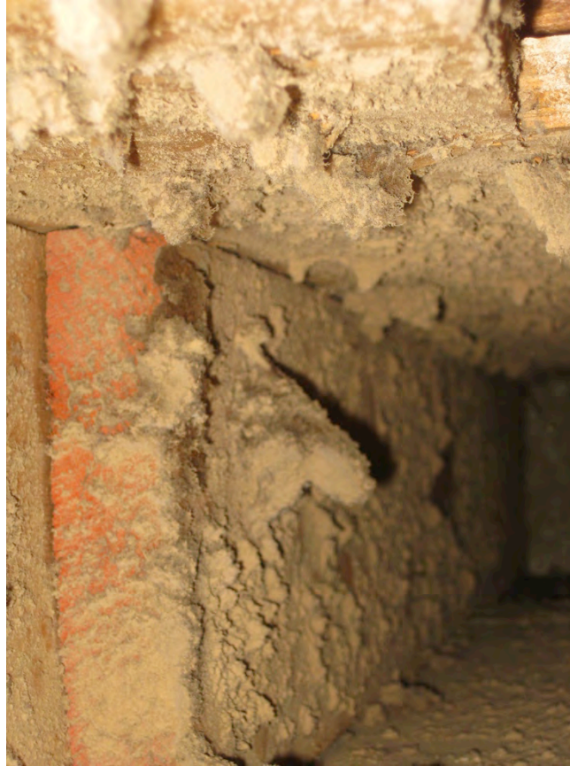
Figure 4. View inside framing cavity forced-air duct return at Test Home 1
