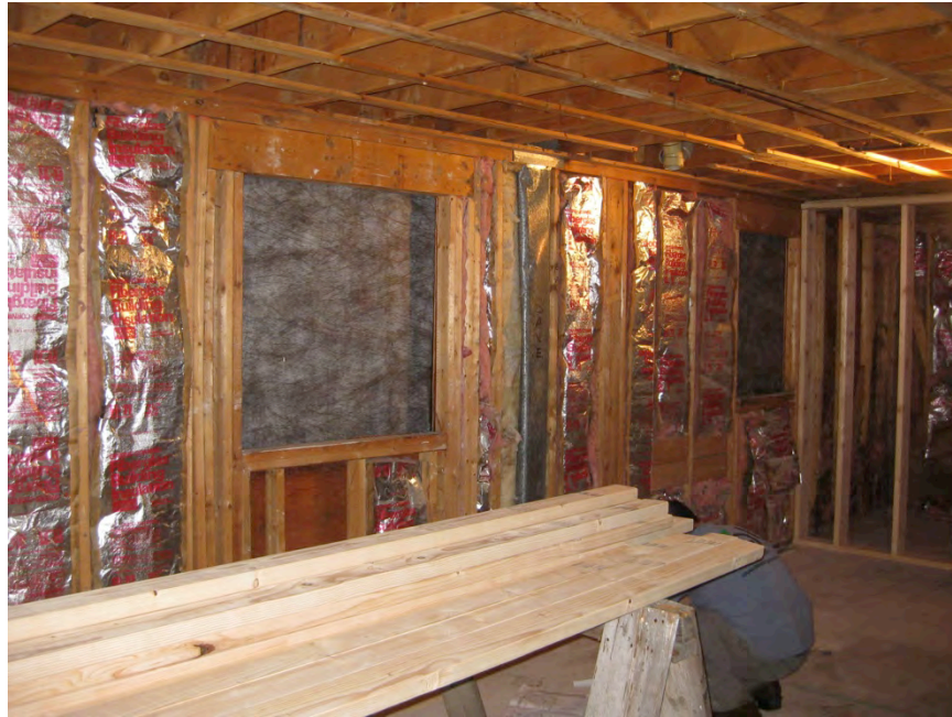
Figure 42. Foil-faced cavity insulation representing a second vapor retarder, Test Home 1
