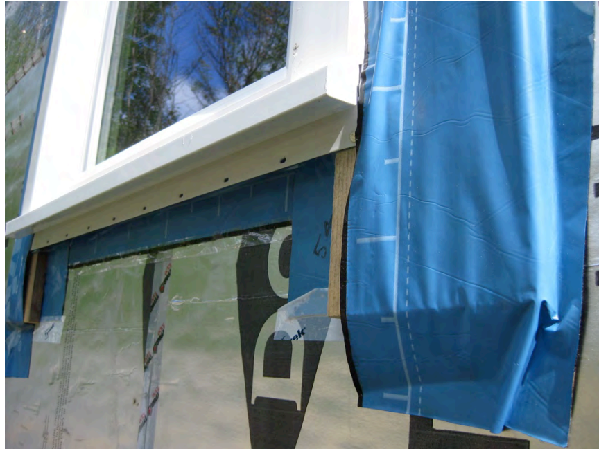
Figure 50. Installation of the window over strapping provides a generous drainage gap for the sill pan flashing.
