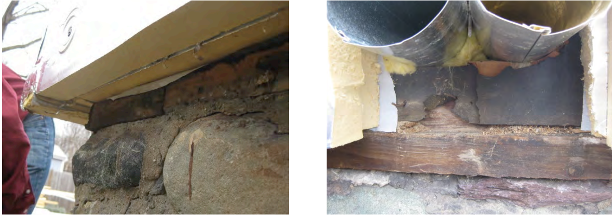
Figure 38. Left: Exterior insulation installed prior to sealing house wrap to base of wall for airflow control transition; Right: Portions of exterior insulation must be removed to allow air sealing of the house wrap at these pipe penetrations.
