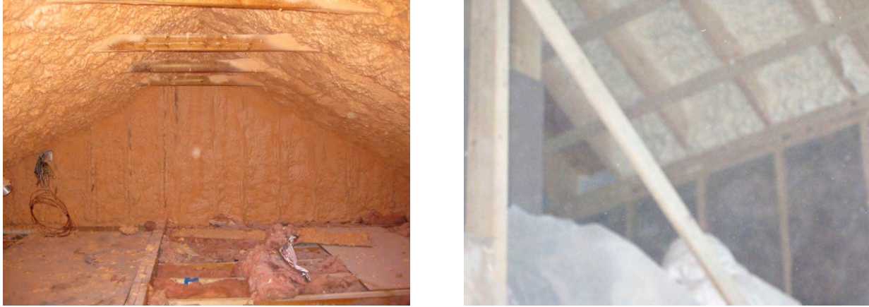
Figure 19. Left: ccSPF insulated roof at Test Home 1; Right: partial ccSPF insulation in a section of roof framing at Test Home 3. Note that Test Home 1 remained unoccupied except for active construction for a period of several months after application of ccSPF. During active construction, doors and windows remained open. During the period after application of ccSPF in Test Home 3, the application floor and floor below were active construction zones with doors and windows typically open during daytime hours.
