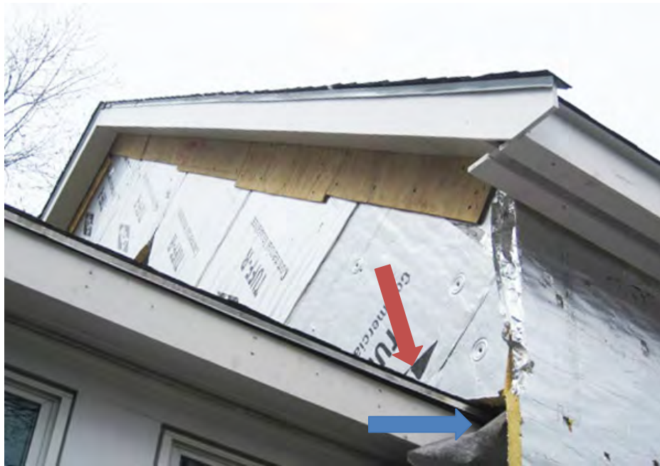
Figure 35. Wall-roof interface at Test Home 4 showing two common flashing errors: 1) step flashing is not located at plane of water control, and 2) drip edge of lower roof creates a condition where water may be directed in behind the drainage plane. Note that both of these conditions were corrected at this test home.
