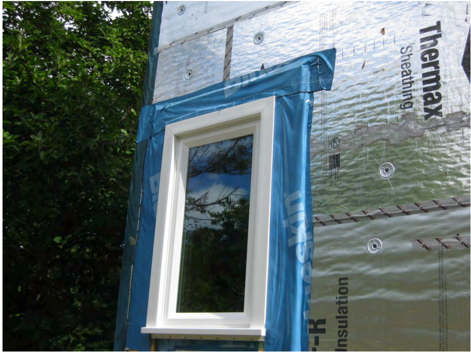
Figure 36. Nonterminated flashing membrane presents risk of collecting water
