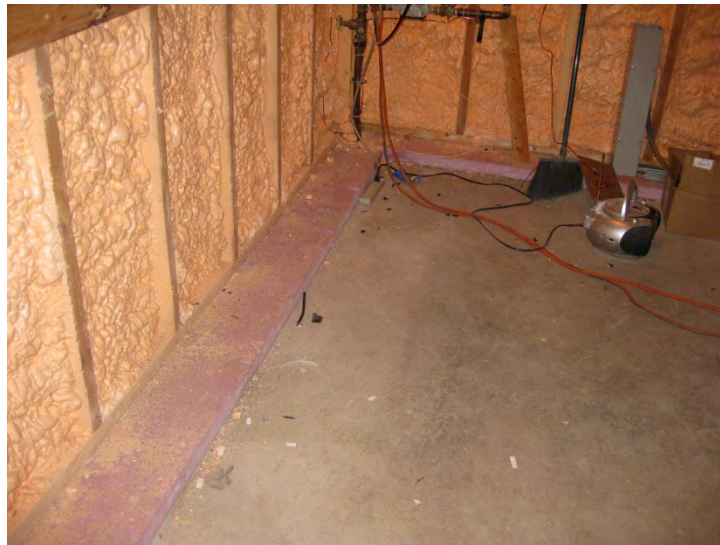
Figure 54. Thermal break between wood stud wall and existing concrete slab at Test Home 1
