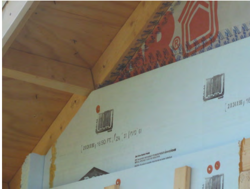
Figure 32. Example of airflow control transition at gable end of vented attic. The house wrap is taped to the wall sheathing at the level of the attic floor. Note that it is not necessary to tape the house wrap above this level.
