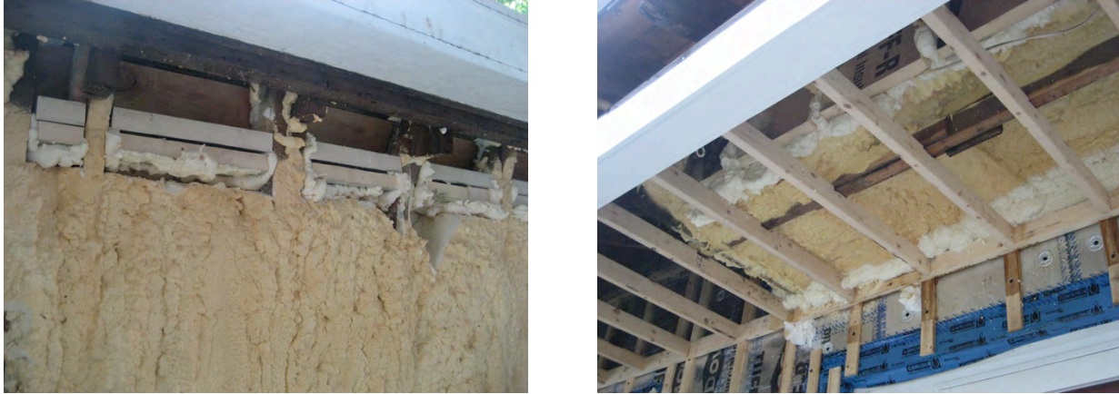
Figure 10. Left: Initial two-part ccSPF application to connect wall insulation to previous work; Right: subsequent two-part ccSPF providing more robust connection.
