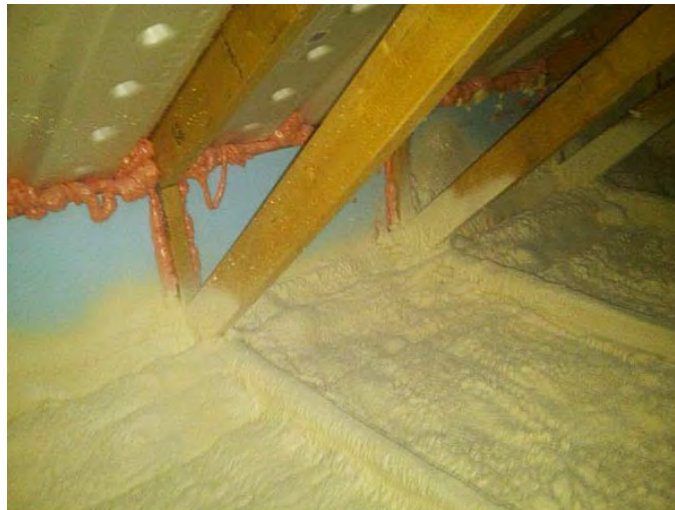
Figure 29. ccSPF airflow control layer in vented attic at Test Home 5
