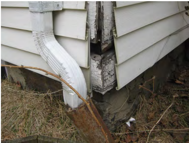
Figure 65. Vinyl siding and deteriorated wood cladding at Test Home 2
