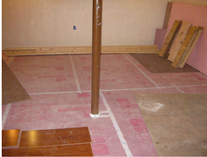
Figure 56. Basement floor insulation at Test Home 1 installed near end of project to prevent damage to insulation
