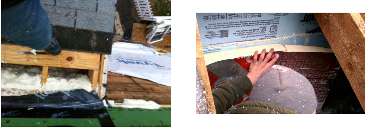
Figure 40. Left: ccSPF airflow control around porch roof framing at Test Home 3; Right: Worker applying rigid foam and foam sealant between attached porch roof and porch ceiling, Test Home 4
