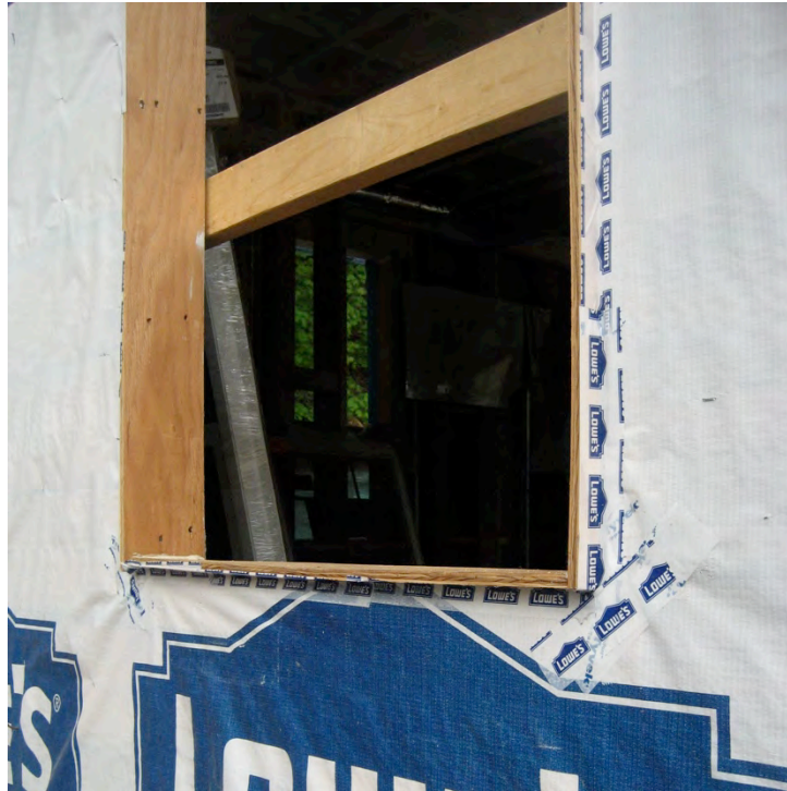
Figure 43. House wrap airflow control layer sealed to window extension box at Test Home 5
