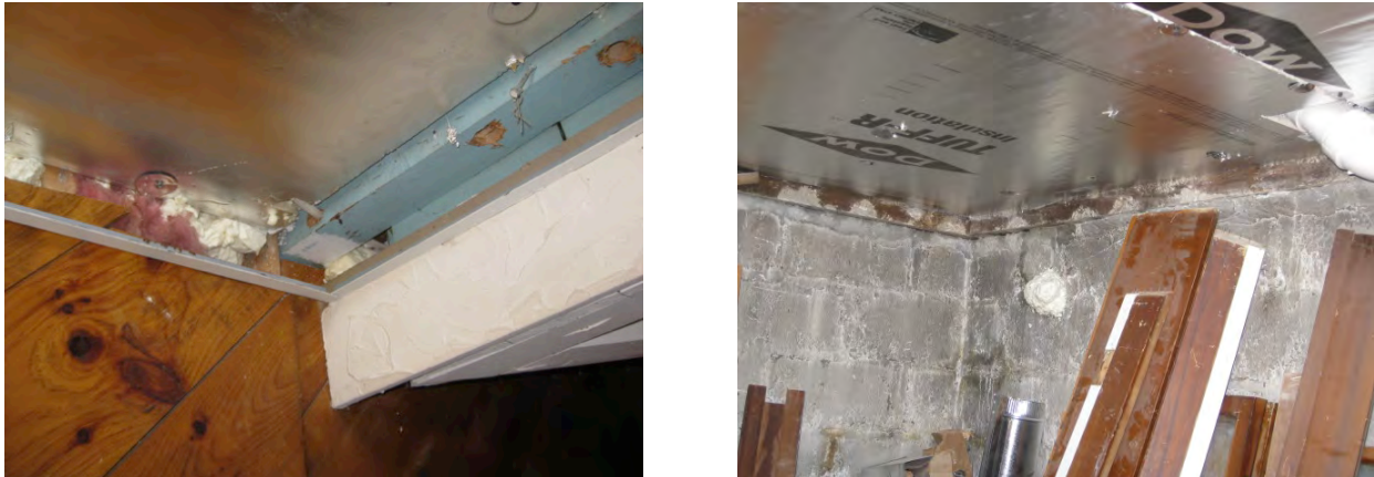
Figure 55. Left: Structural beam exposed to basement; Right: Framed wall sill exposed to basement
