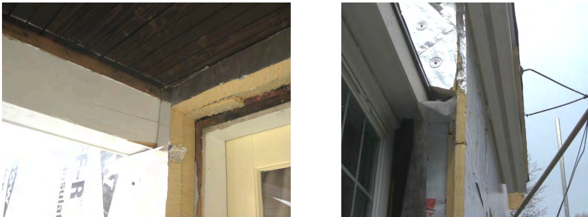
Figure 39. Left: Porch roof support beam with trim and porch ceiling void airflow control where they connect to the wall and penetrate exterior insulation; Right: A porch roof return that connects to the existing wall challenges continuity of airflow control.
