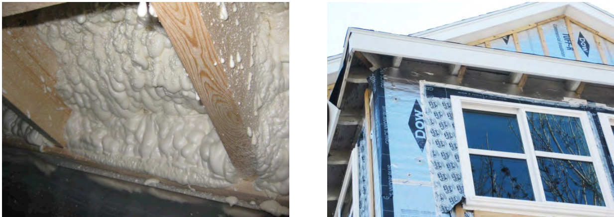
Figure 14. Left: ccSPF providing transition of airflow control at new roof to new wall transition; Right: Rigid exterior insulation notched around projecting rafters.
