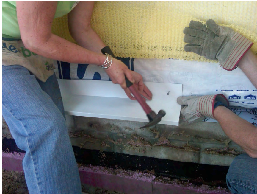
Figure 45. Brake-formed metal protection for exterior foam insulation at Test Home 5
