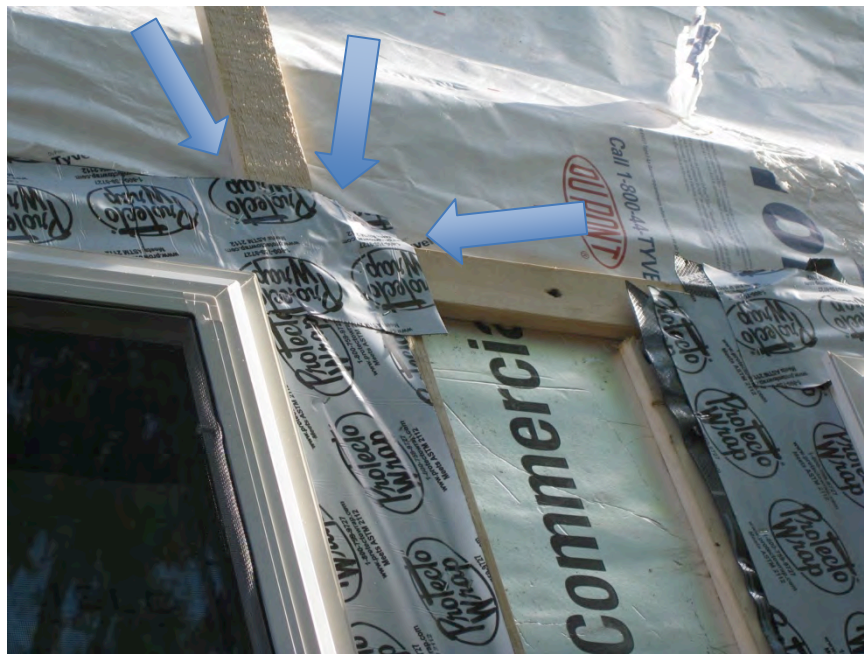
Figure 48. Scoop flashing at head of window installed over strapping at Test Home 3. Arrows indicate where water would be able to pass behind the flashing.
