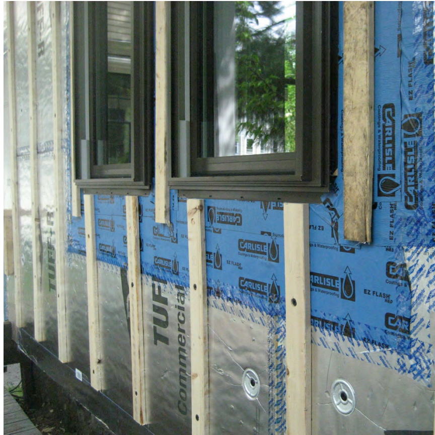
Figure 51. Window installed with flanges aligned with drainage plane at Test Home 2. Note strapping run up to, but not over, bottom flange of window. A single piece of strapping at the side of the window is sufficient to support both trim and cladding attachment.
