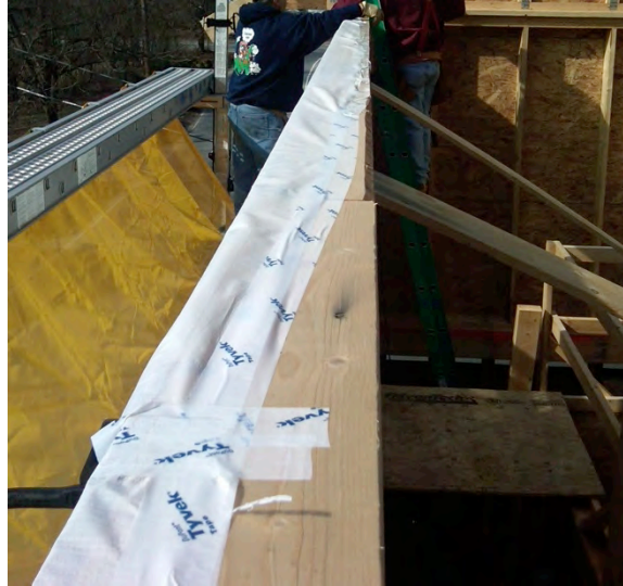
Figure 31. House wrap airflow control transition at top of wall at Test Home 5
