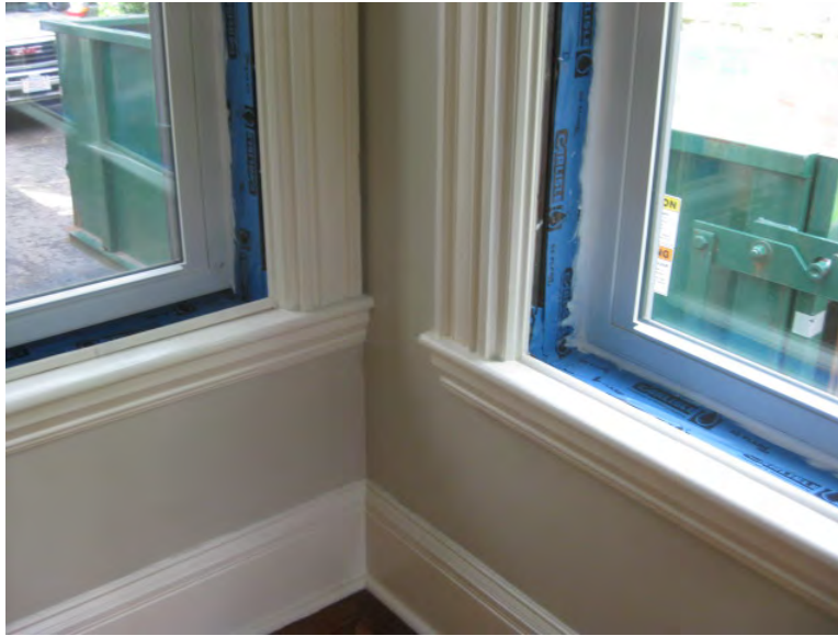
Figure 52. Window sealed to membrane at inside perimeter of window at Test Home 2. Note how the window frame is slightly larger than the finished opening.
