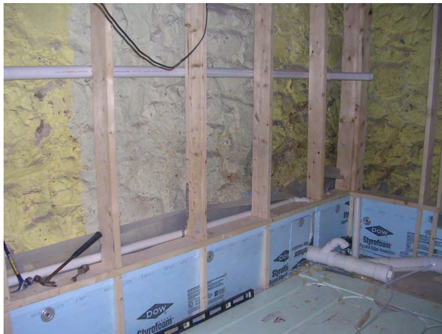
Figure 53. Thermal break between wood stud wall and concrete underpinning wall at Test Home 4
