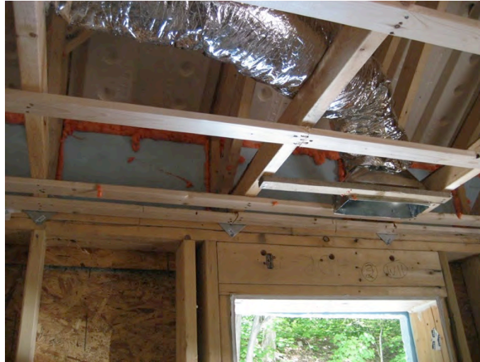
Figure 30. Ventilation duct initially located above airflow control layer in vented attic at Test Home 5
