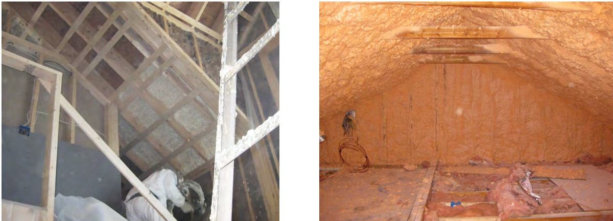
Figure 24. Left: SPF insulation being installed in roof framing cavities at Test Home 3. Note how roof framing precludes insulation for an appreciable portion of the roof area and that the strapping depth does not allow much depth for insulation over the framing; Right: roof rafters fully embedded in spray foam insulation at Test Home 1.
