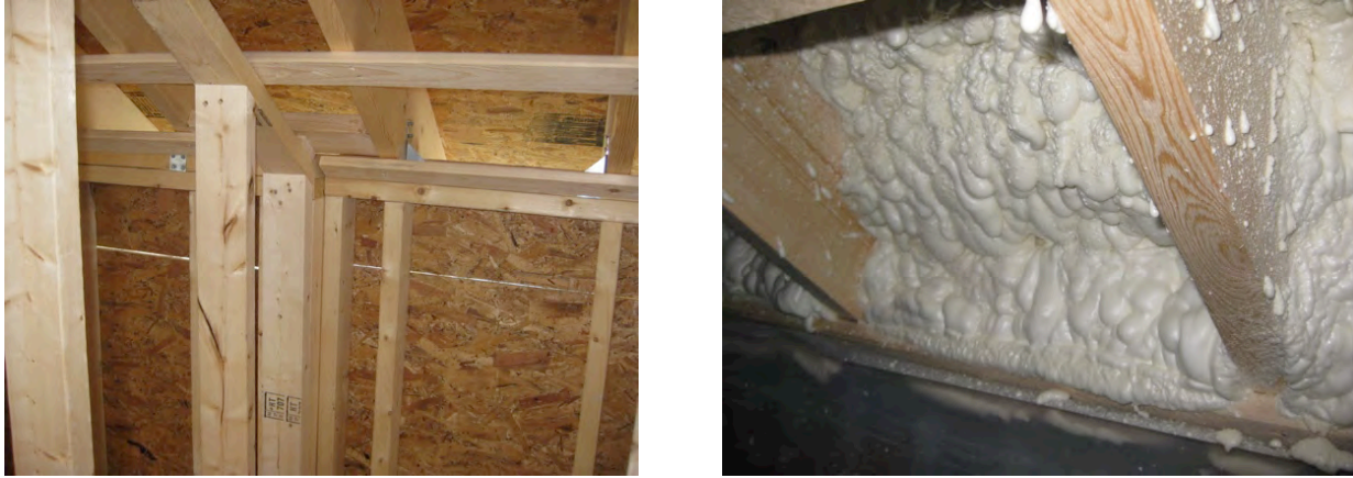
Figure 22. Left: Rafter bay continuous to soffit area at Test Home 3; Right: SPF insulation in rafter bay connecting to top of wall at Test Home 3
