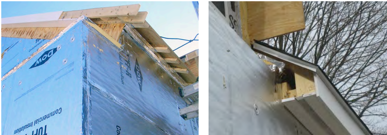
Figure 28. Left: Plywood gable rake support at Test Home 4. Right: fascia and soffit of main roof framed over insulation layers and attached to 2 × 4 purlins.
