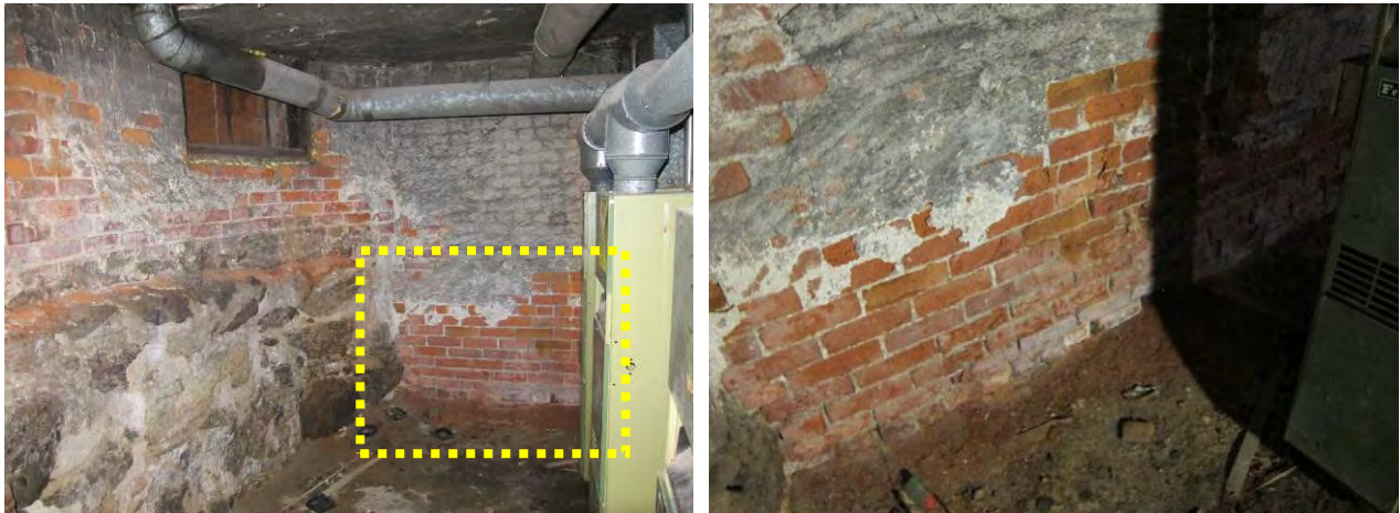
Figure 17. Capillary rise on south party wall (near furnaces). Left image shows front of building.
