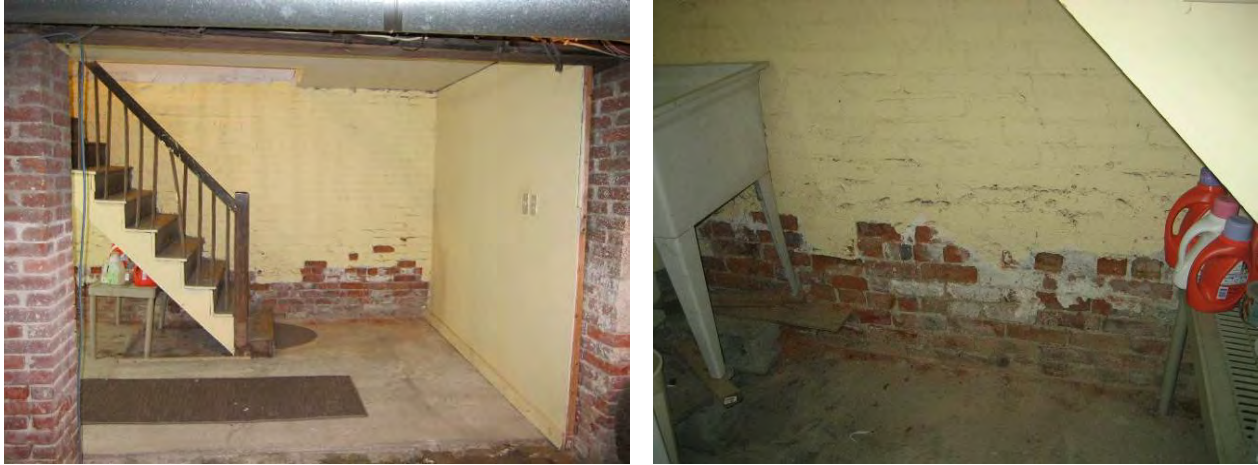
Figure 16. Evidence of capillary rise on north party wall (laundry area)
