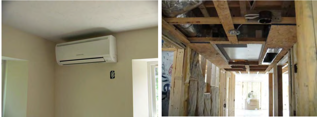
Figure 41. Mini-split wall-mounted unit (left) and recessed compact air handler (right)
