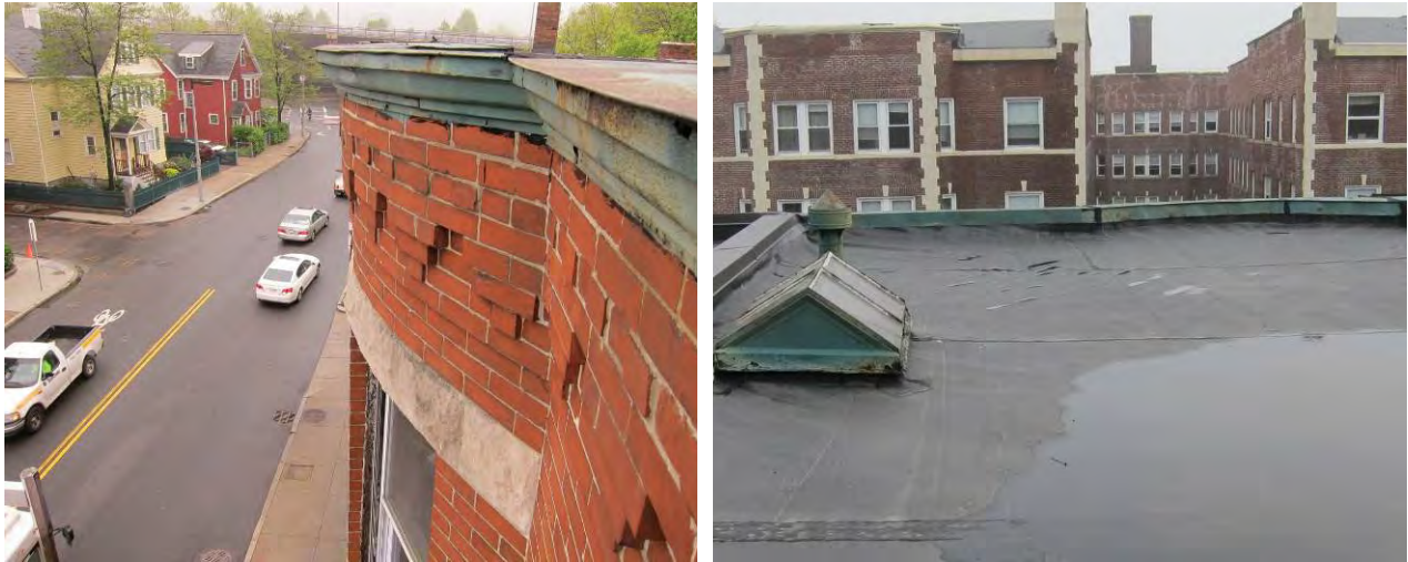
Figure 8. Front parapet brick condition (left) and interior side of parapet showing height (right)
