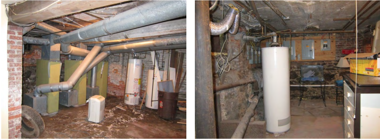
Figure 29. Gas furnaces (left) and DHW tanks (right)
