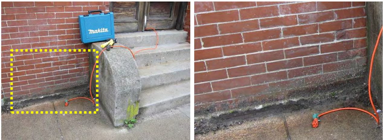
Figure 9. Brick condition adjacent to front steps (left) and evidence of splashback (right)
