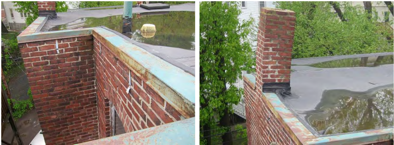
Figure 15. Brick condition at parapet near light well (left), and chimney condition (right)
