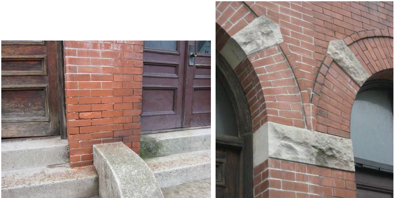
Figure 11. Freeze-thaw damage at front party wall (left) and doorway arch details above (right)
