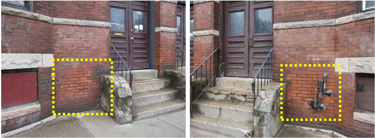
Figure 12. Freeze-thaw damage and mortar erosion next to front steps at two adjacent buildings
