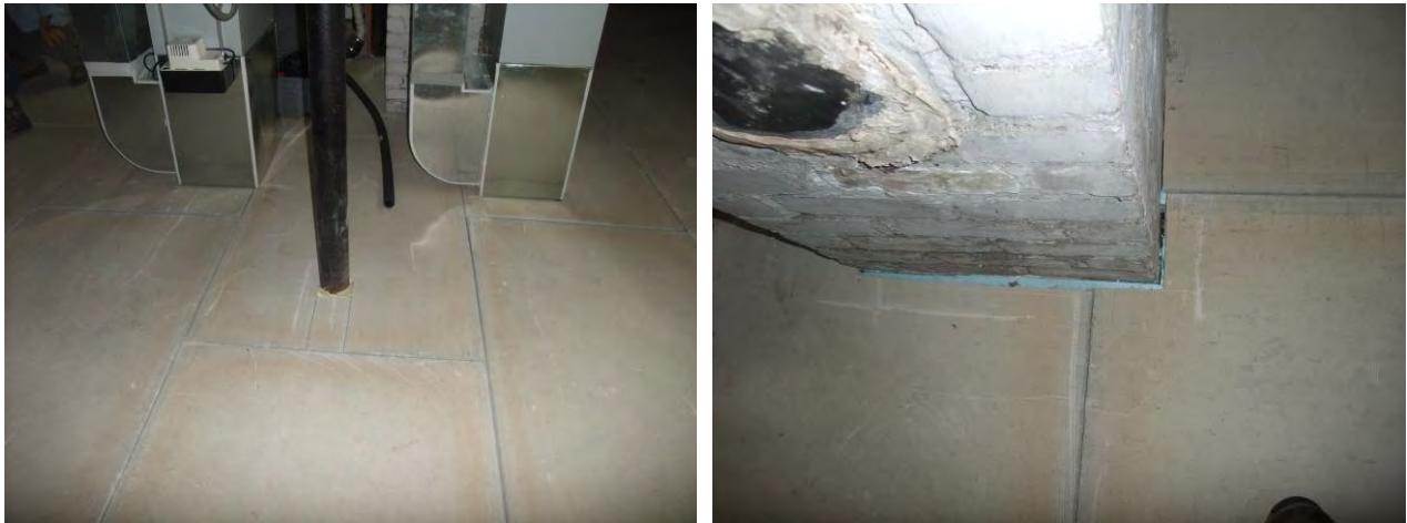
Figure 38. Storage use basement slab insulation/moisture control retrofit (left); cement board surface (right)
