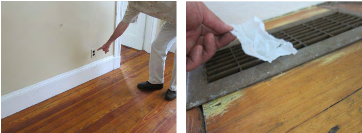
Figure 27. Air leakage was evident at electrical receptacles and ductwork registers
