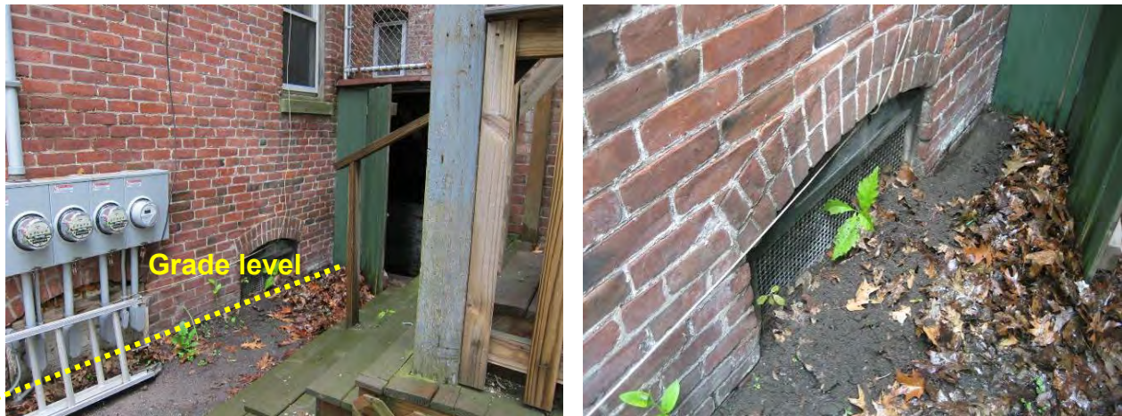
Figure 19. Rear wall near subfluorescence damage visible in basement
