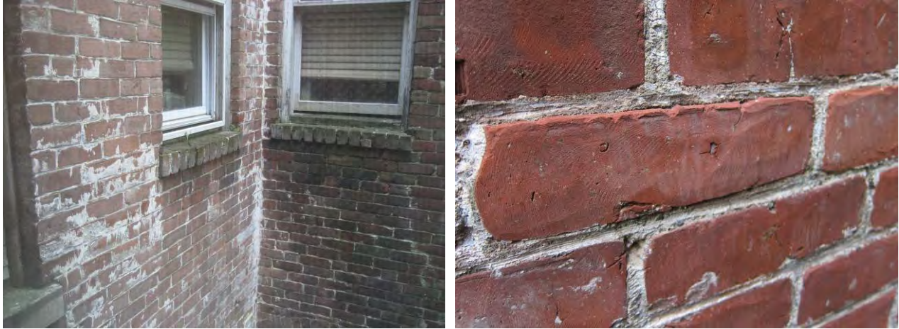
Figure 14. Residual paint at rear of building (left) and scarification of brick due to abrasive cleaning (right)
