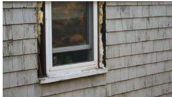
Figure 18. Abandoned sash weight and insulation installation
