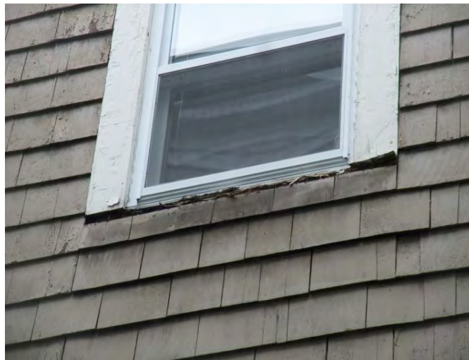
Figure 5. Failed window sill with replacement window installed
