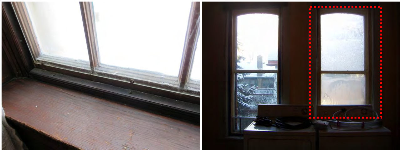
Figure 19. Examples of condensation problems with interior storm window retrofits
