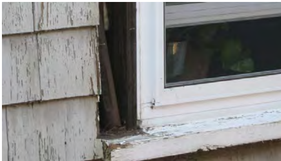
Figure 17. Sash weight pockets
