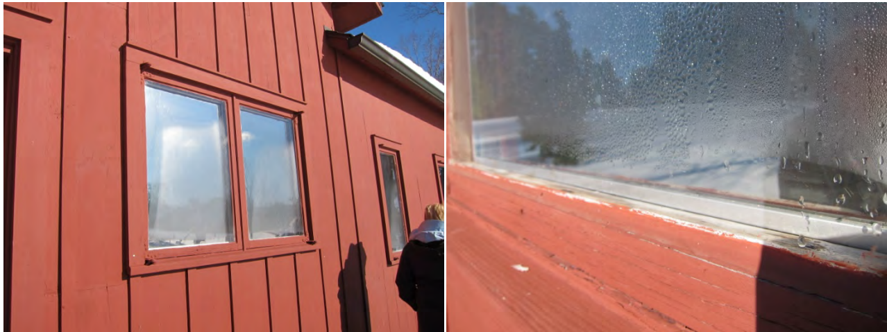
Figure 20. Examples of condensation problems with interior storm window retrofits
