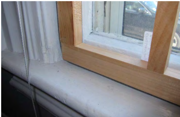
Figure 26. Installed interior removable storm window
