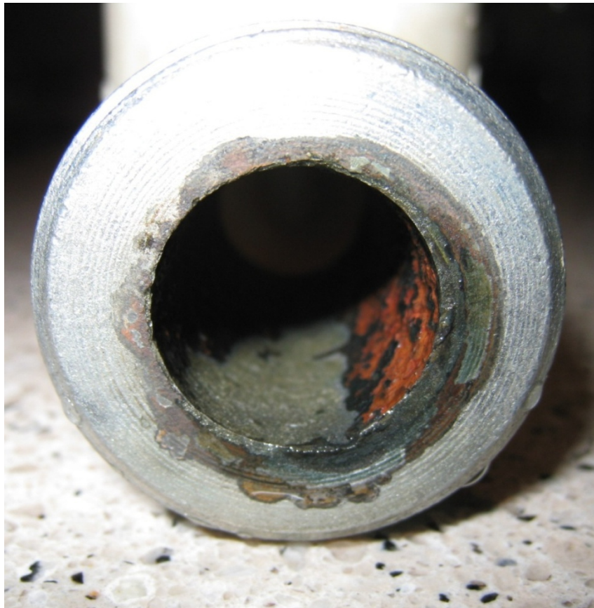
Figure 12(b). Scale being removed from a galvanized dielectric union fitting weeks after installation of an electronic water conditioner; the electronic water conditioner apparently loosens calcium carbonate particles and makes them electro-chemically less “sticky” so that they flow through the system
