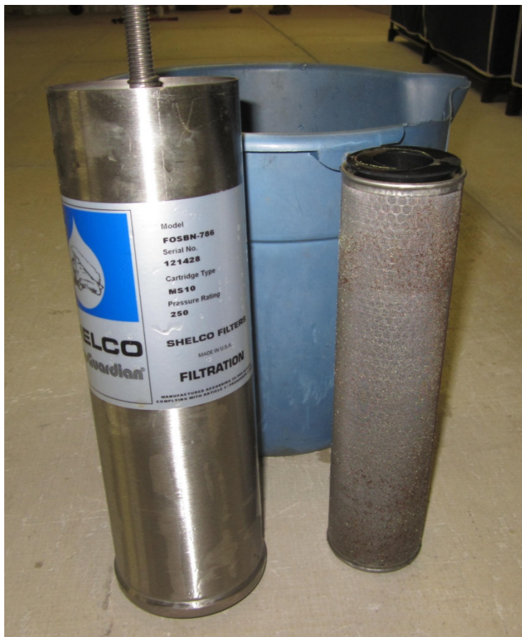
Figure 11. Large pre-strainer installed to extend the water heater inlet strainer service interval to annual cleaning at most
