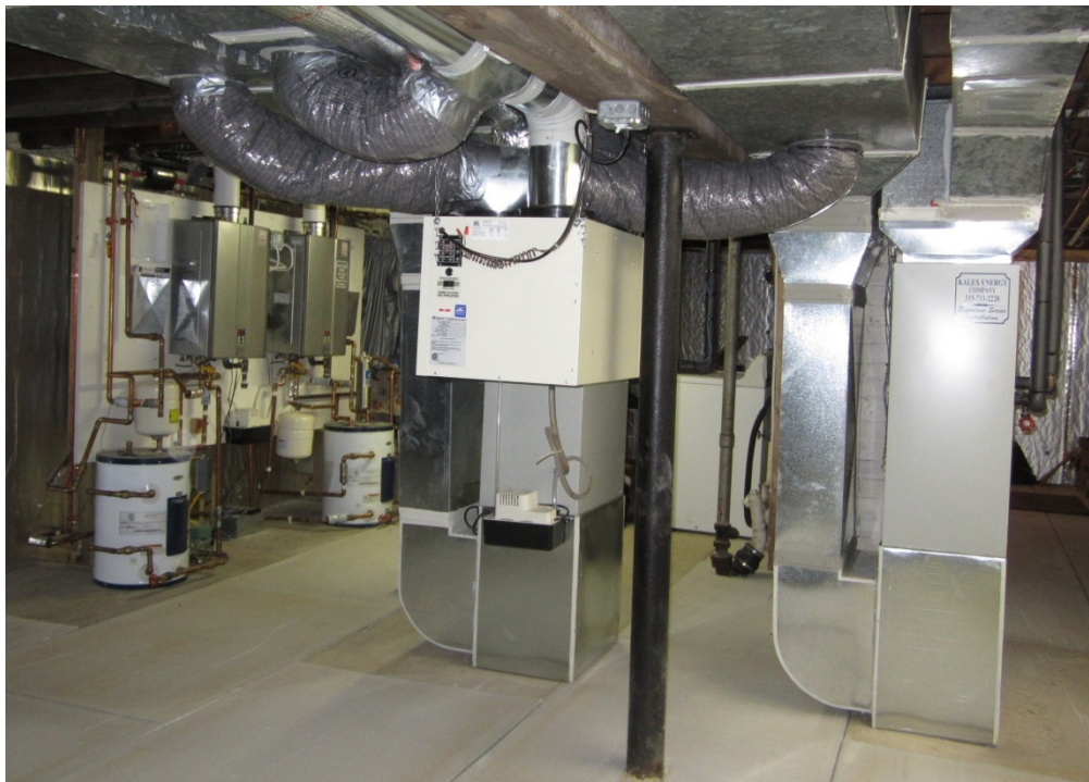
Figure 1. Photo of two installed combination space and domestic water heating systems with a condensing TWH and small storage tank
