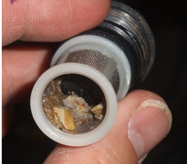
Figure 10(c). Strainer-clogging debris that broke loose within the existing water pipes; new water heater supply pipes should be used when possible
