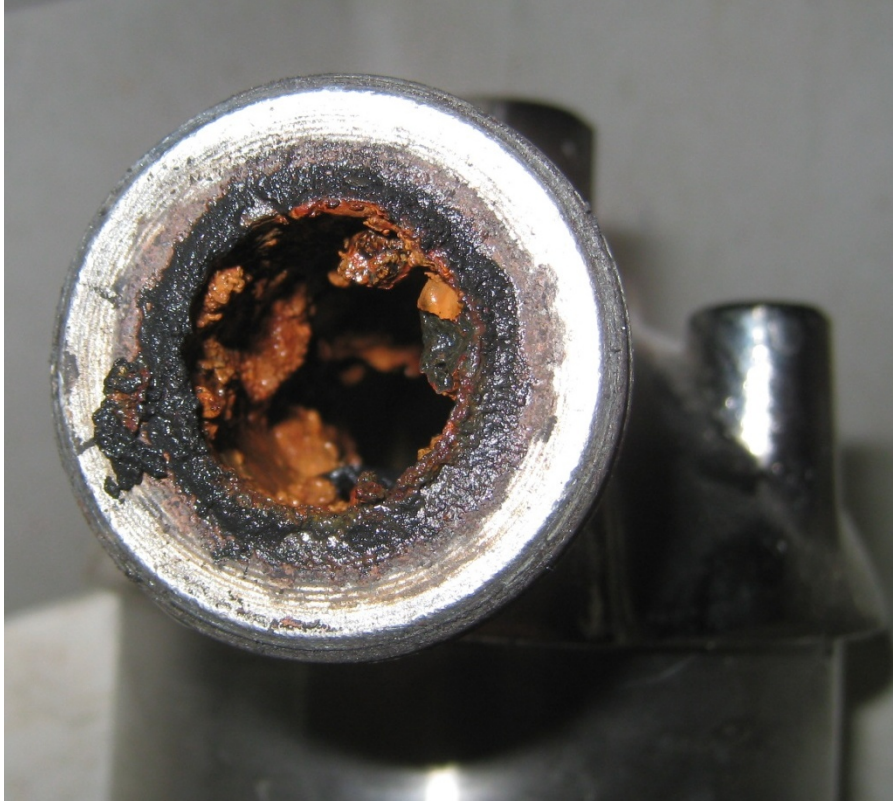
Figure 12(a). Scale forming in a galvanized dielectric union fitting; all galvanized fittings should be plastic lined to reduce scale buildup
