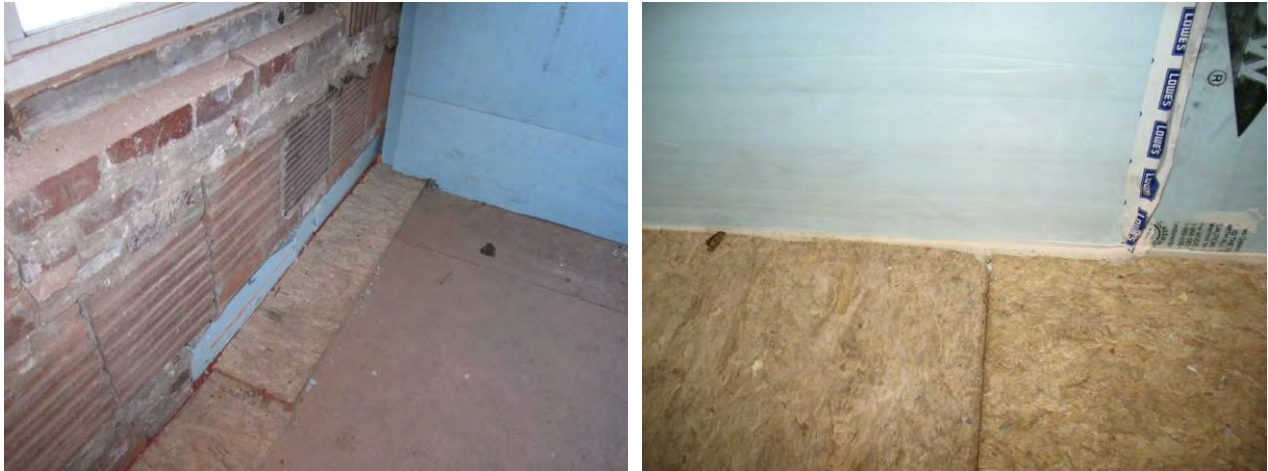
Figure 45: Floor edge detail, showing added floor sheathing (left) and air seal between foam and floor (right)
