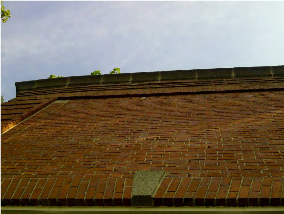
Figure 20: Bricks and belt course pushing out on north façade
