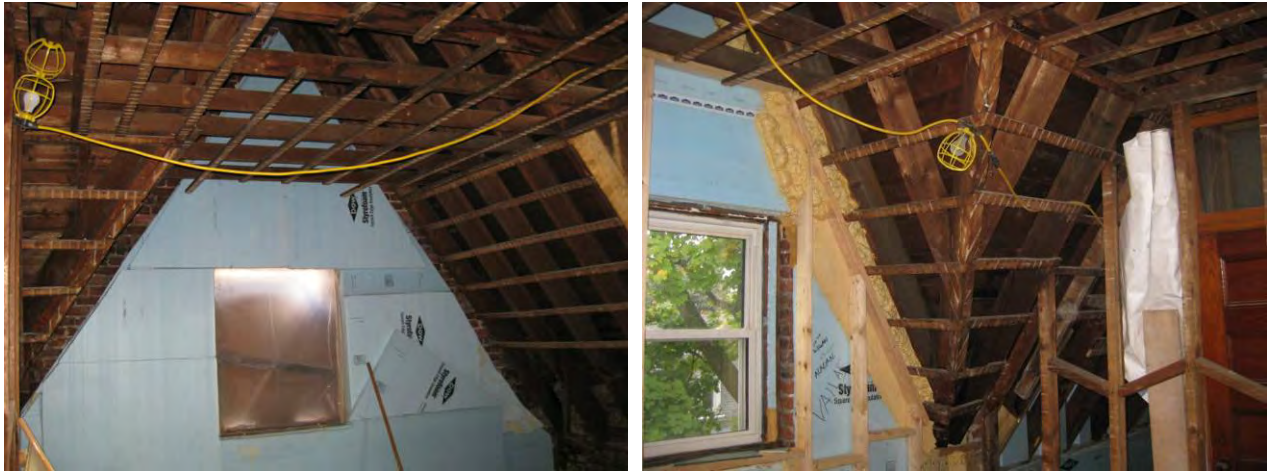
Figure 34: Rigid wall insulation left clear of roof (left) and infill with spray foam kit (right)
