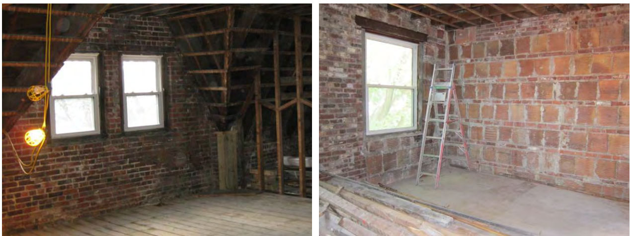
Figure 22: Exterior wall conditions at solid brick (left) and hollow clay block infill (right) conditions
