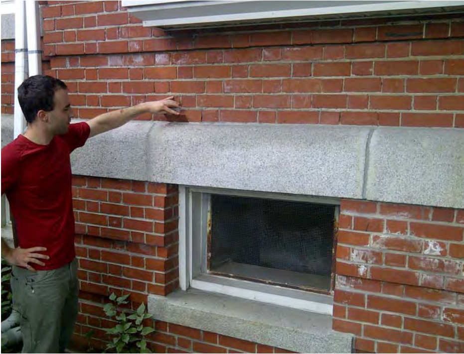
Figure 7: Original building: brickwork spalling and surface efflorescence
