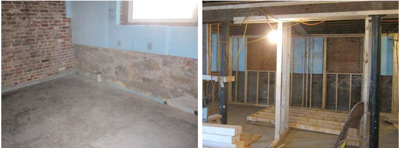
Figure 40: Edge detail after casting of slab (left) and installation of interior framing (right)
