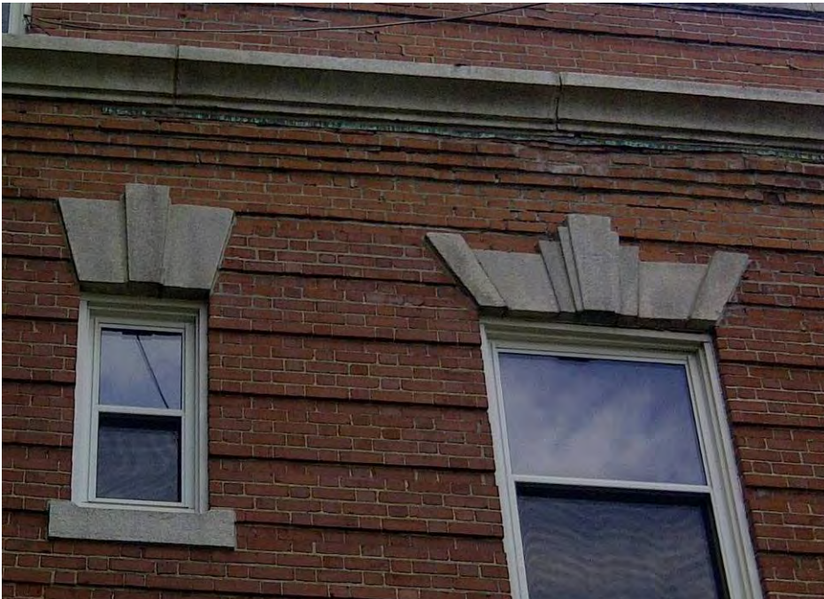
Figure 8: Original building: brickwork and mortar damage below belt course
