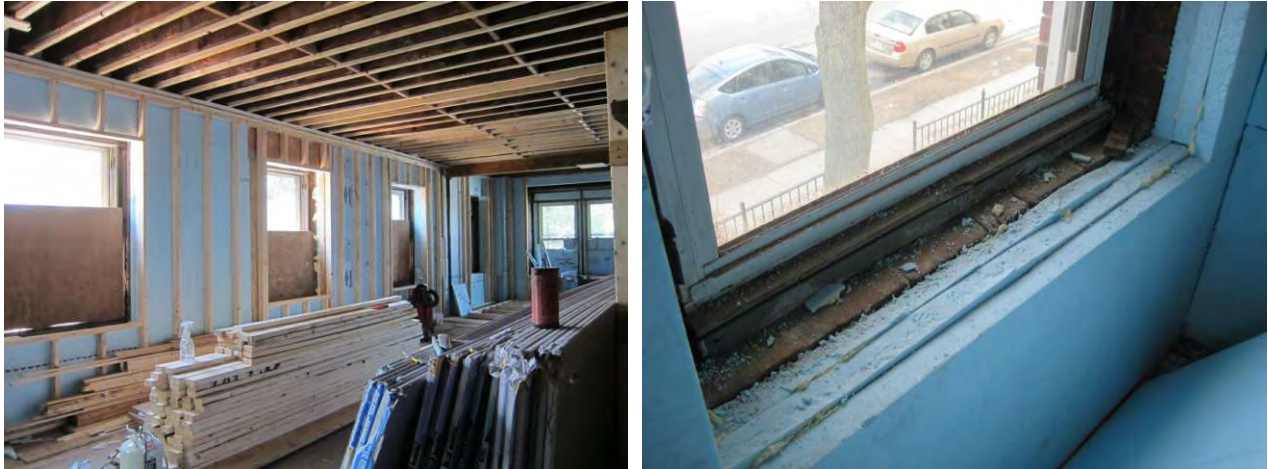
Figure 26: Framing installed inboard of insulation (left) and conditions at window opening (right)
