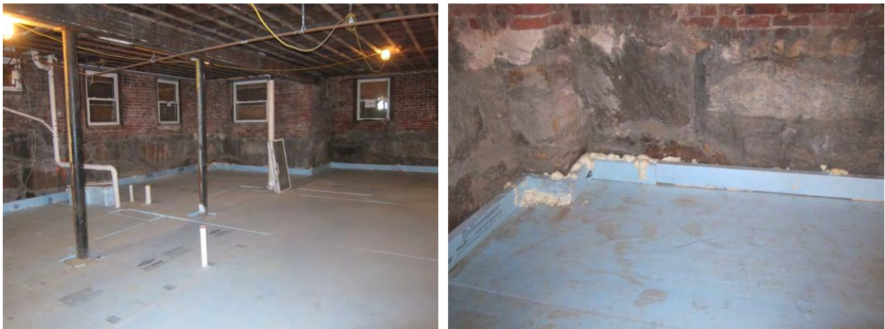
Figure 39: Installed sub-slab insulation at basement (left) with detail of slab edge insulation (right)
