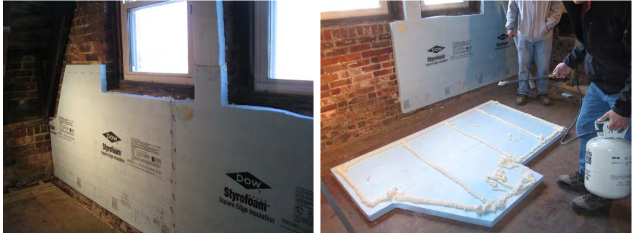
Figure 24: Test installation of foam on masonry (left) and use of polyurethane adhesive (right)
