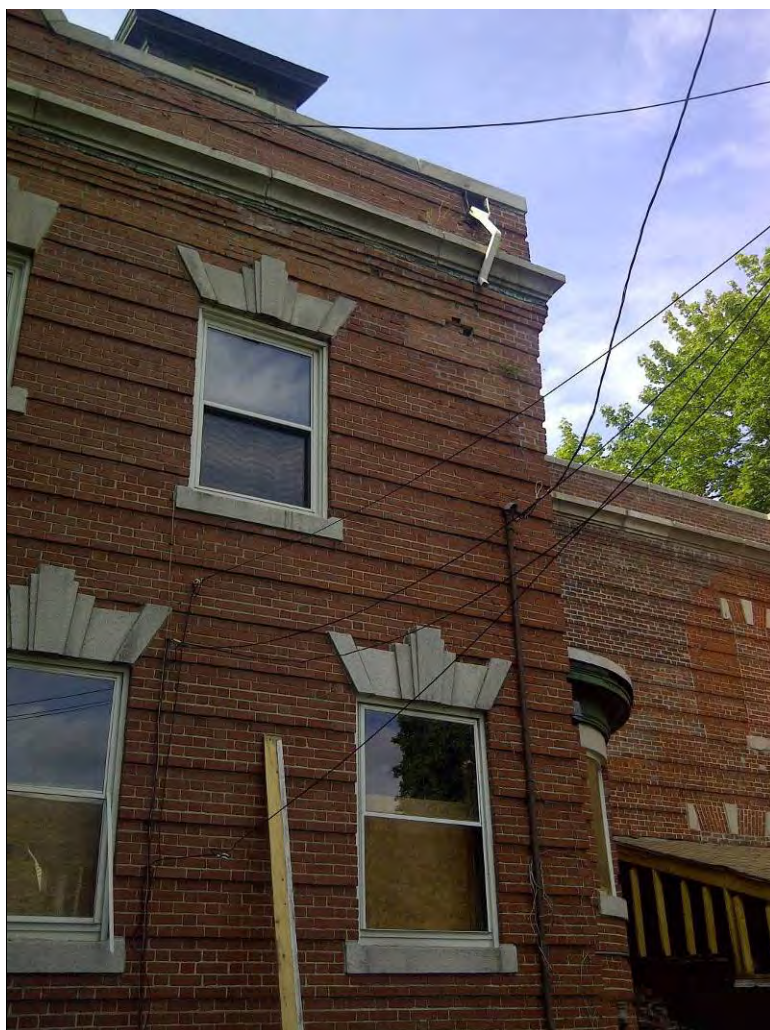
Figure 9: Original building – missing downspout
