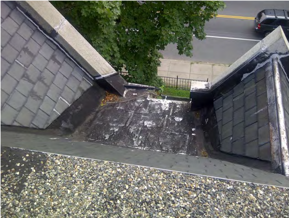
Figure 12: Roof drain filled with debris
