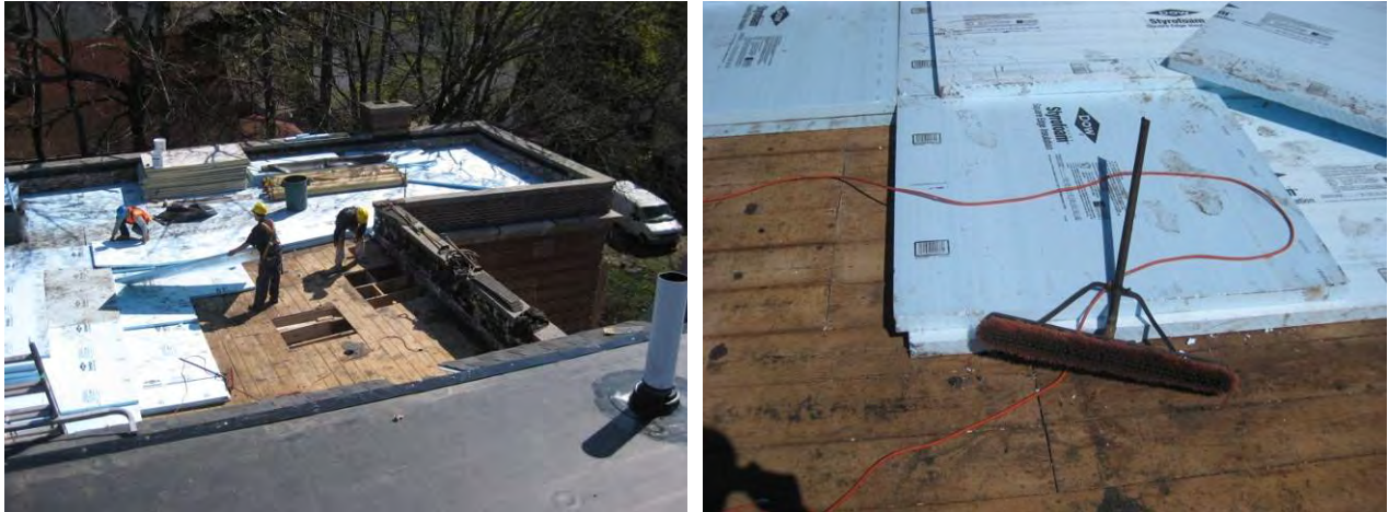
Figure 30: Insulation of lower roof, showing lack of air barrier at board sheathing
