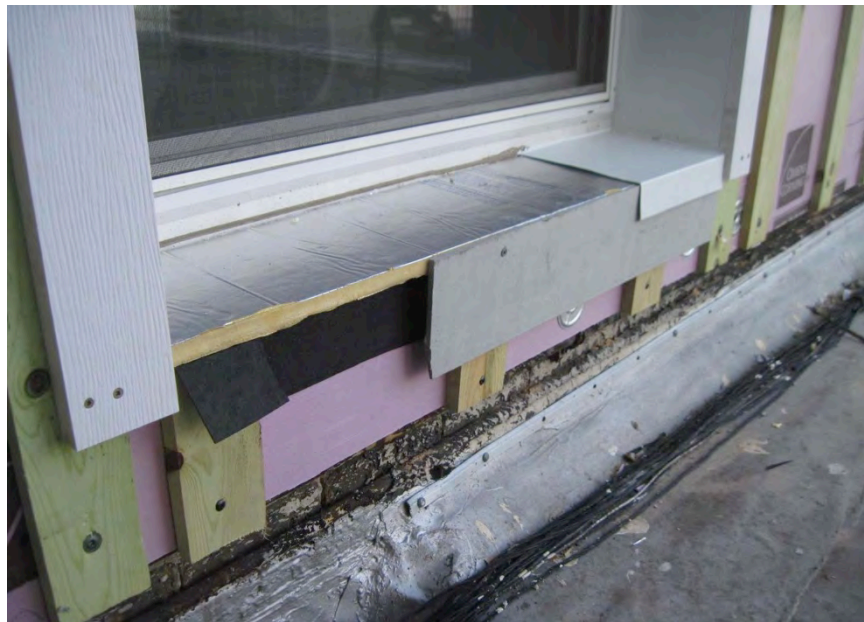
Figure 41. Second mockup of window surround showing the flashing membrane placed beneath the insulation return (Credit: Scott Sanders, CEDA)
