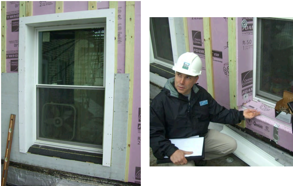
Figure 39. (L) Contractor mockup of window surround; (R) BSC personnel explaining placement of flashing membrane (Credit: John Yi, CEDA)
