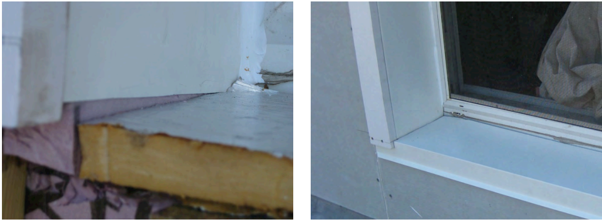
Figure 42. (L) Insulation return at the jamb installed before the insulation return at the sill. Note also that the sill flashing membrane does not extend over the outer face of the insulating sheathing. This was later corrected. (R) Sill trim installed after the jamb return trim. Sill extensions are actually cut around the jamb trim. Note that the window sill trim has a kick-out to direct water away from the face of the building.
