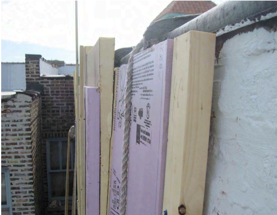
Figure 26. Beveled roof insulation used to true new cladding attachment at top of wall. Note that fasteners are left loose at the time of this photo.
