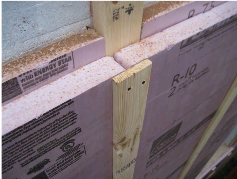
Figure 22. Offset of seams in successive layers of insulating sheathing. Offset for vertical seam is limited by the size of insulation boards and the spacing of framing. (Credit: Scott Sanders, CEDA)
