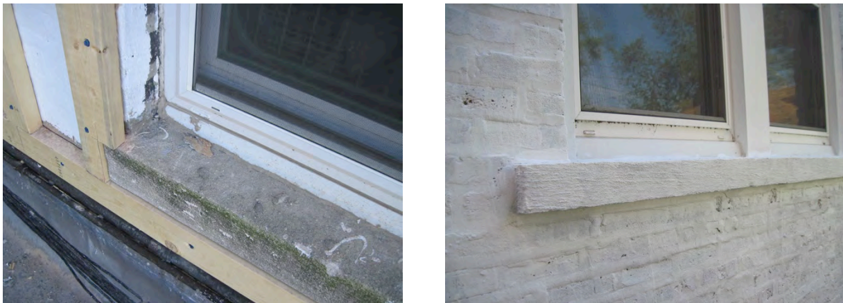
Figure 14. (L) Elastomeric paint application not complete around windows and portions of masonry surface obscured by wood framing; (R) elastomeric paint application at the two-family building covering the window sill and lapping onto the window frame (Credit: Scott Sanders, CEDA)
