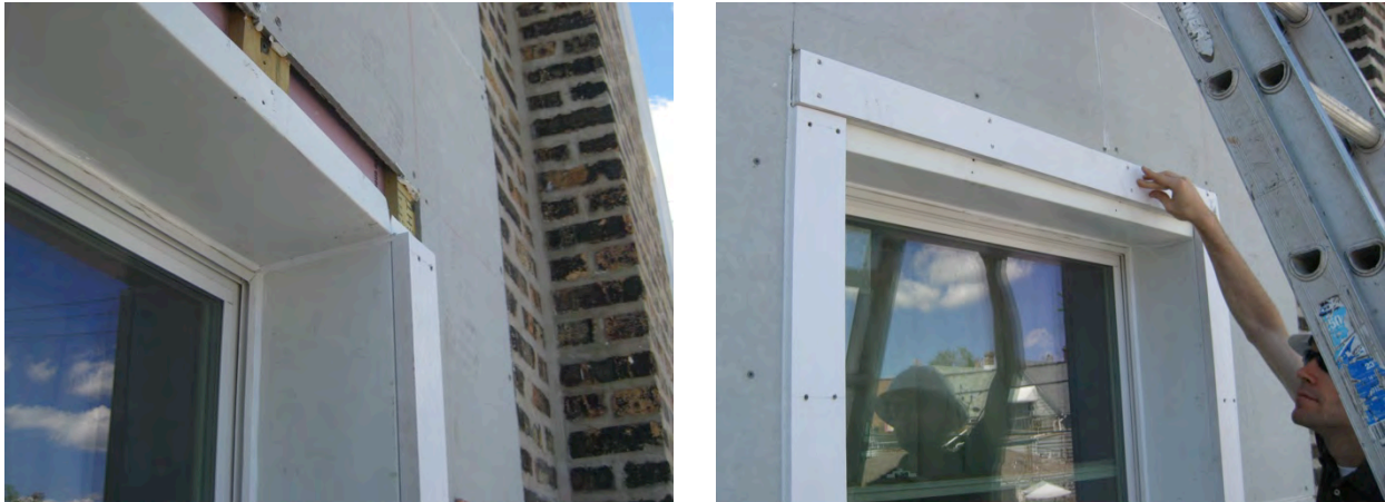
Figure 45. (L) Window head return trim sloping toward the window; (R) CEDA personnel demonstrating the reconfiguration of the window head return trim
