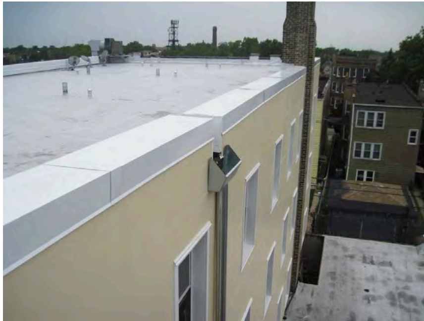
Figure 53. Visible butt joints in the finished wall
