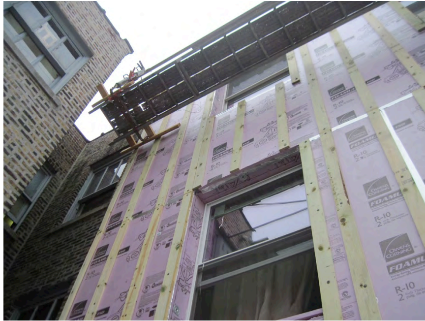
Figure 23. Wood strapping installed in vertical orientation only over face of insulating sheathing (Credit: Scott Sanders, CEDA)
