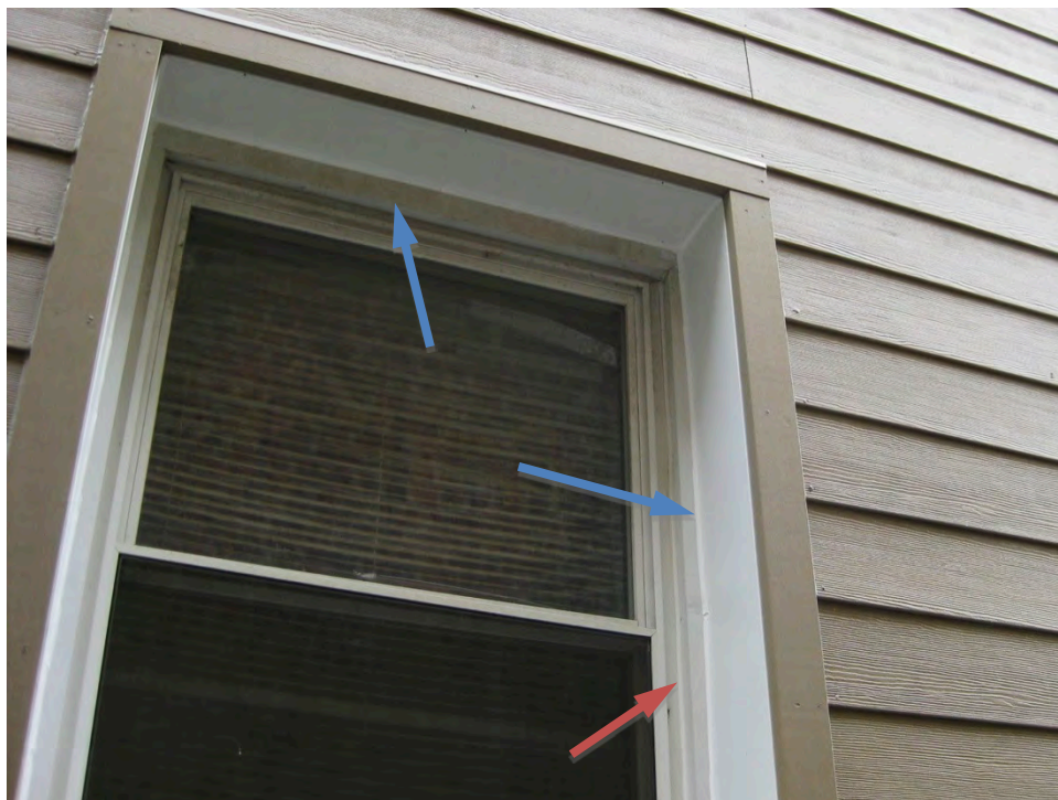
Figure 38. Return trim at the smaller building butting into the metal-clad trim surround (blue arrows) leaving the joint around the vinyl window frame exposed (red arrow)
