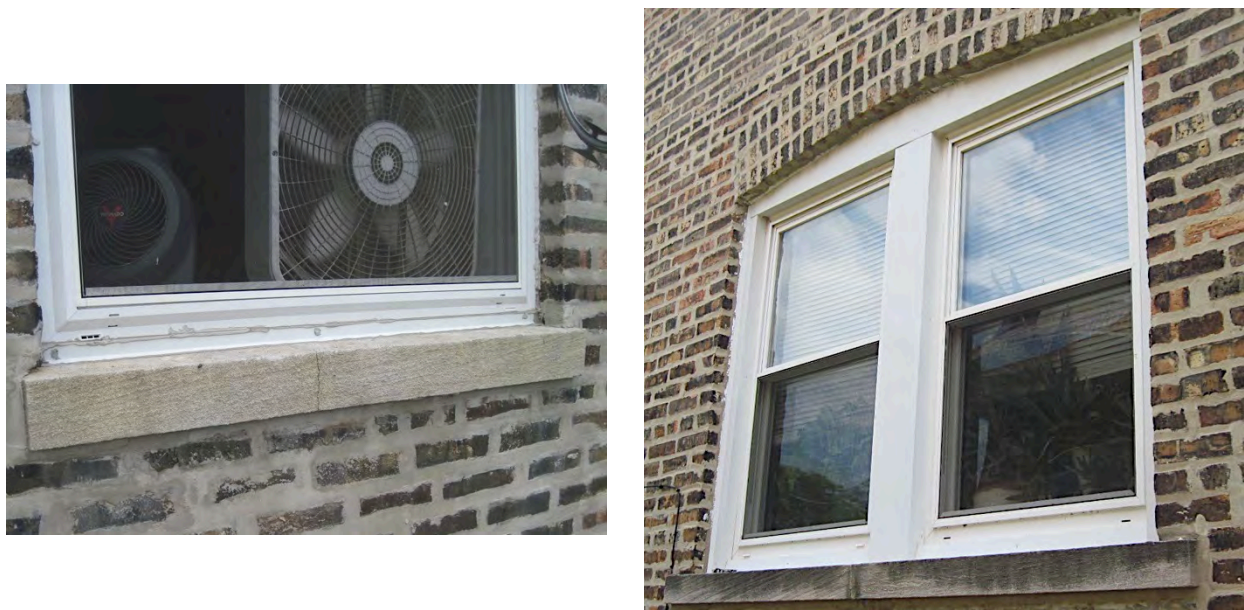
Figure 36. (L) Window set directly in masonry opening at the larger building; (R) windows set in metal-clad trim/frame surround at the two-family building (Credit: Scott Sanders, CEDA)
