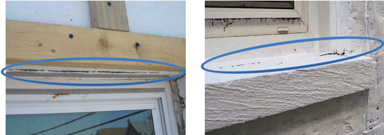
Figure 17. (L) Gap between masonry and lintel; (R) gaps at joints where sealant had not been applied as a substrate for the elastomeric paint (Credit: Scott Sanders, CEDA)
