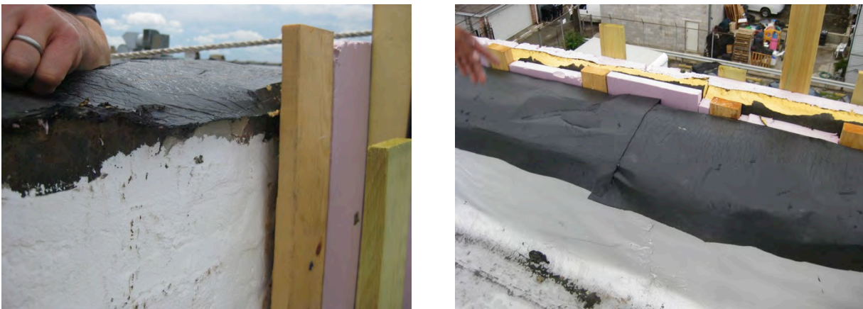
Figure 30. (L) Transition membrane not connected to elastomeric coating at face of wall; (R) transition membrane not adhered to roof membrane at inside face of parapet
