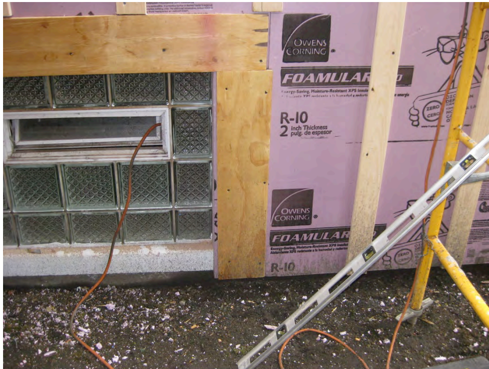
Figure 33. Base of wall insulation and over-clad assembly very close to grade at the two-family building
