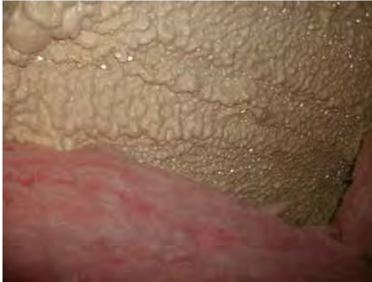
Figure 3. ccSPF unvented roof with condensation
