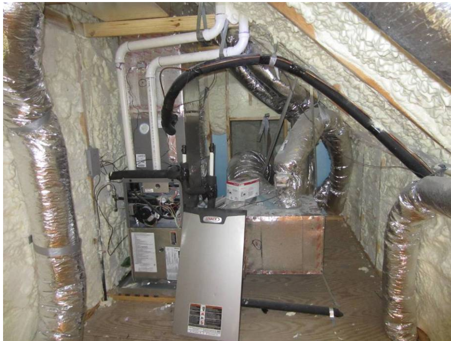
Figure 15. Plan 4127 mechanical closet in attic
