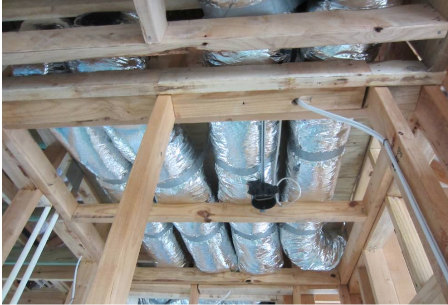
Figure 14. HVAC runouts in dropped ceiling at plan 4127
