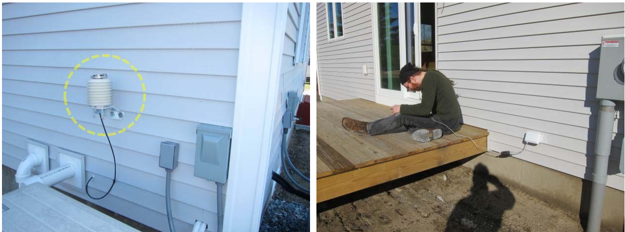
Figure 14. (L) Exterior T/RH sensor; (R) data collection from exterior connection port
