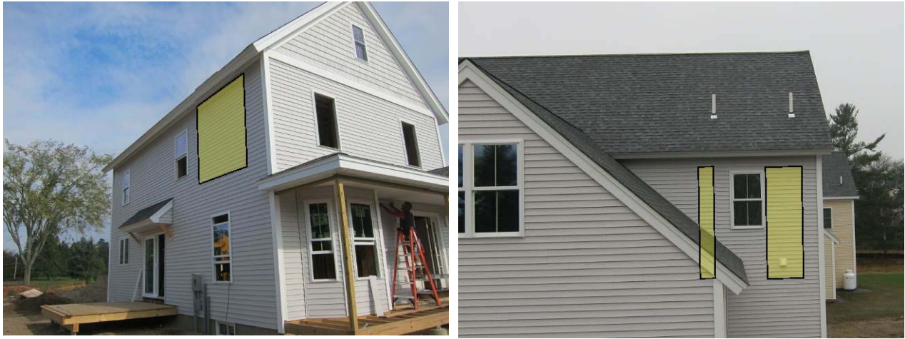
Figure 8. Test wall locations shown on exterior of house; south (L) and north (R) orientations
