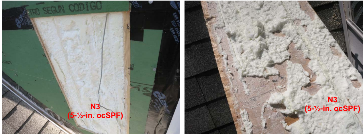
Figure 45. Stud bay cavity and sheathing conditions at 5-1/2-in. ocSPF north-facing wall (N3)
