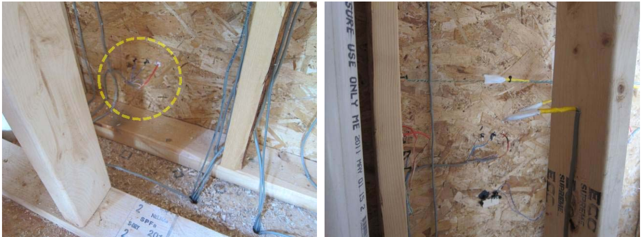
Figure 9. (L) Temperature and MC sensor at sheathing; (R) sensors at mid-height of stud bay
