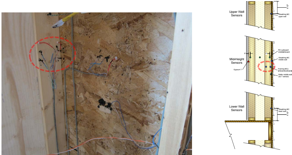
Figure 30. Framing MC/temperature sensor locations
