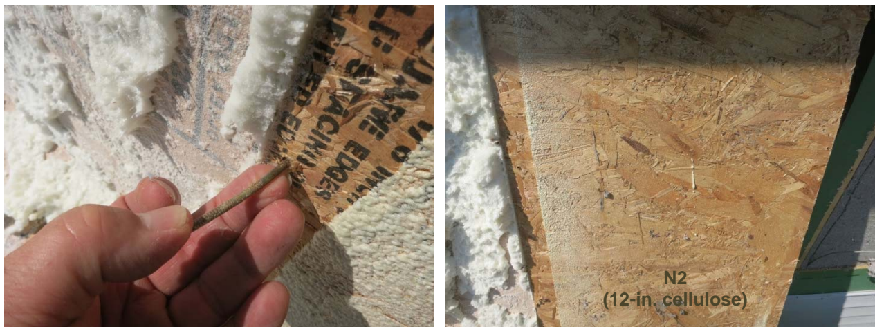
Figure 44. North-facing wall conditions at fastener and sheathing at cellulose bay (N2)
