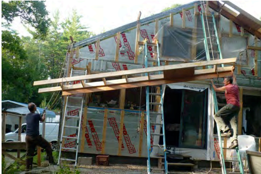
Figure 9. Pre-assembled insulated roof overhang framing being lifted into place at a gable rake for a “chainsaw” retrofit
