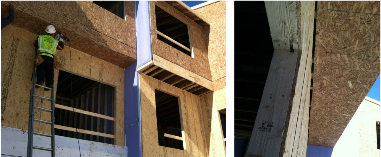
Figure 26. Overhang detail in framed building, showing gap in sheathing at inside corner
