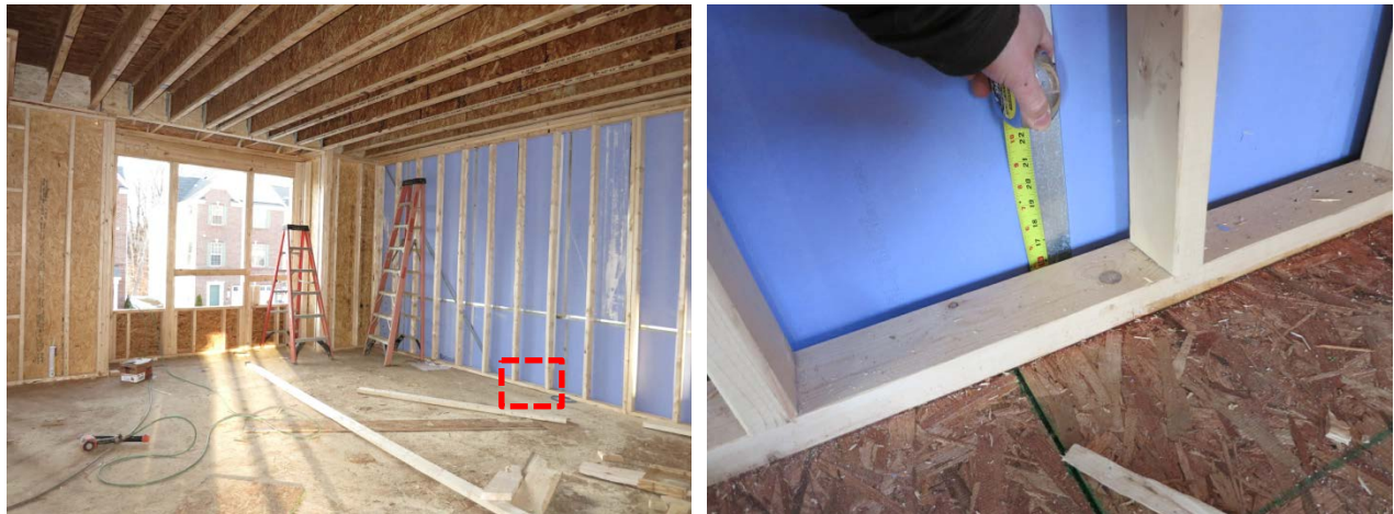
Figure 55. Missing gypsum fireblocking at garage ceiling rim joist area
