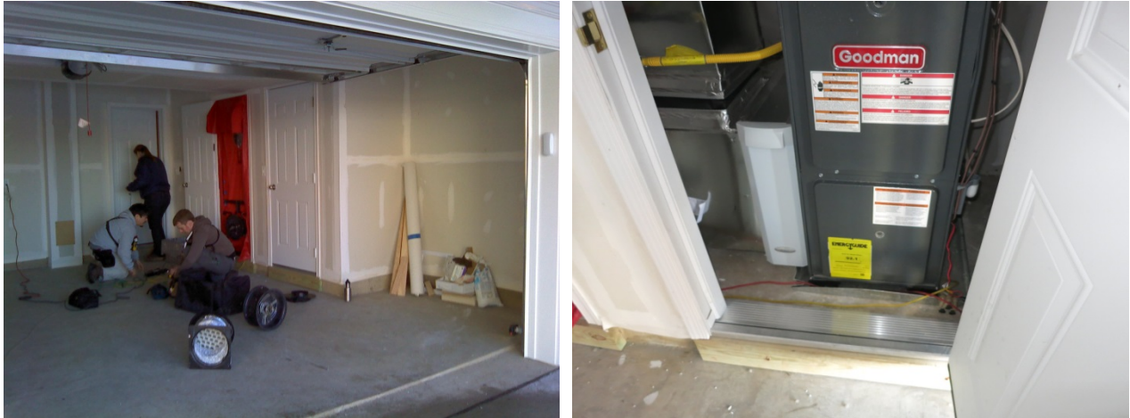
Figure 68. Mechanical room located in rear garage (Unit 6706)
