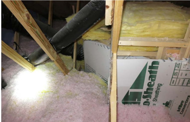
Figure 37. Attic knee wall condition and sheathing (Unit 6704)
