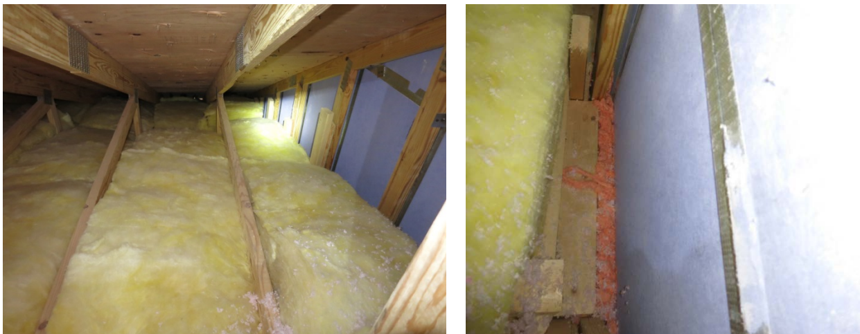
Figure 57. Vaulted attic and separation wall conditions, Unit 6704
