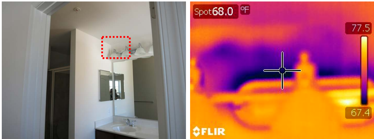
Figure 61. Air leakage at light mounted on area separation wall
